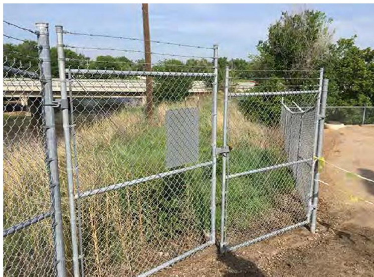
In evaluating safety improvements for the City of Greeley, our team assessed the perimeter security and identified access control deficiencies to be included in the CIP.
