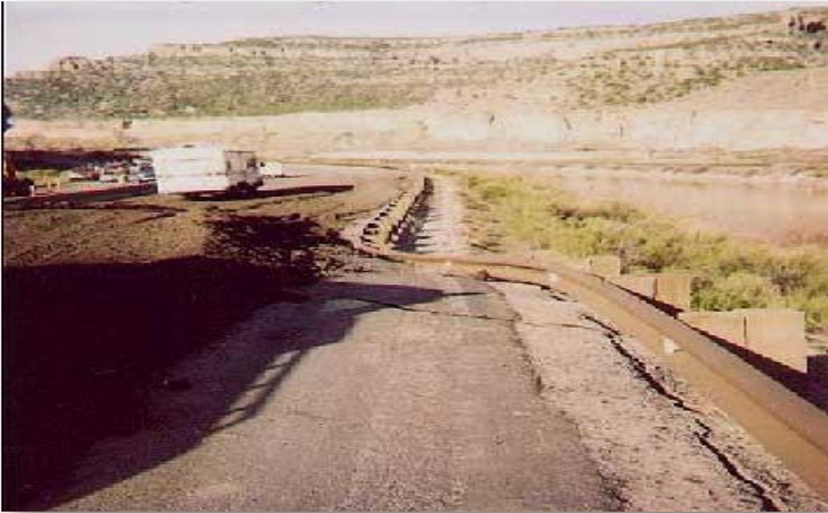
FIGURE 11 PHOTO OF DEBEQUE CANYON SLIDE AREA- INTERSTATE 70
