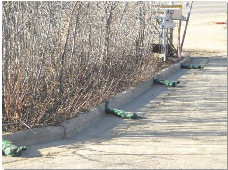
Photograph RS-1. Rock socks placed at regular intervals in a curb line can help reduce sediment loading to storm sewer inlets. Rock socks can also be used as perimeter controls.
