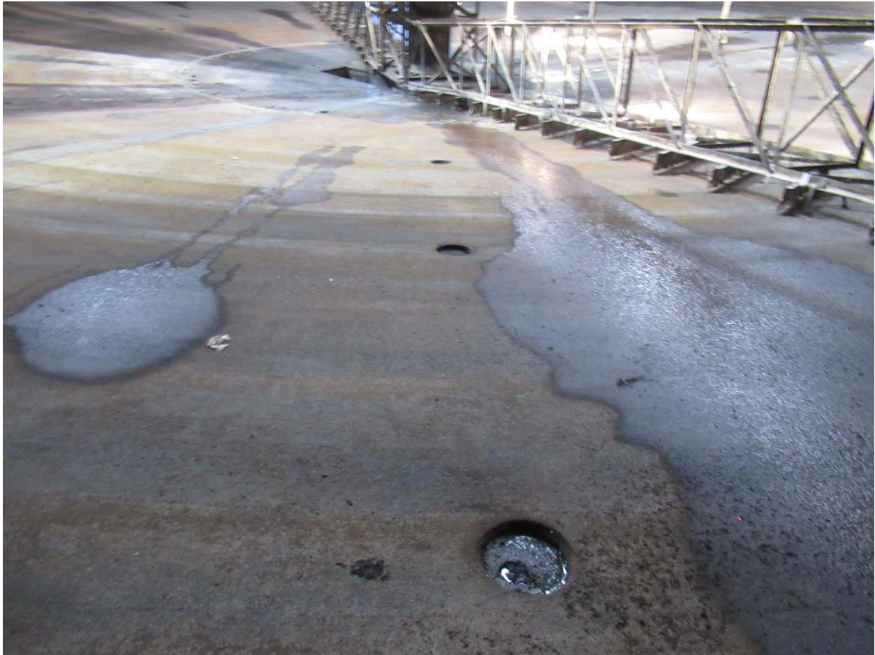
Figure 27. Typical depressions in concrete topping.
