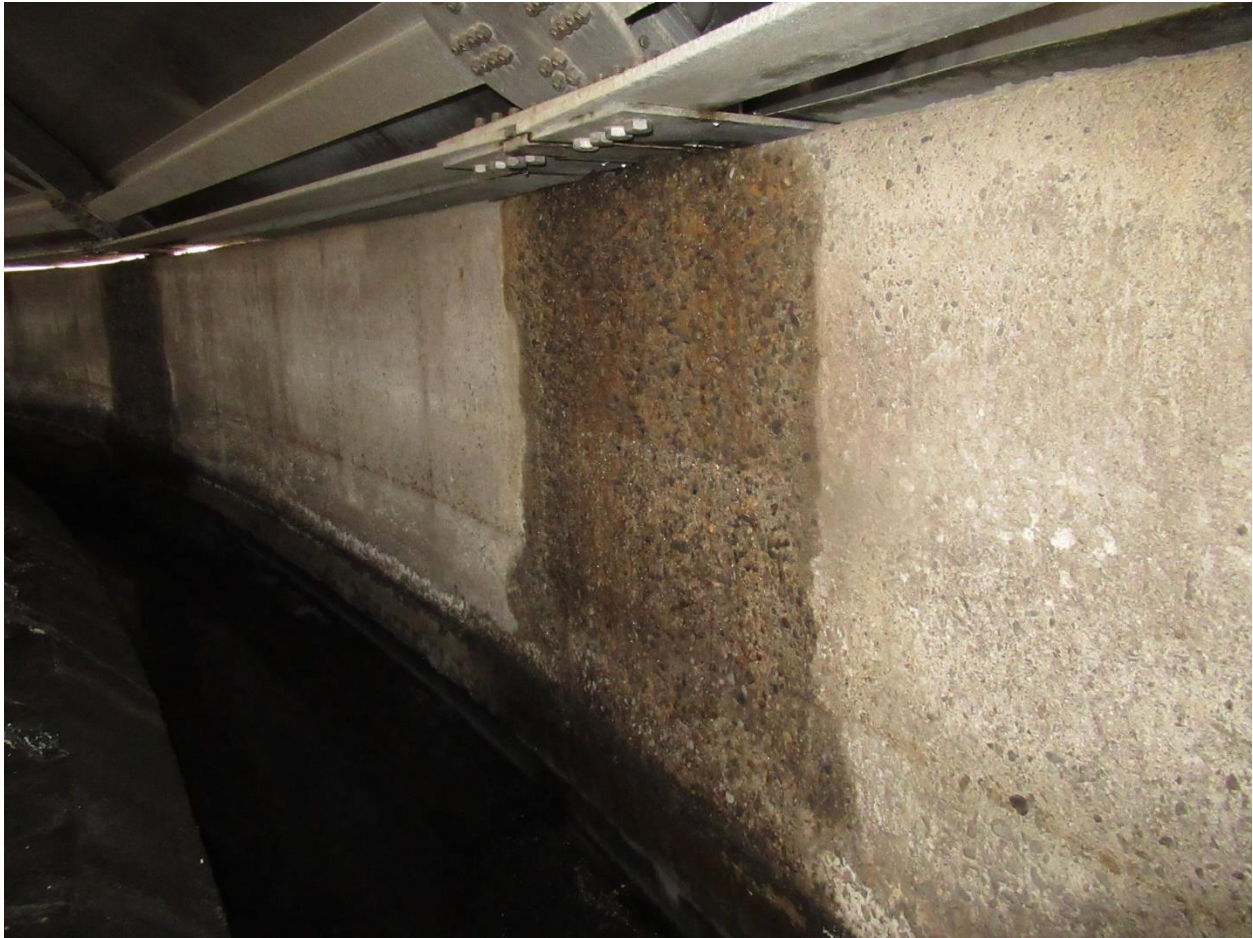
Figure 30. Erosion of concrete surface at trough underneath dome connection nodes.
