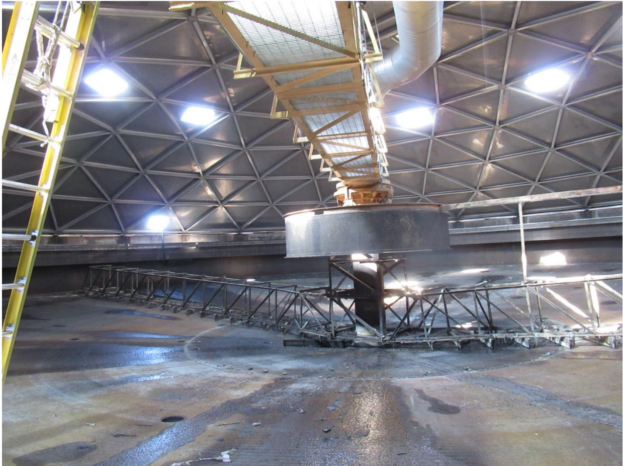
Figure 22. Catwalk bridge and central mechanical equipment.
