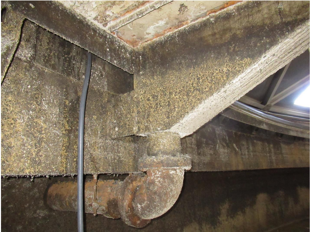
Figure 16. Scum box drain.
