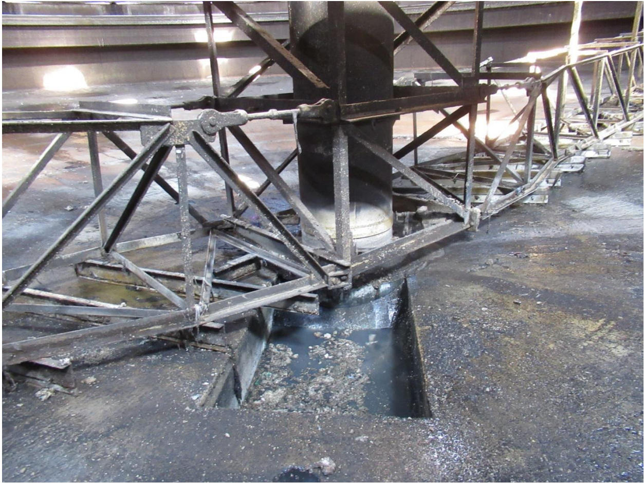
Figure 23. Sludge pit at center of clarifier adjacent to mechanical equipment.
