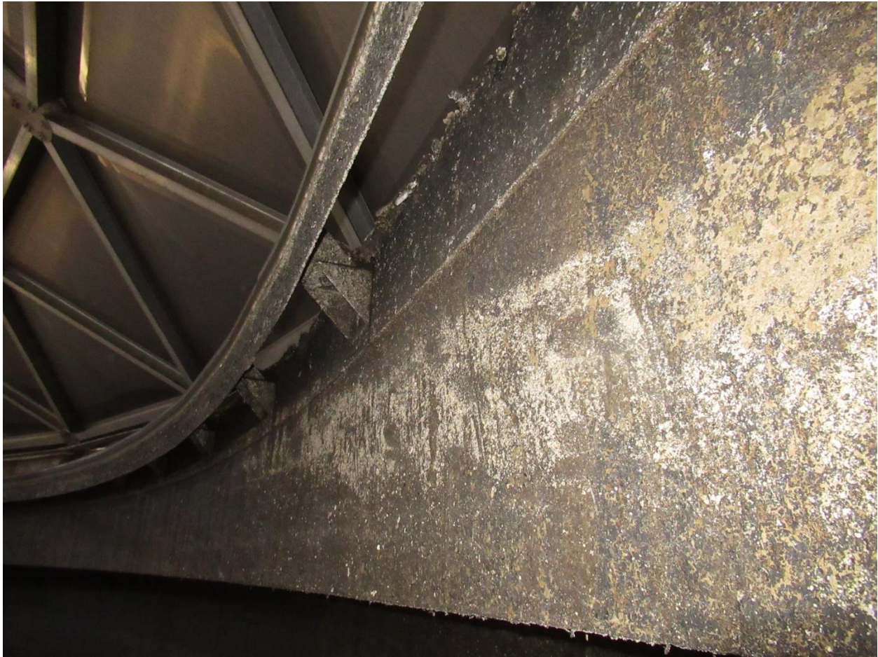
Figure 17. Overall view of weir plate and scum baffle at exterior side of trough.
