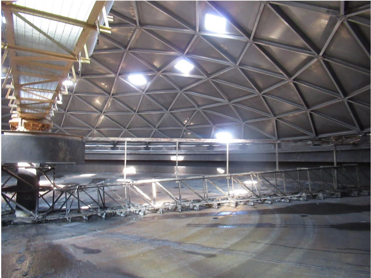
Figure 24. Scum and bottom screed at base of clarifier.
