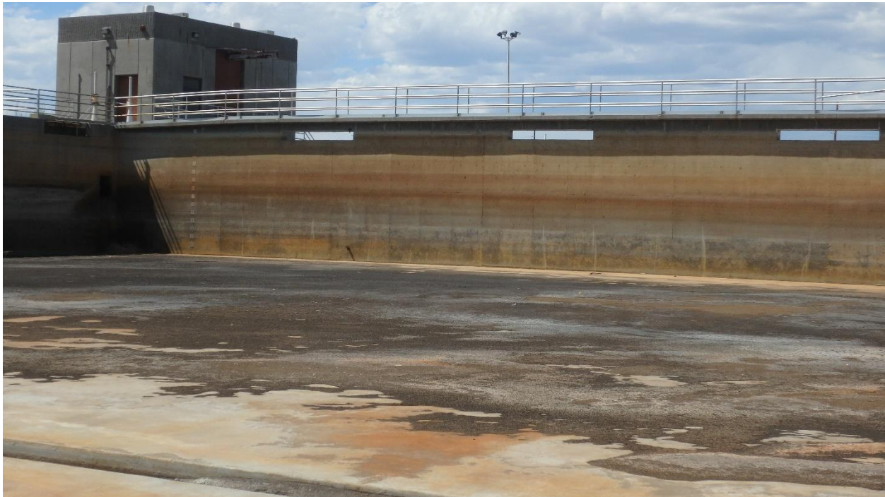
Figure 2. Closeup of the west end of the north dividing wall showing slope down (June 2020).
