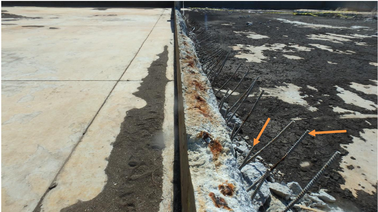
Figure 6. Typical condition of bent #6 reinforcing, at 5 1/2" on-center, from the slab to be repaired.
