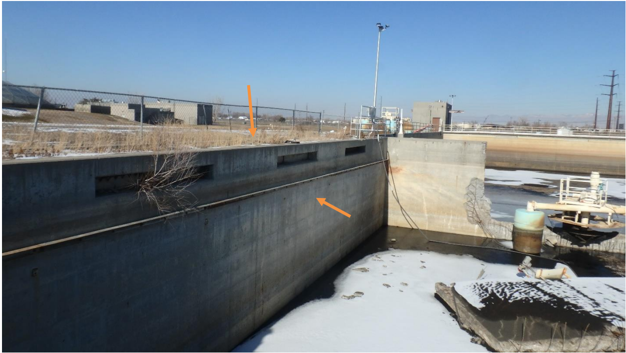
Figure 7. Chlorine contract area/chamber adjacent to south wall which has been filled with soil.
