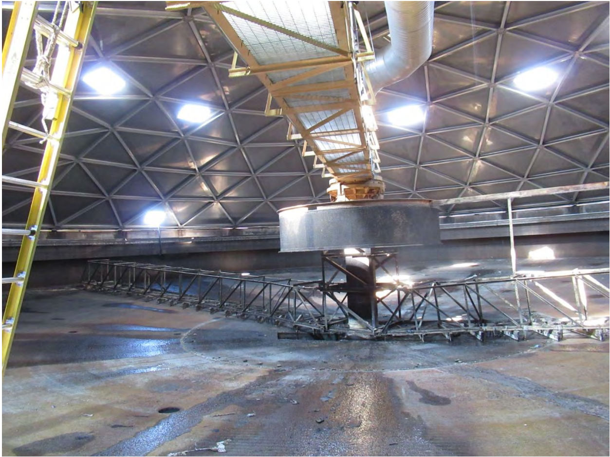
Figure 22. Catwalk bridge and central mechanical equipment.
