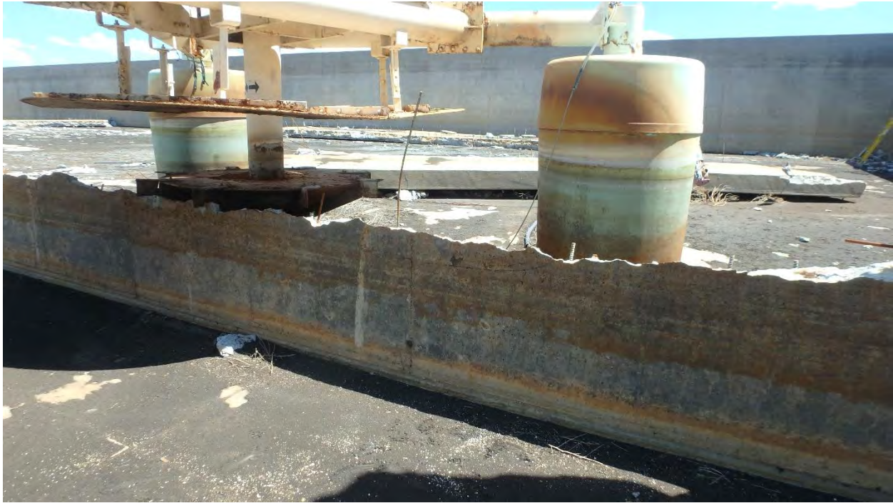
Figure 5. Remaining roughly 3'-0" tall portion of the south dividing wall where collapsed.
