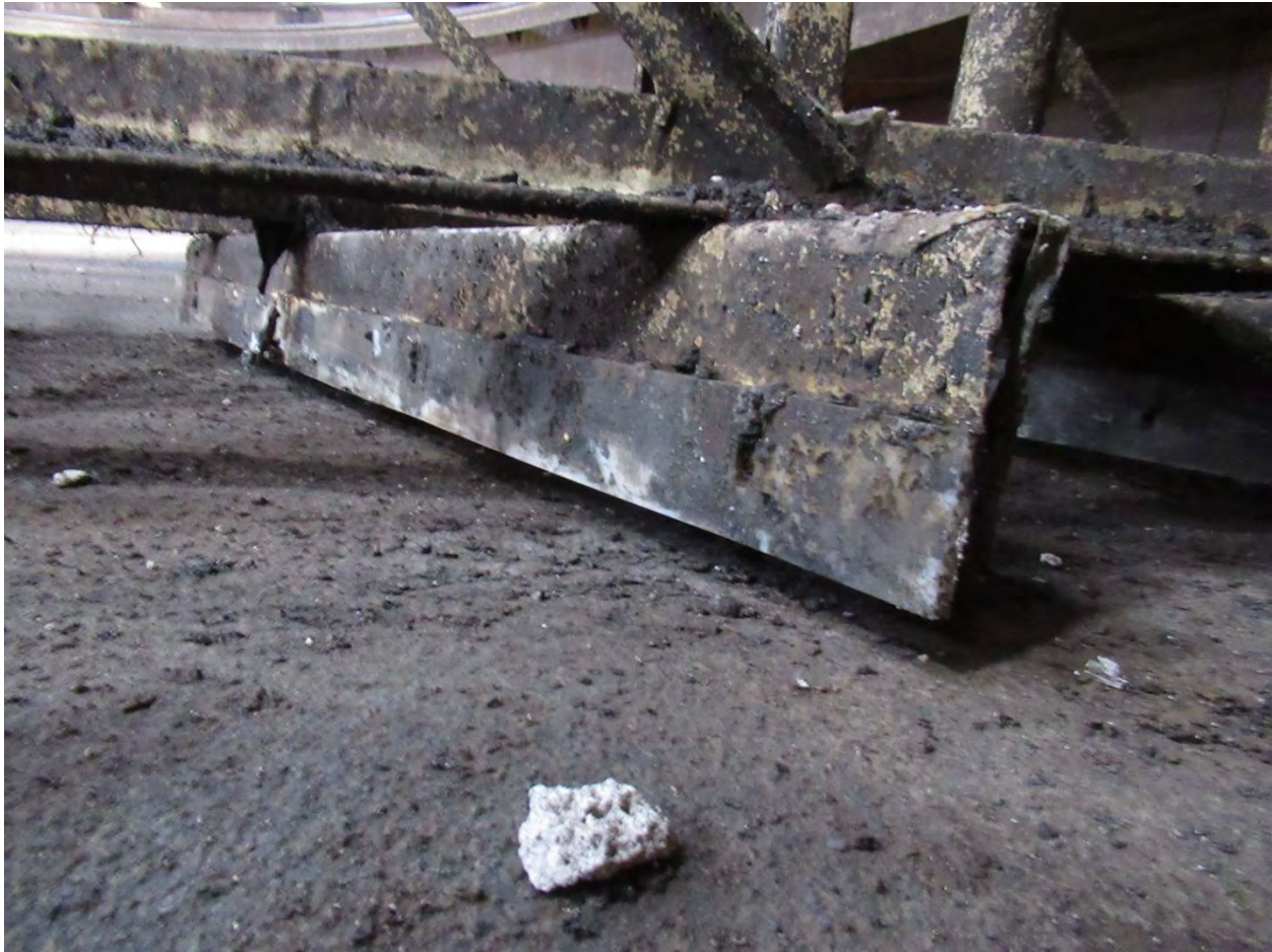
Figure 26. Close-up of bottom screed plate. Blade height will be adjusted by Owner.
