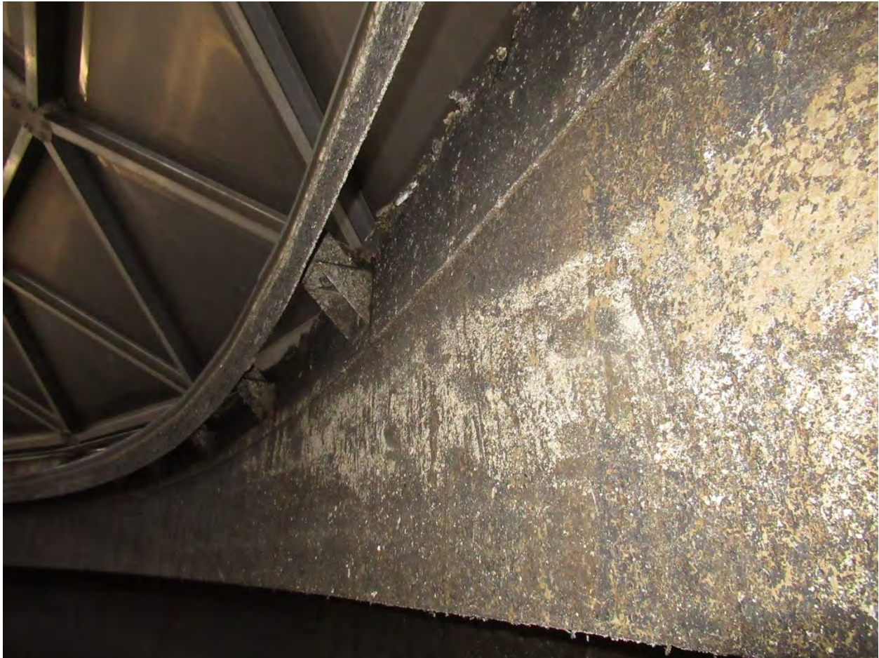
Figure 17. Overall view of weir plate and scum baffle at exterior side of trough.
