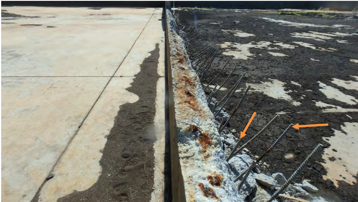
Figure 6. Typical condition of bent #6 reinforcing, at 5 1/2" on-center, from the slab to be repaired.
