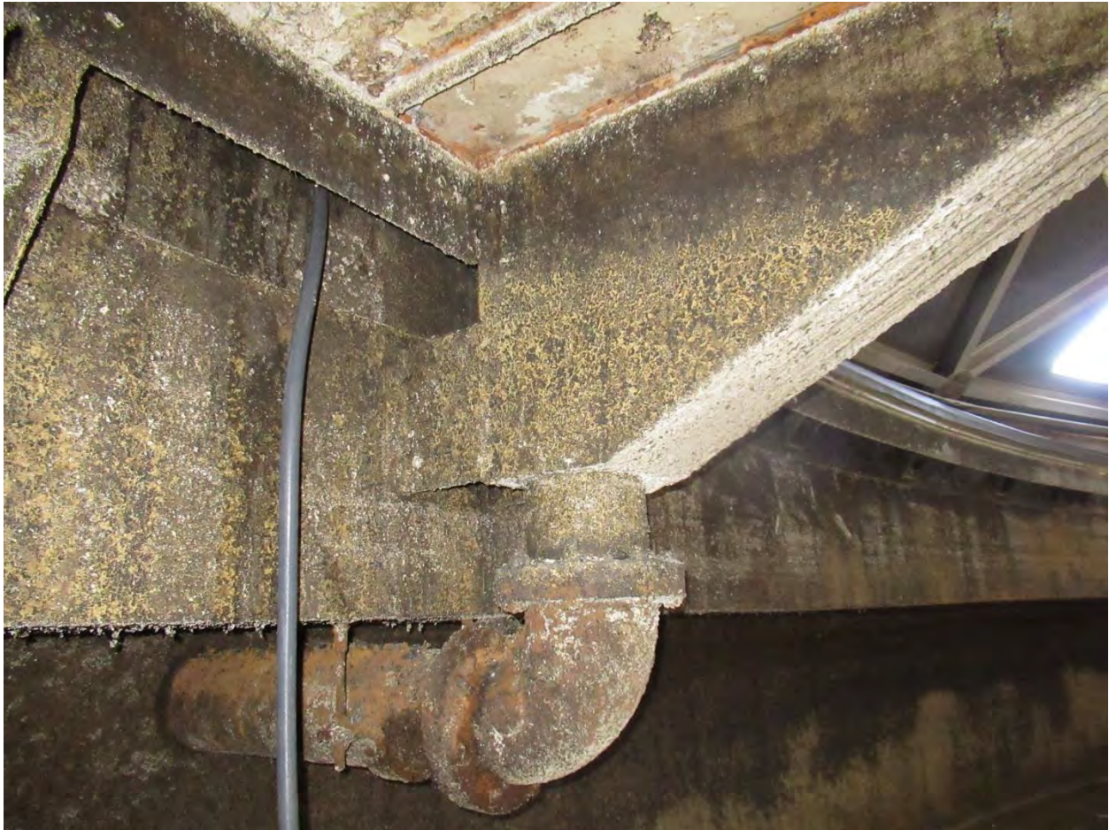
Figure 16. Scum box drain.
