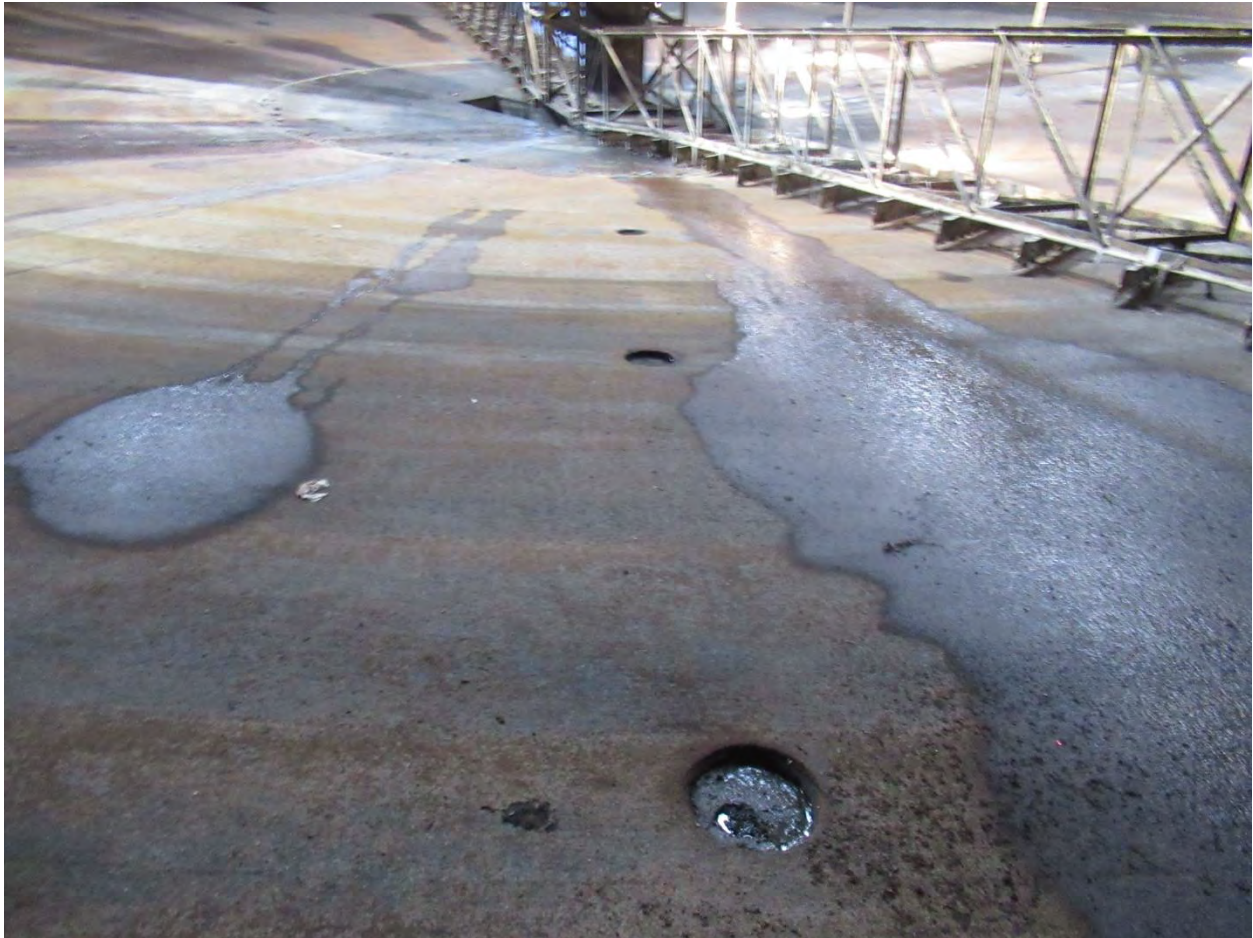
Figure 27. Typical depressions in concrete topping.
