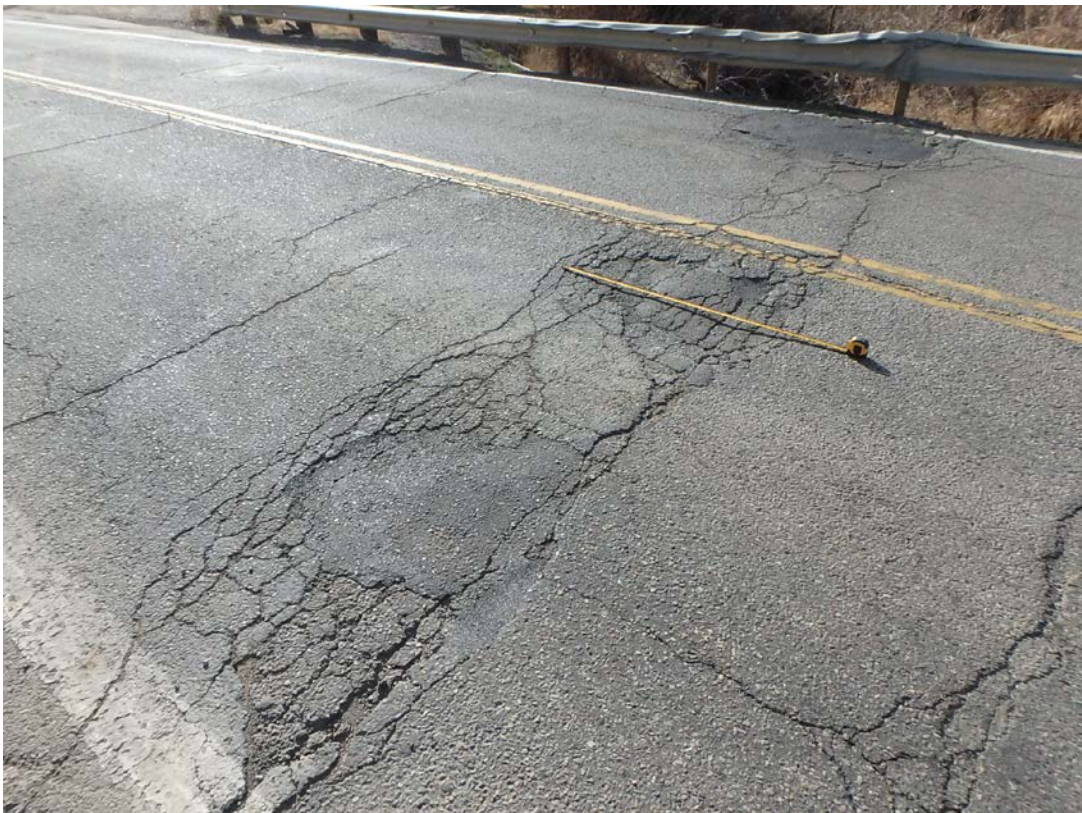
Cracked, Broken-Up Asphalt with Patched Potholes and Depressions at West End of Deck
