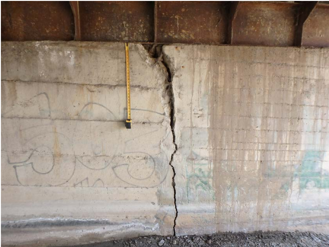
Spalling along Vertical Crack in East Abutment
