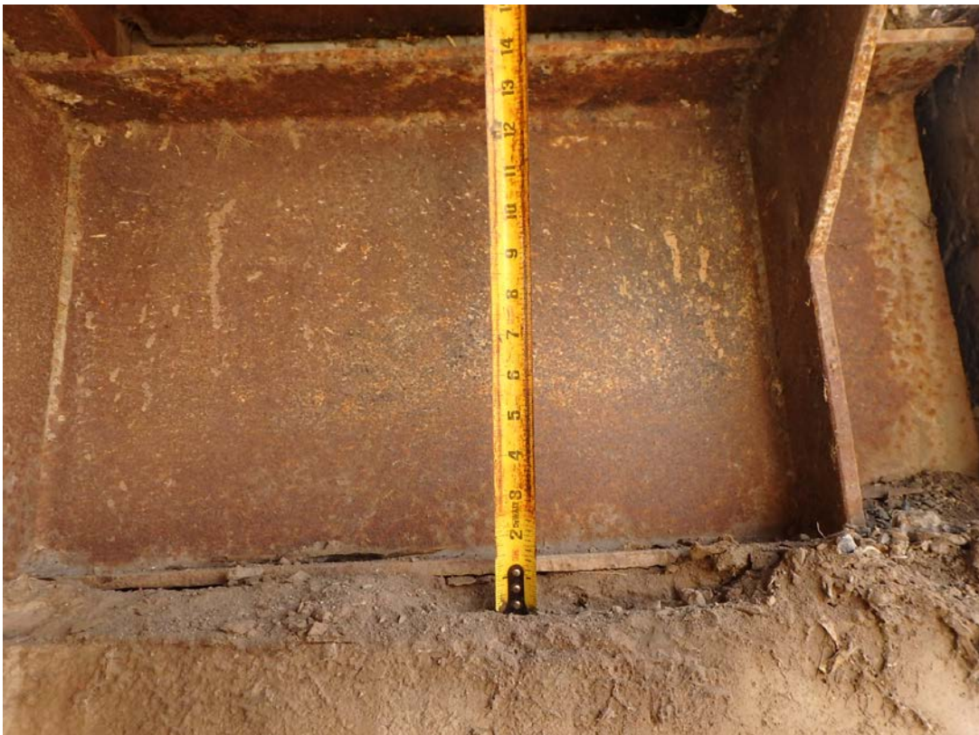
Gap between East Abutment Wall and Cap indicating Settling of South End of Wall
