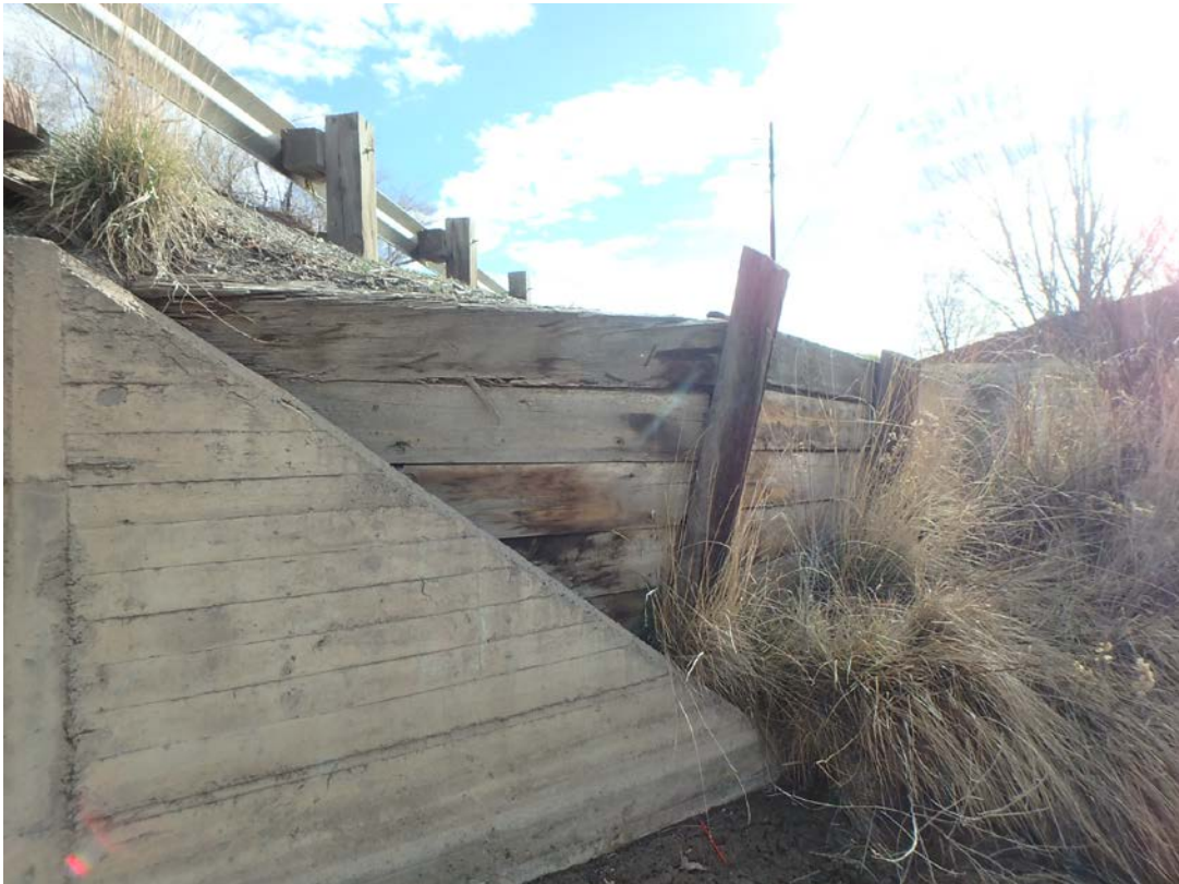
Southeast Wingwall Extension Leaning into Channel
