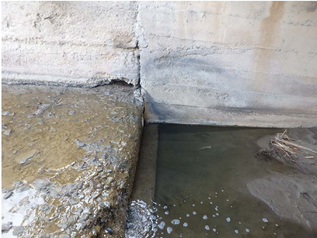
Scour Hole and Spall/Void at North End of East Abutment
