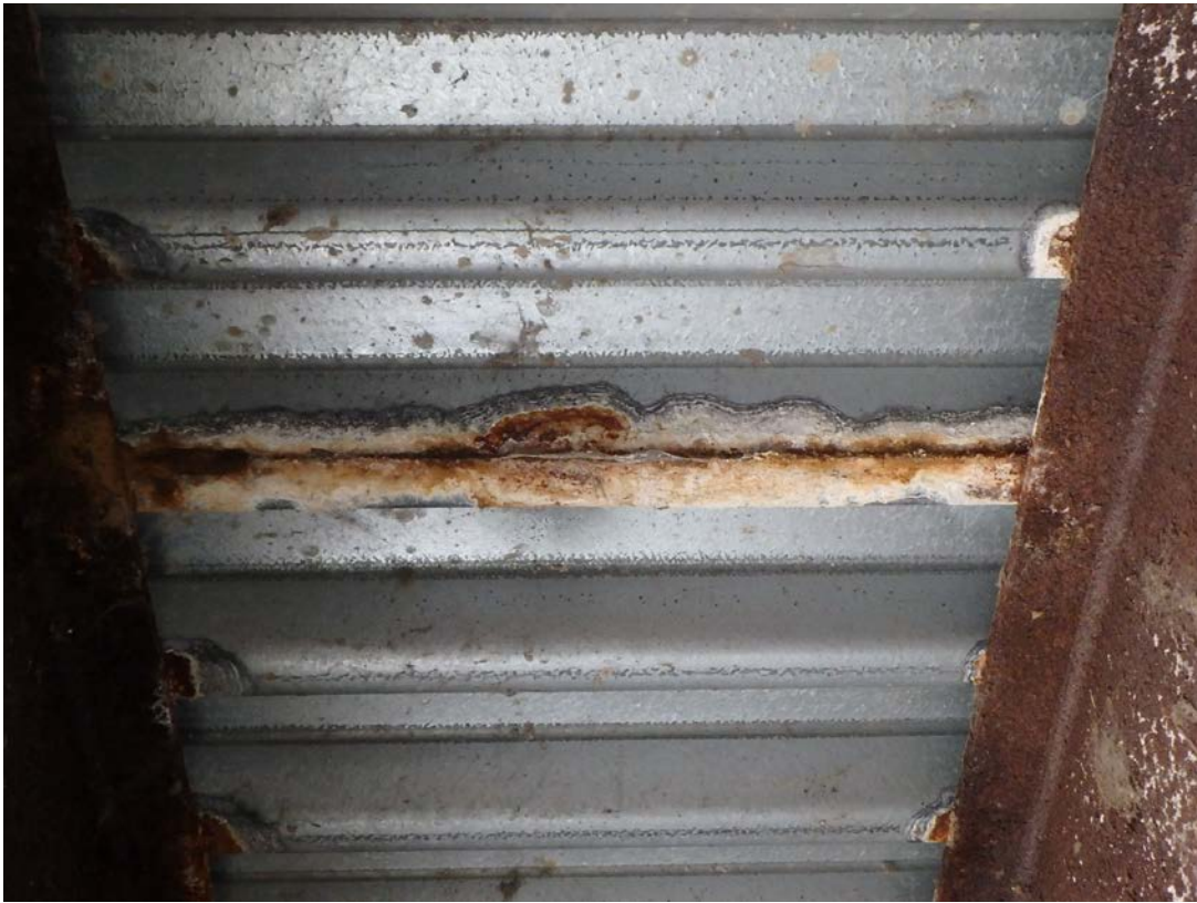
Typical Rust and Corrosion along Deck Joints and at Contact Points with Top Flanges
