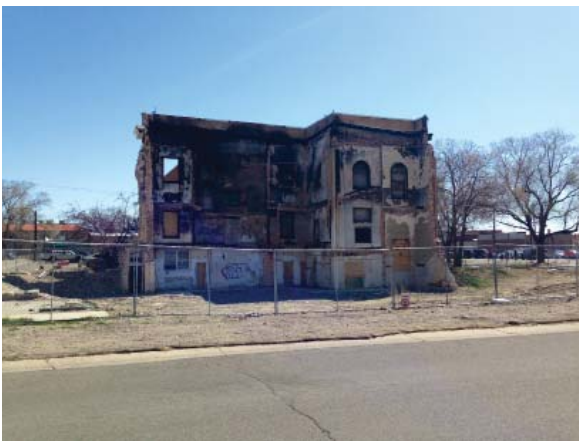
Image 3. White Hall as it stands today, with a demolished west-facing wall and open pit.
