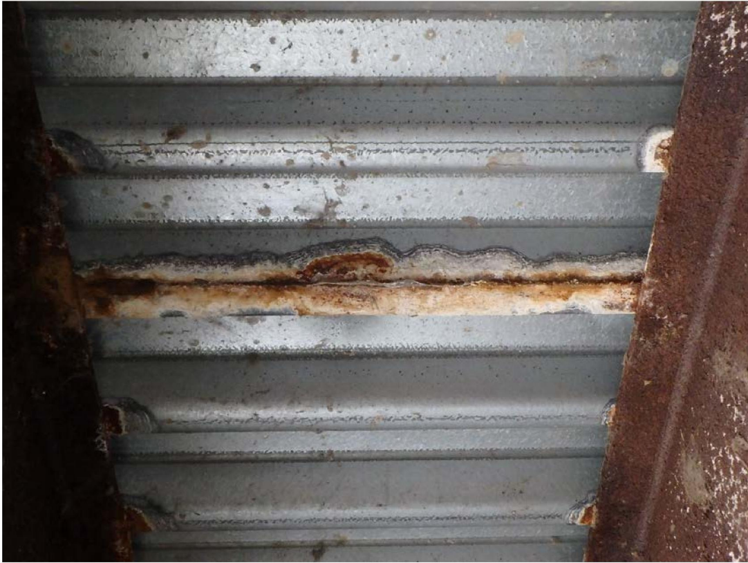
Typical Rust and Corrosion along Deck Joints and at Contact Points with Top Flanges
