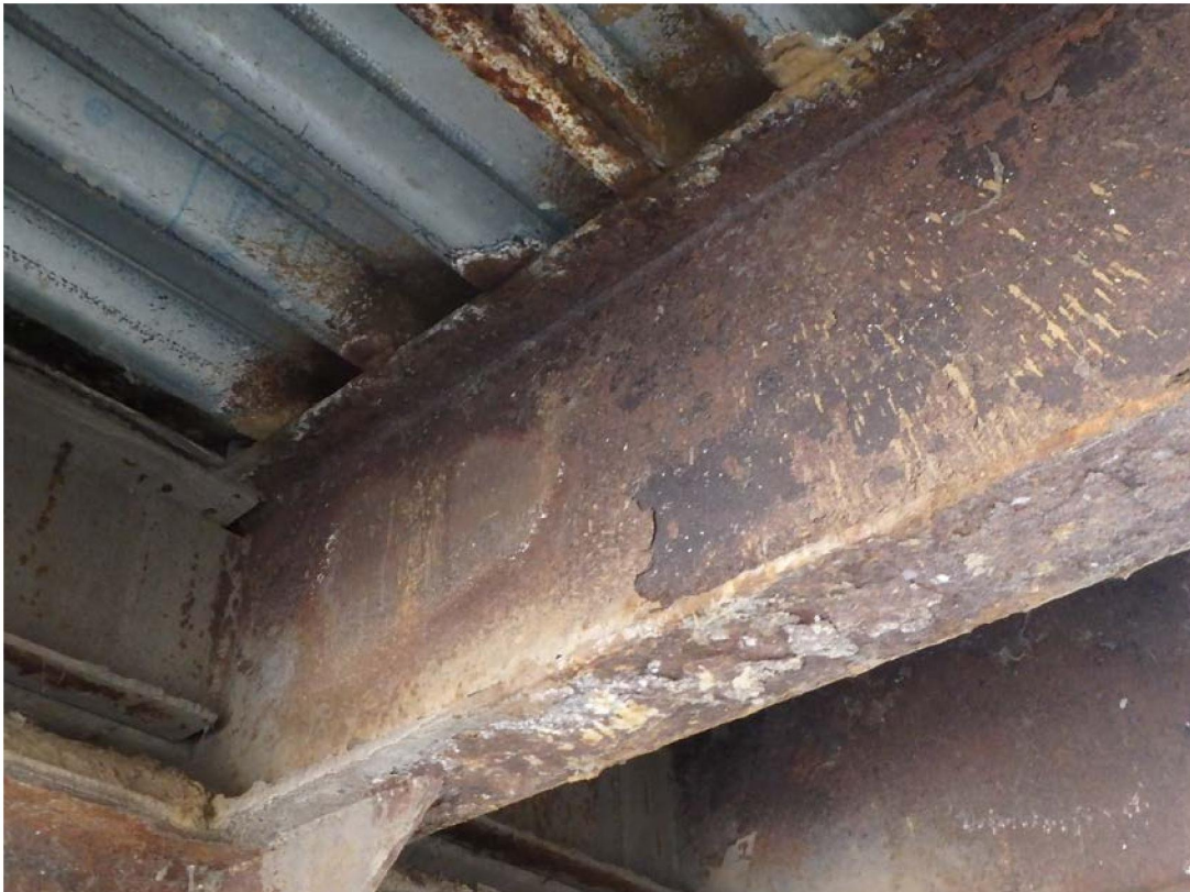
Flaking Rust Typical on Girders, Especially below Corroded Deck Joints
