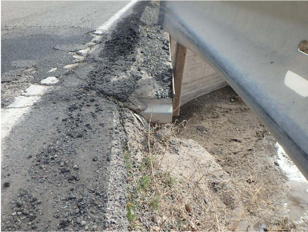
Exposed Abutment Backwall due to Erosion at Southwest Corner of Deck
