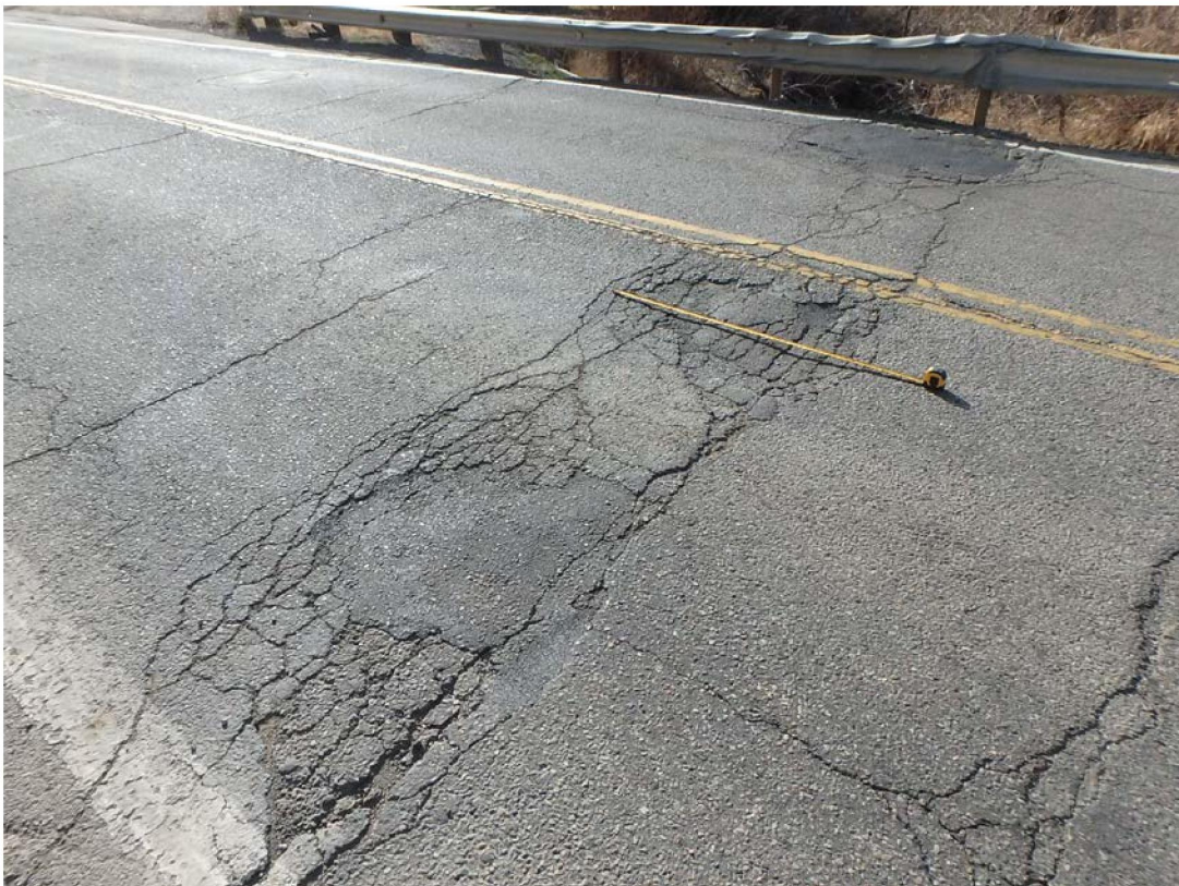
Cracked, Broken-Up Asphalt with Patched Potholes and Depressions at West End of Deck
