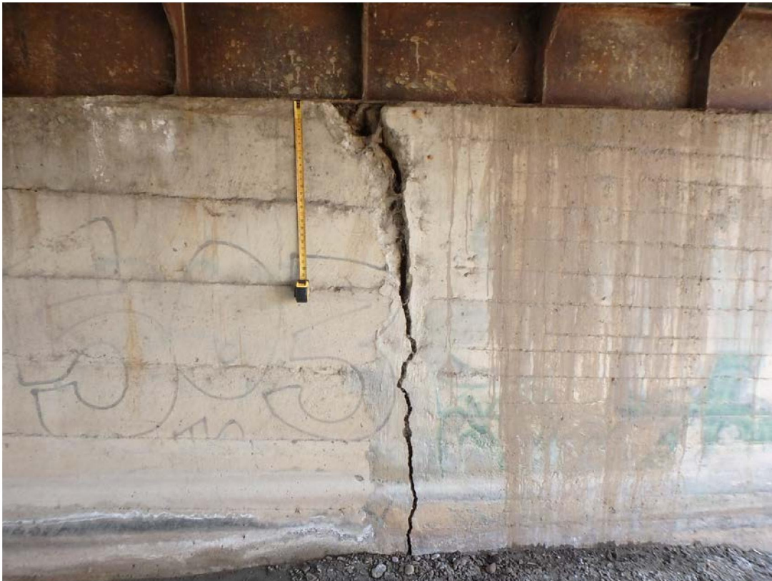
Spalling along Vertical Crack in East Abutment
