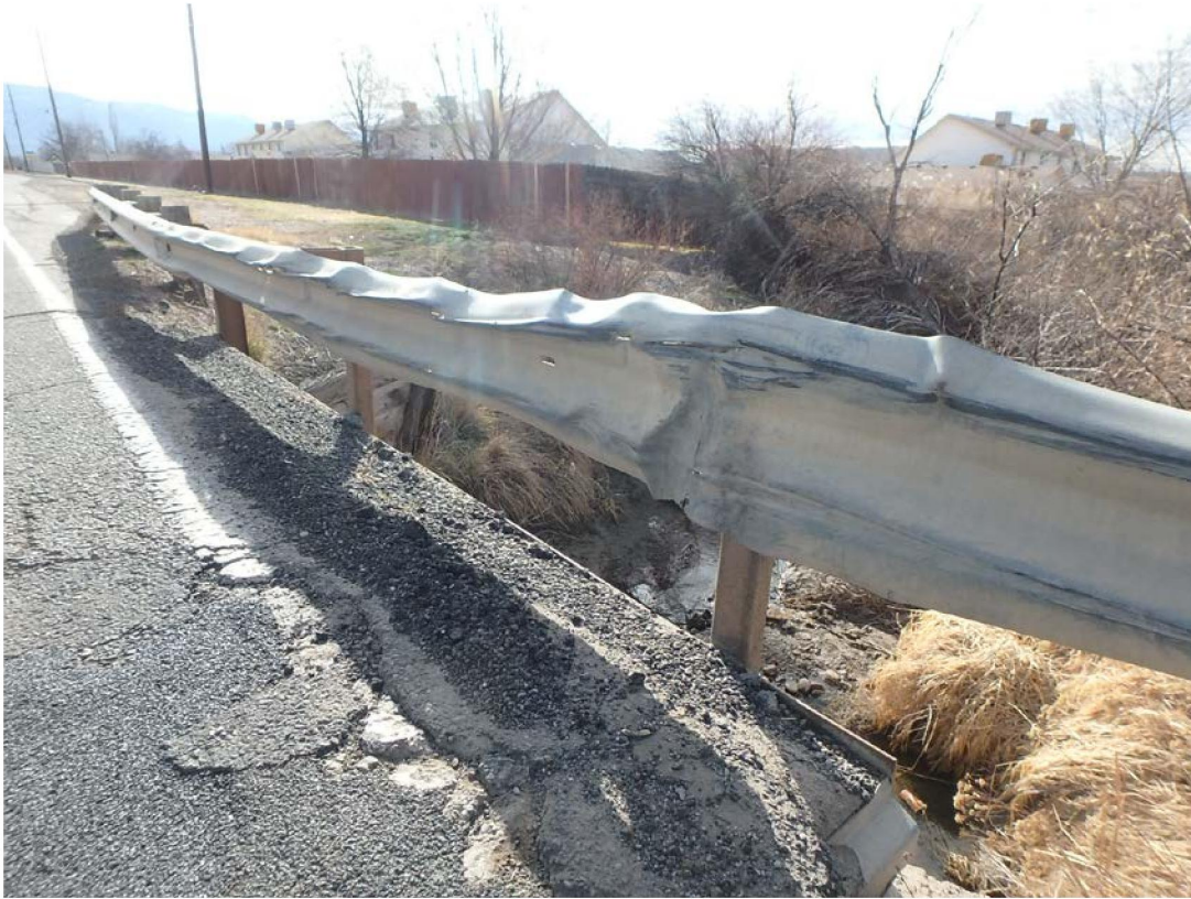
Damaged W-Beam of South Bridge Rail, Mostly at West End
