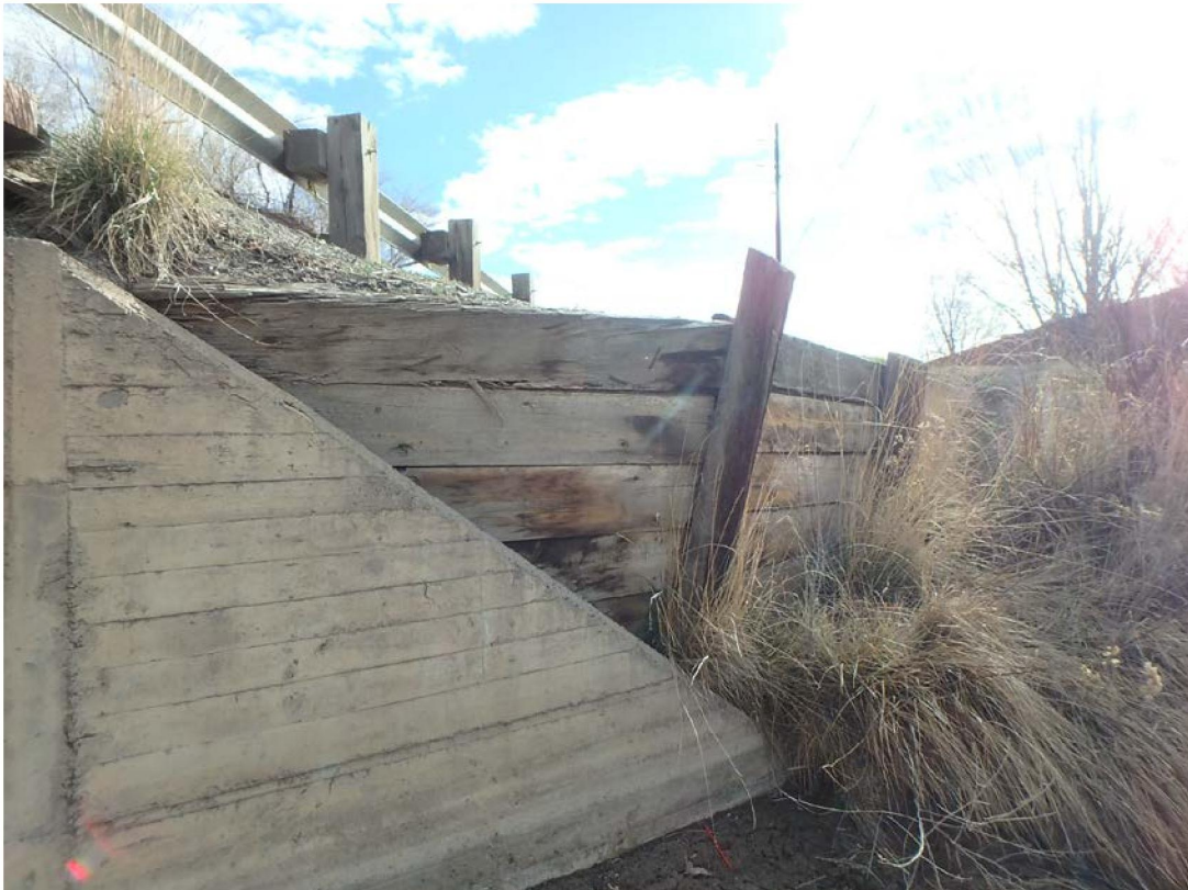
Southeast Wingwall Extension Leaning into Channel
