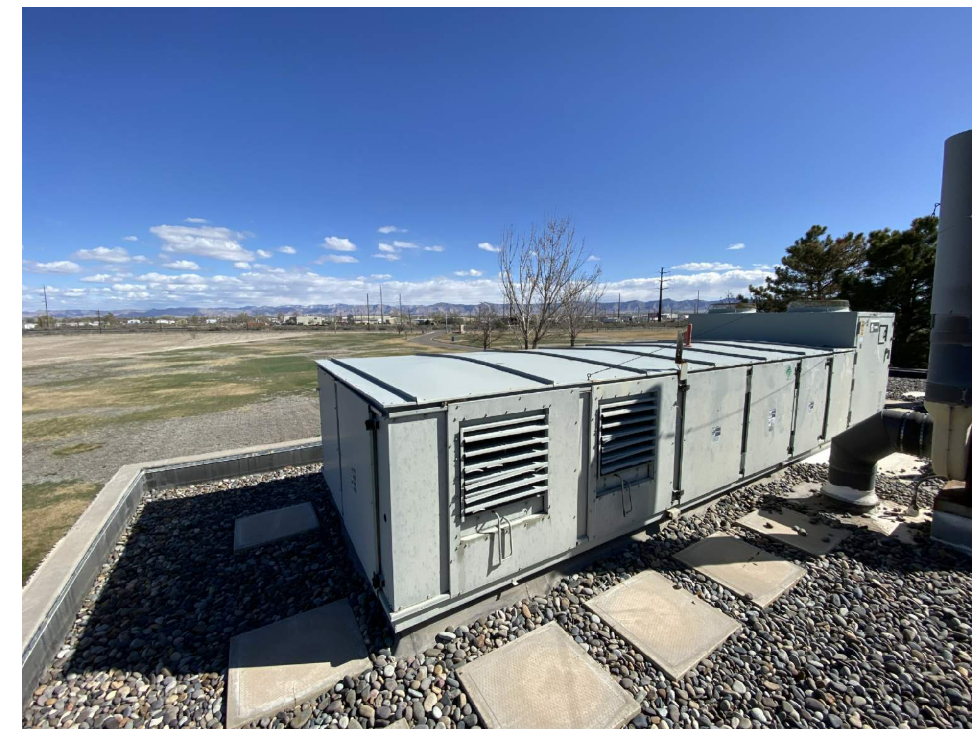
EXISTING LABORATORY TRANE INTELLIPAK
