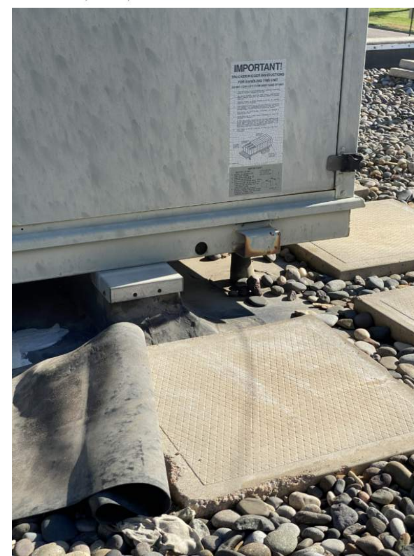
EXISTING LABORATORY TRANE INTELLIPAK THROUGH THE BASE POWER CONNECTION
