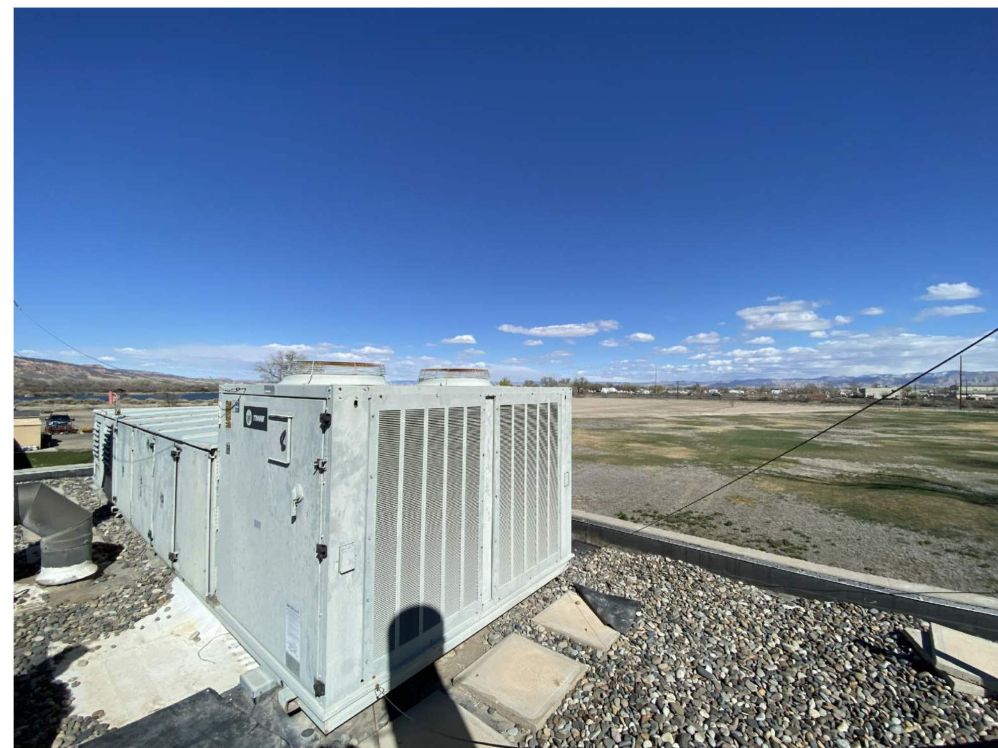
EXISTING LABORATORY TRANE INTELLIPAK
