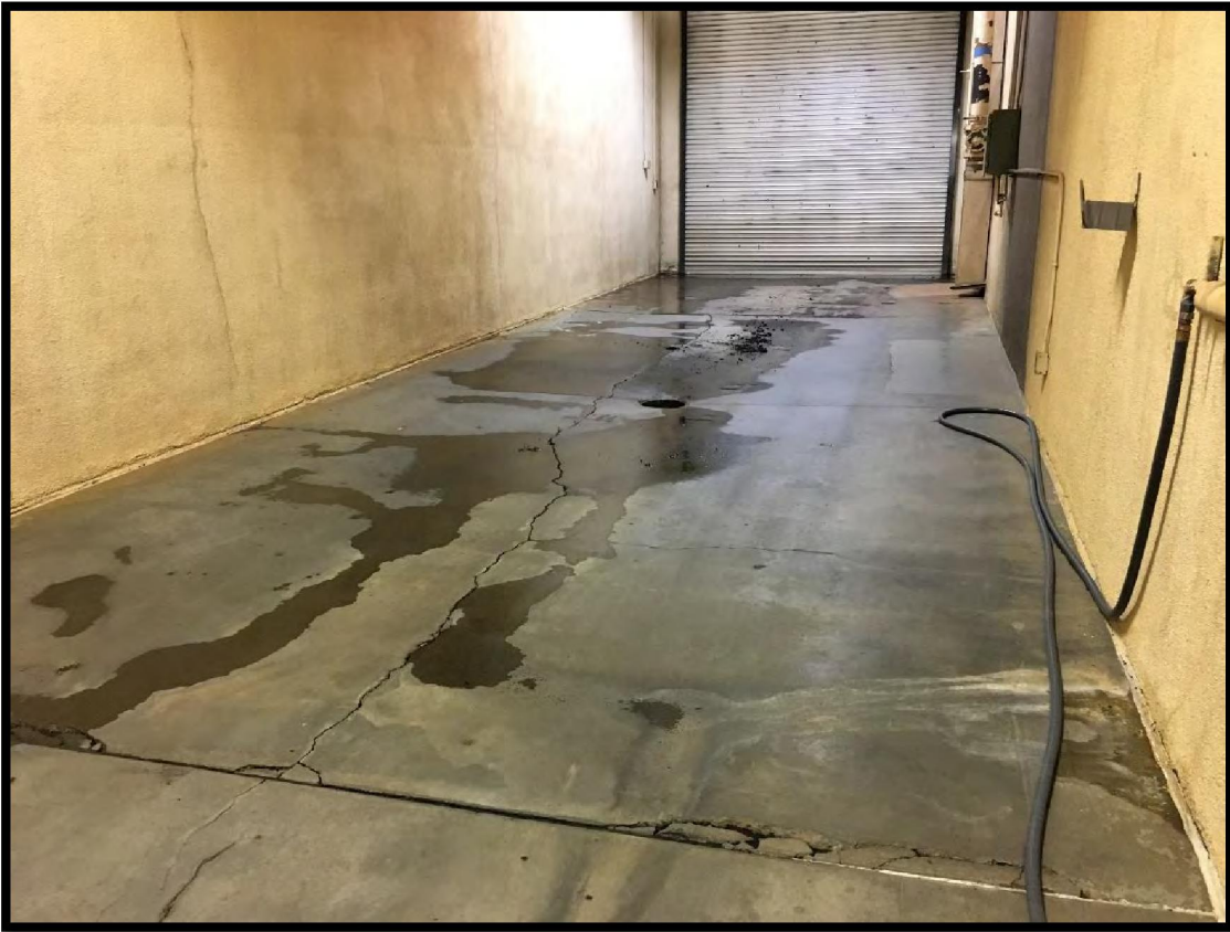
Picture 25, Aerobic Digester Concrete and Wall Cracks (Truck Sludge Loading)
