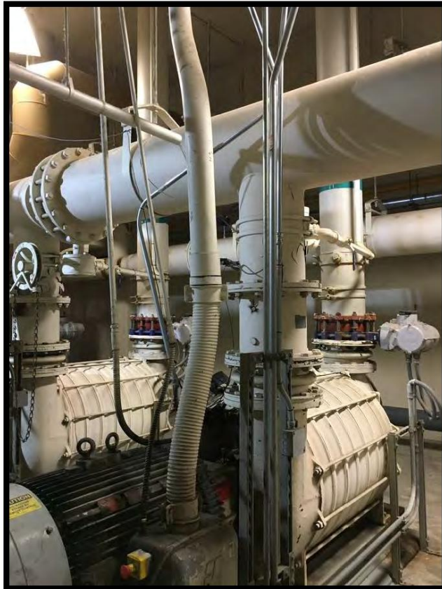
Picture 14, Aerobic Basin Blowers
