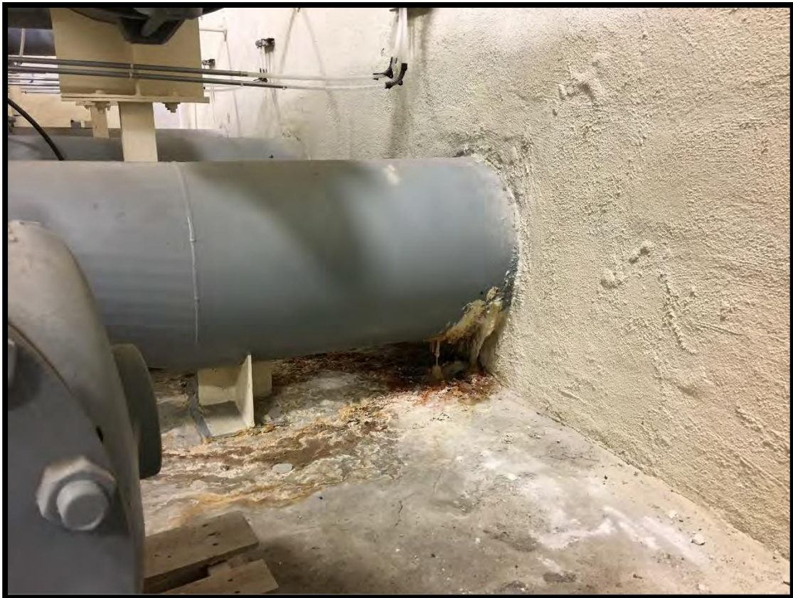
Picture 6, Raw Sewage Station Pump Inlet Pipe
