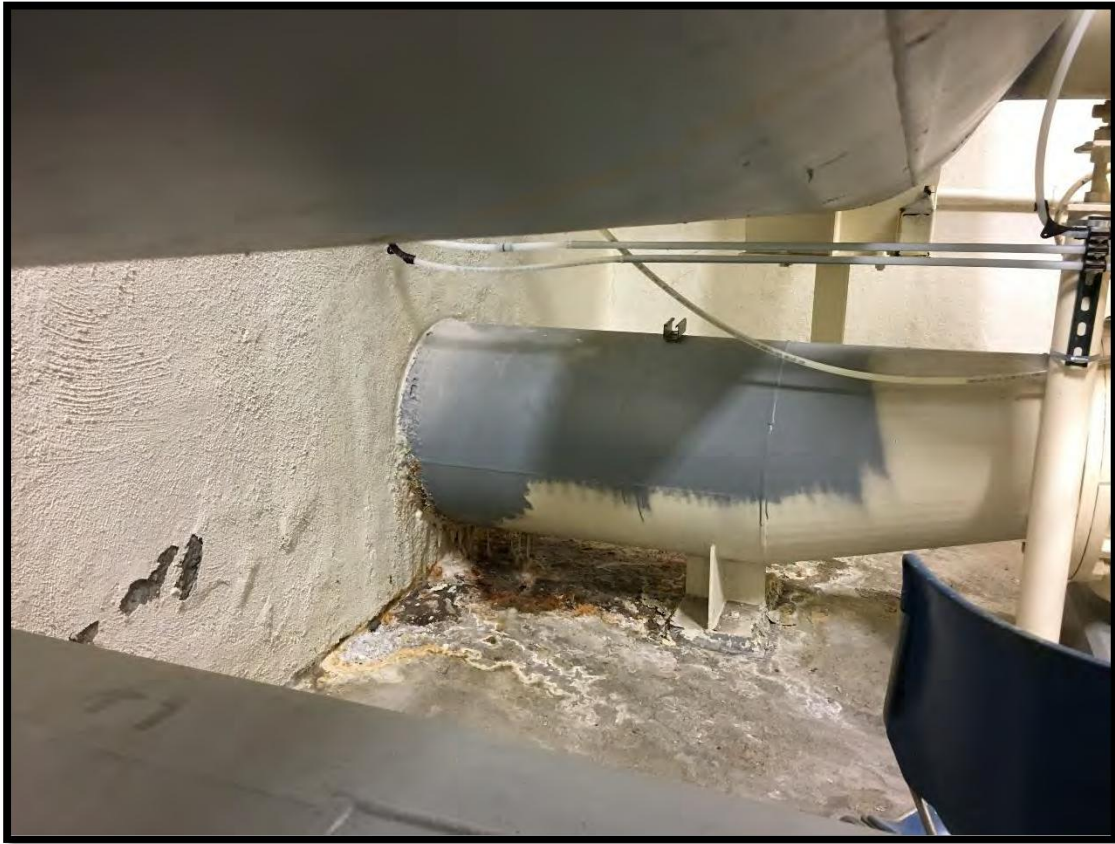
Picture 5, Raw Sewage Station Pump Inlet Pipe
