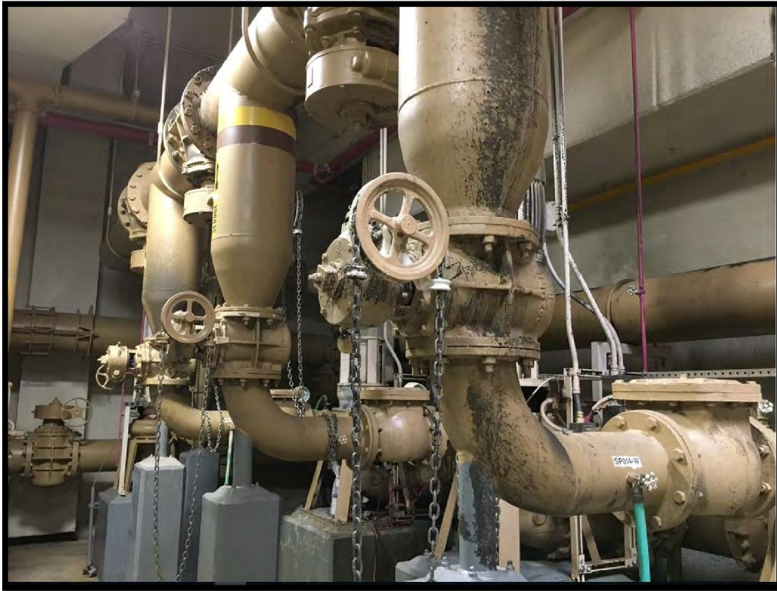
Picture 17, Aerobic Basin Basement Pump Pipe with spray from reducer leak
