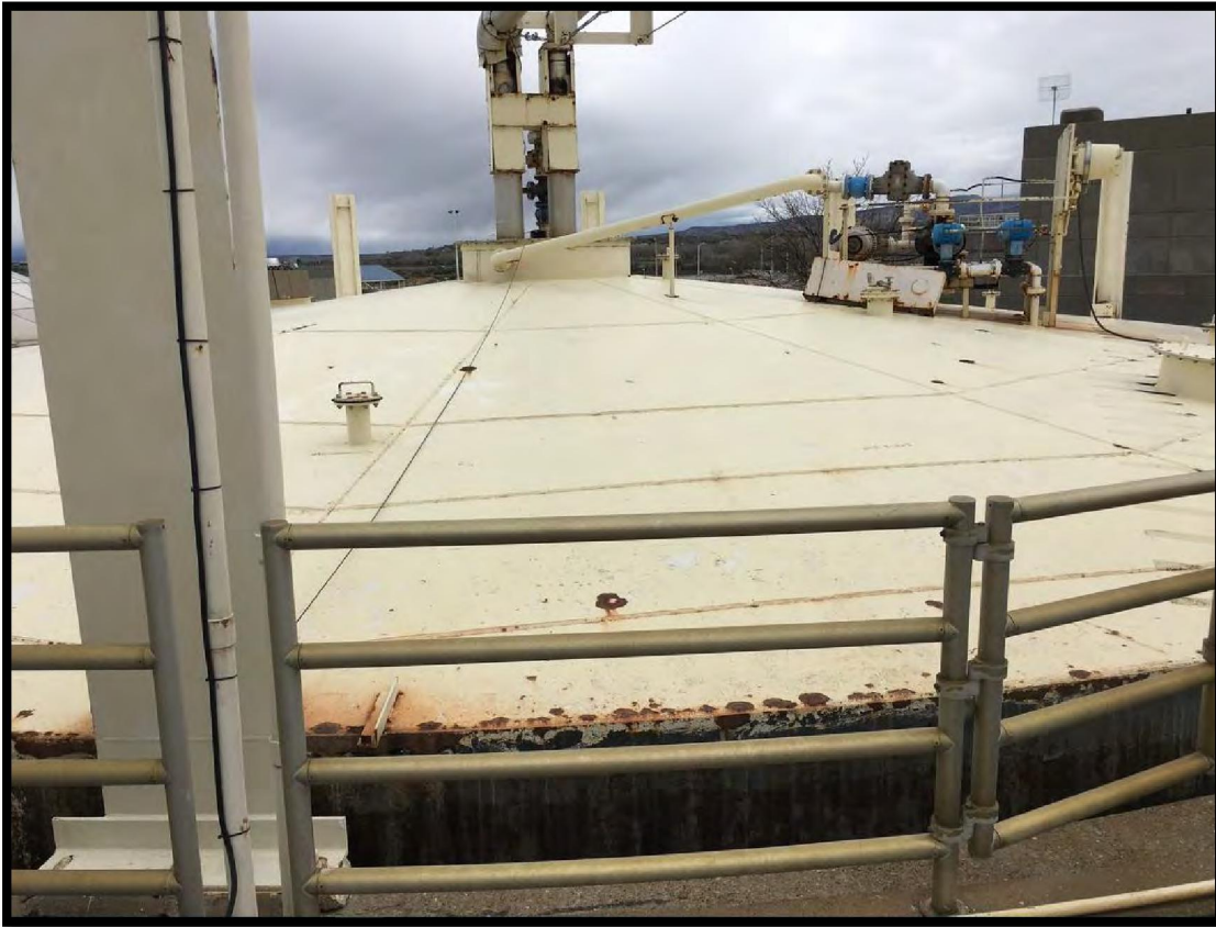
Picture 33 Anaerobic Digester Tank Roof (floating lid)
