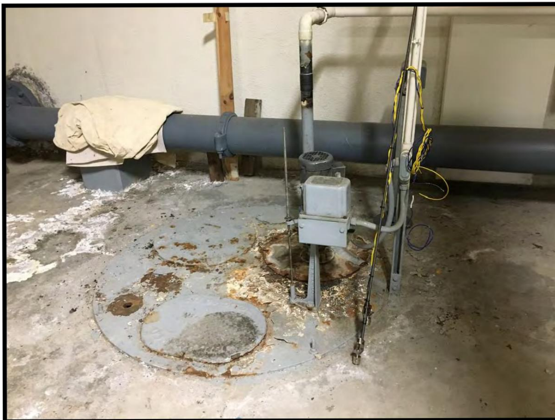
Picture 12, Aerobic Basin and Piping
