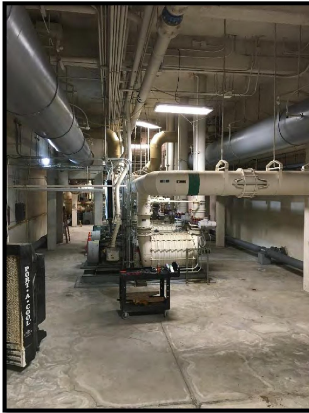
Picture 9, Aerobic Basin Basement Floor (Blowers)
