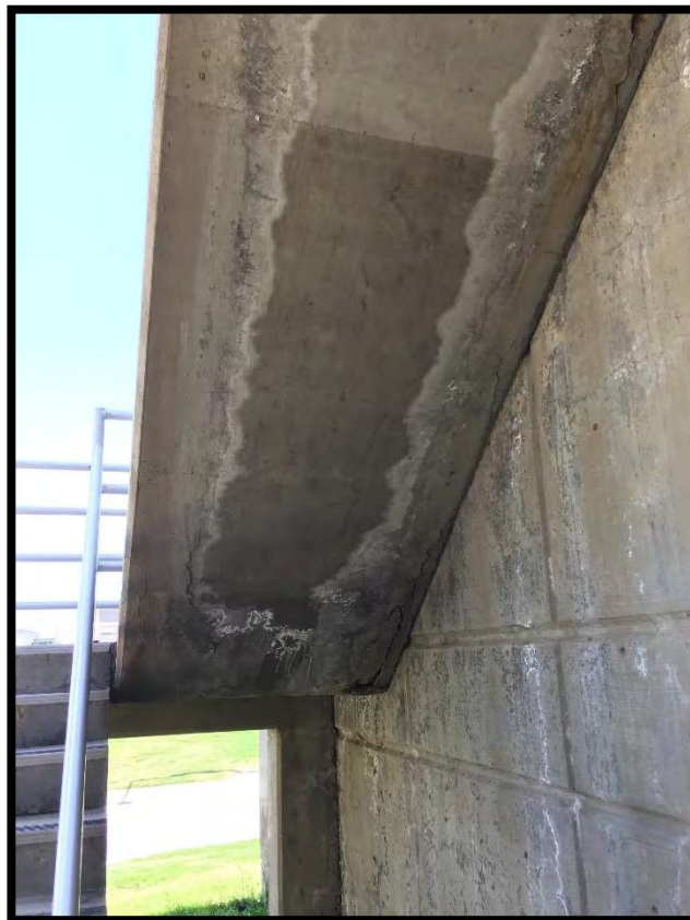
Picture 24, Aerobic Digester Stairway, Rebar erosion in concrete
