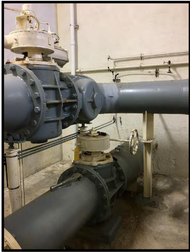
Picture 7, Raw Sewage Station Pump Inlet Pipe Erosion on Elbow
