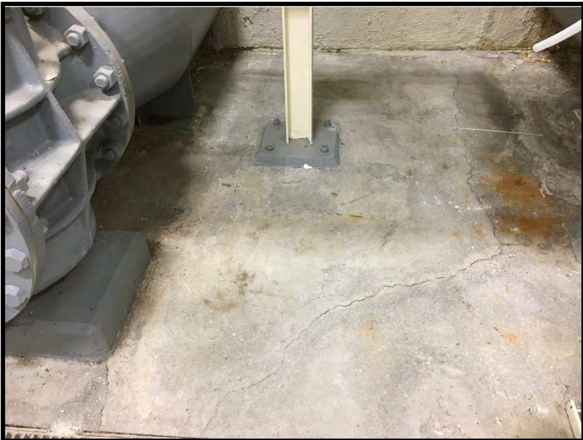
Picture 4, Raw Sewage Station Floor
