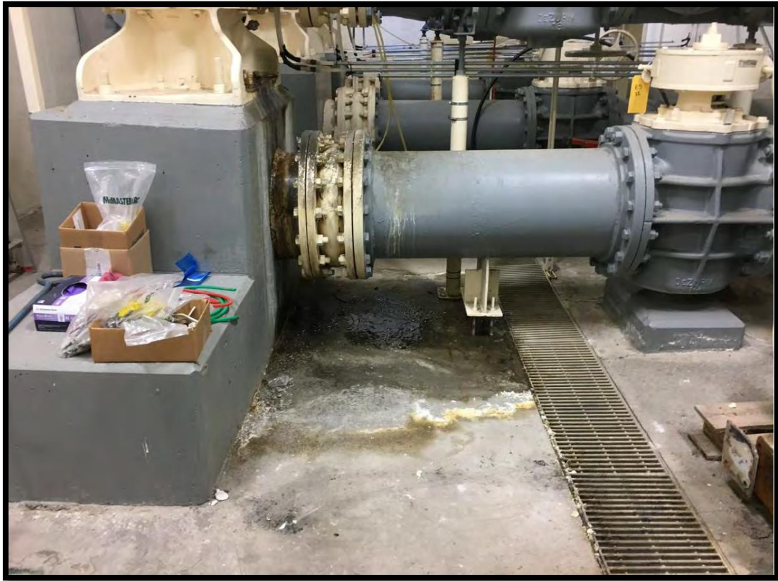
Picture 3, Raw Sewage Station Pump, Pipe and Floor
