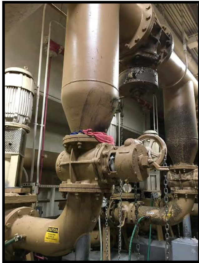
Picture 16, Aerobic Basin Basement Pump Pipe Erosion at Reducer Flange
