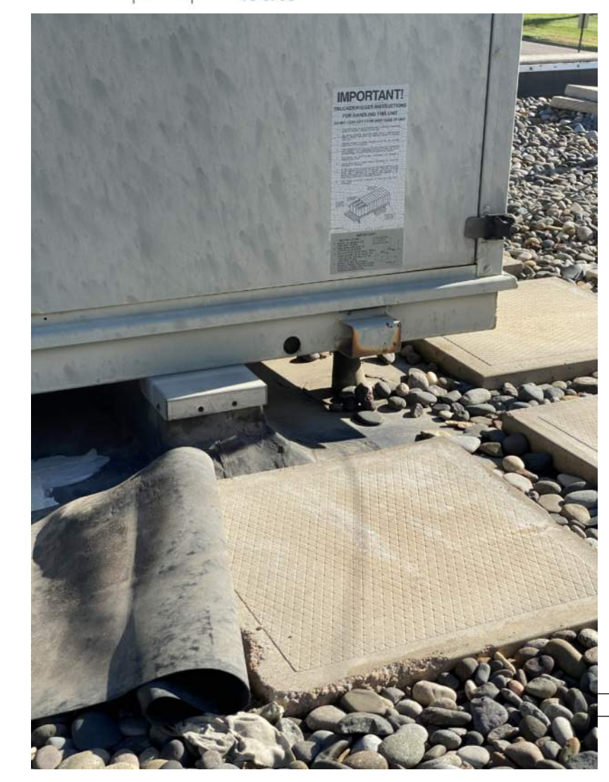
EXISTING LABORATORY TRANE INTELLIPAK THROUGH THE BASE POWER CONNECTION
