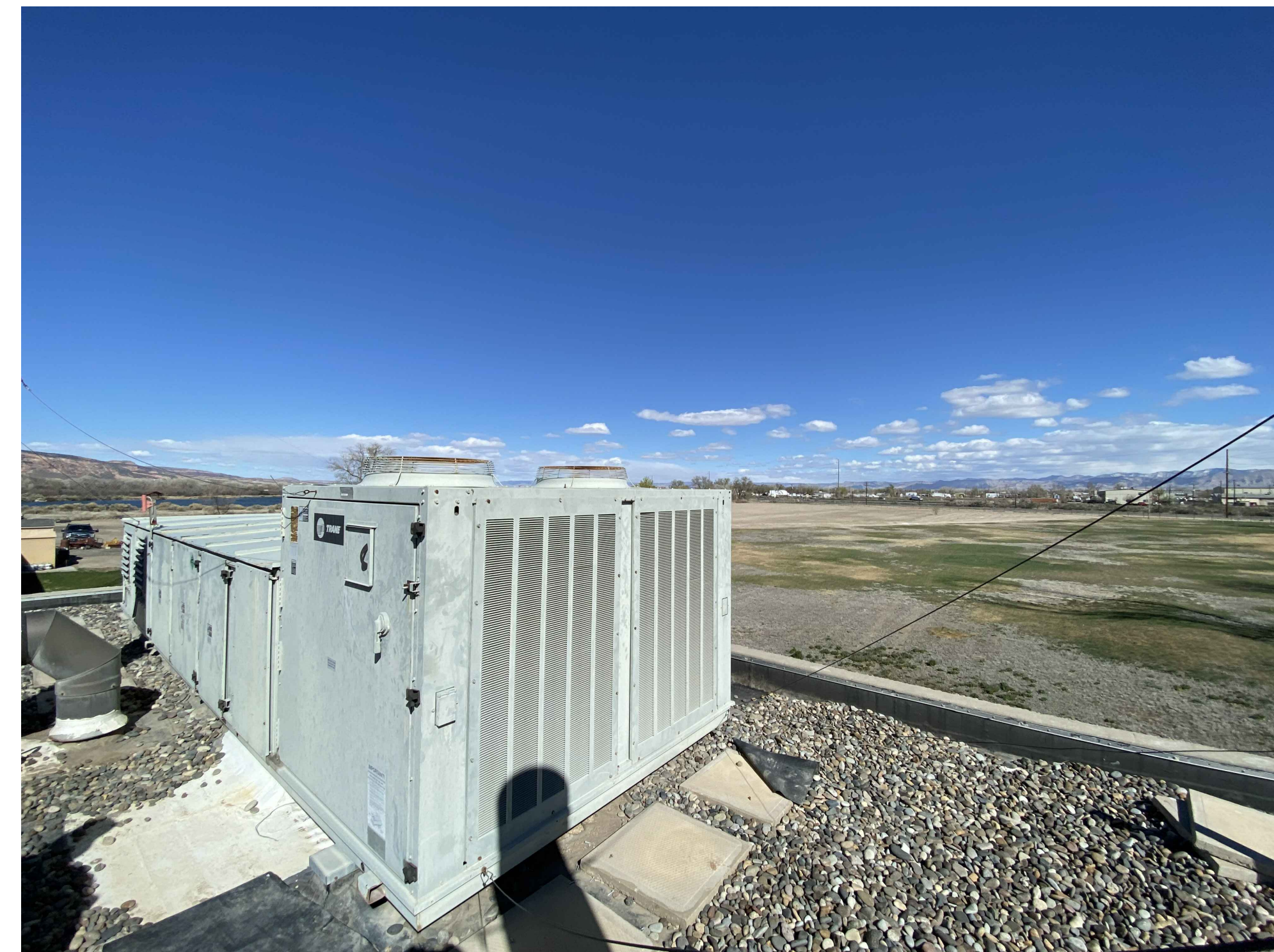
EXISTING LABORATORY TRANE INTELLIPAK
