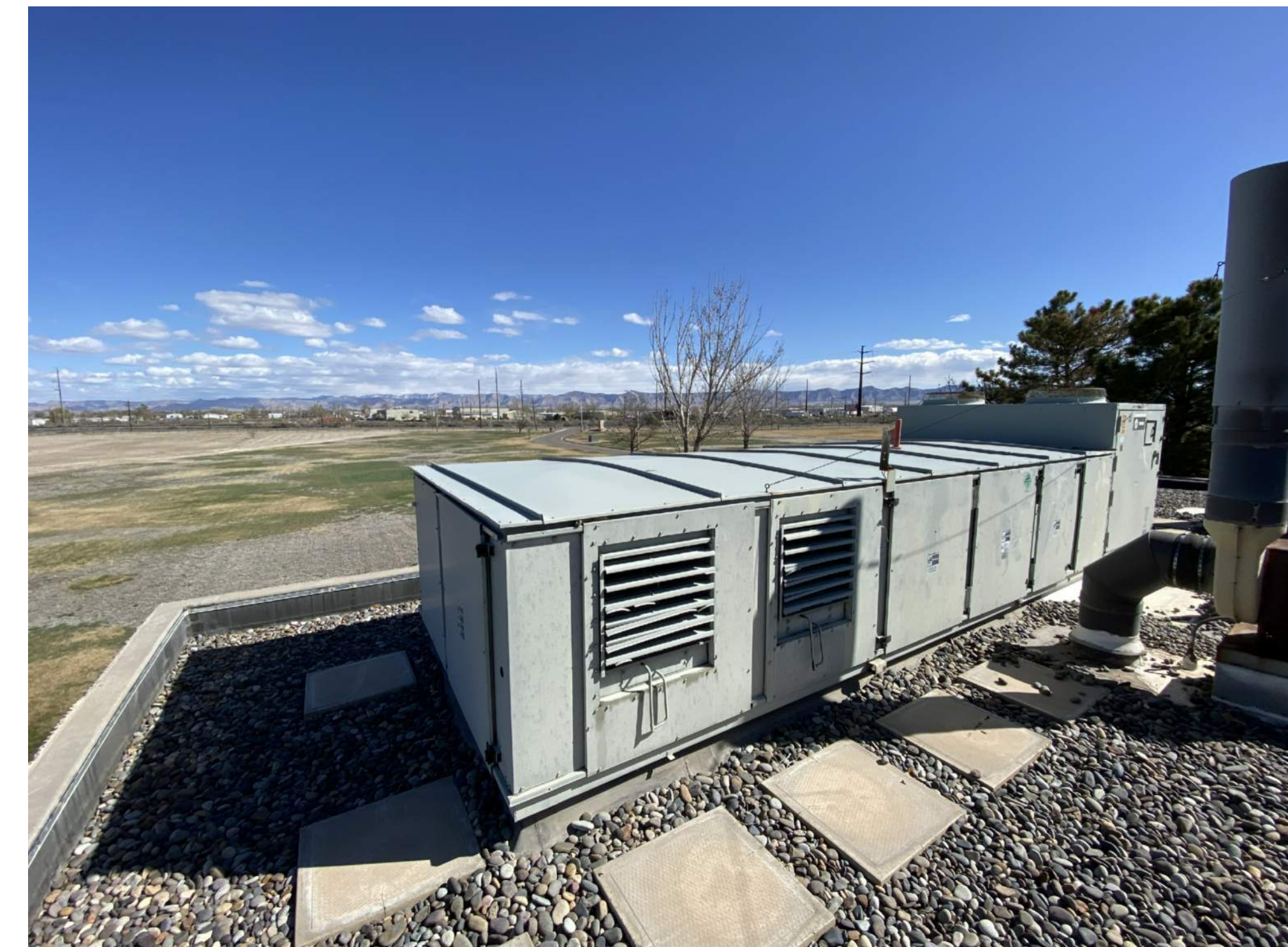
EXISTING LABORATORY TRANE INTELLIPAK
