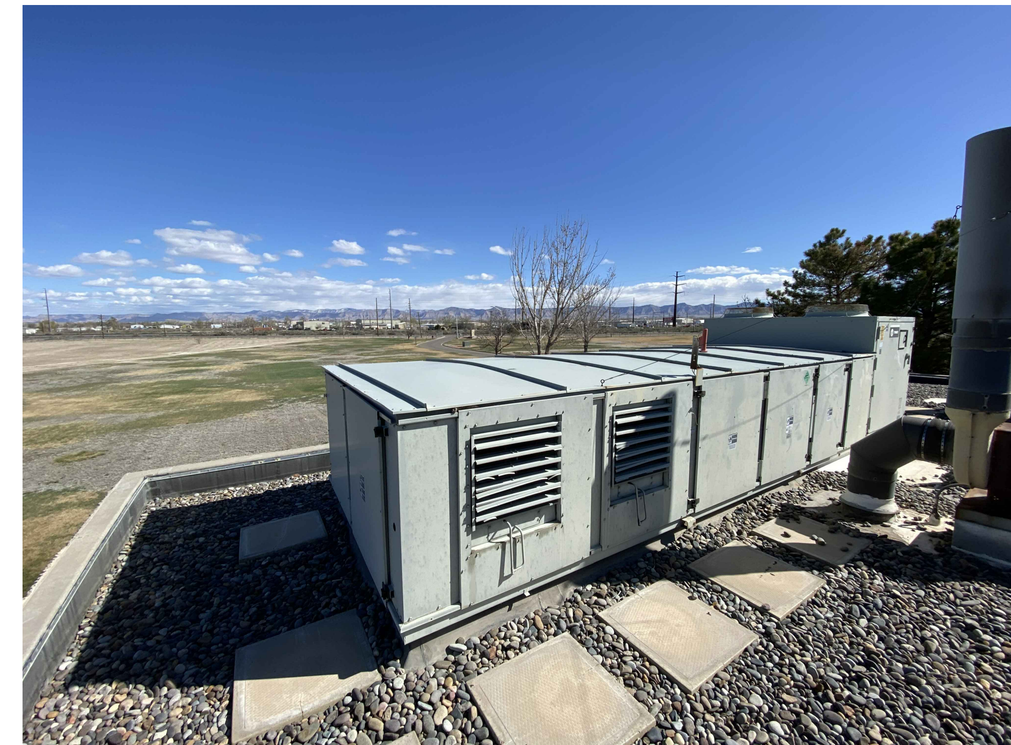
EXISTING LABORATORY TRANE INTELLIPAK
