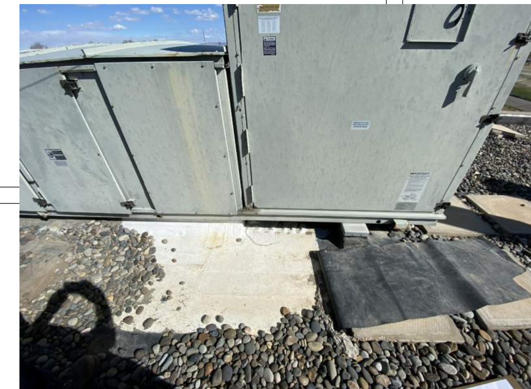
EXISTING LABORATORY TRANE INTELLIPAK THROUGH THE BASE PIPING CONNECTIONS
