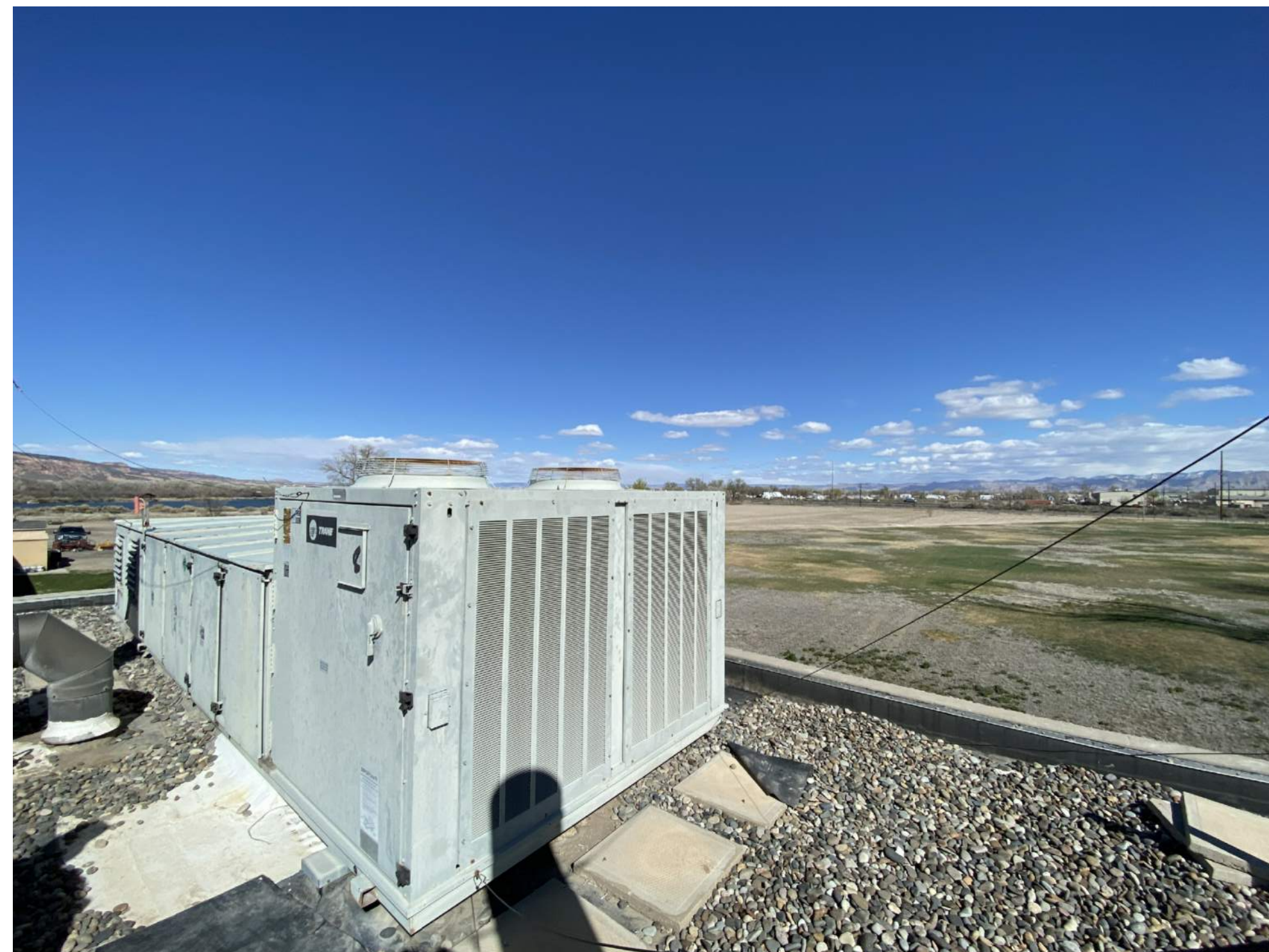
EXISTING LABORATORY TRANE INTELLIPAK
