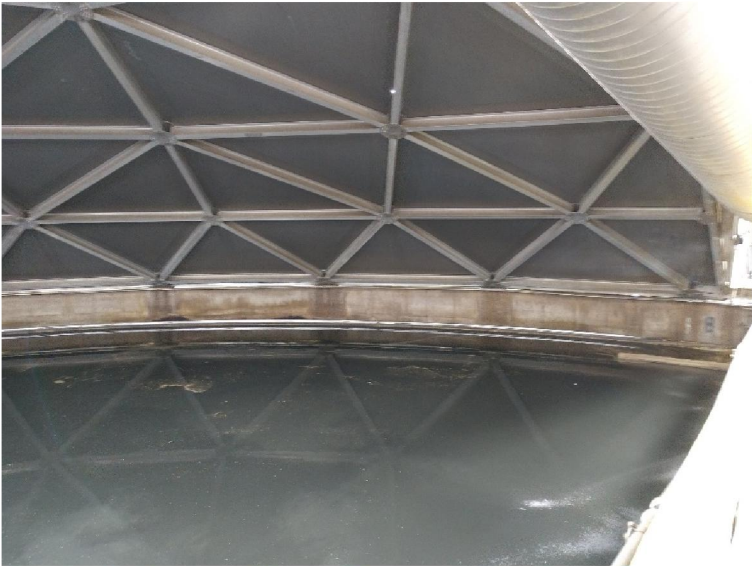
Figure 1 - Interior View of Primary Clarifier
