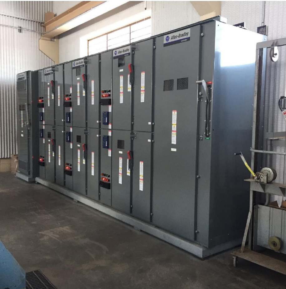
Colorado Springs Utilities - Medium Voltage Motor Control Center
