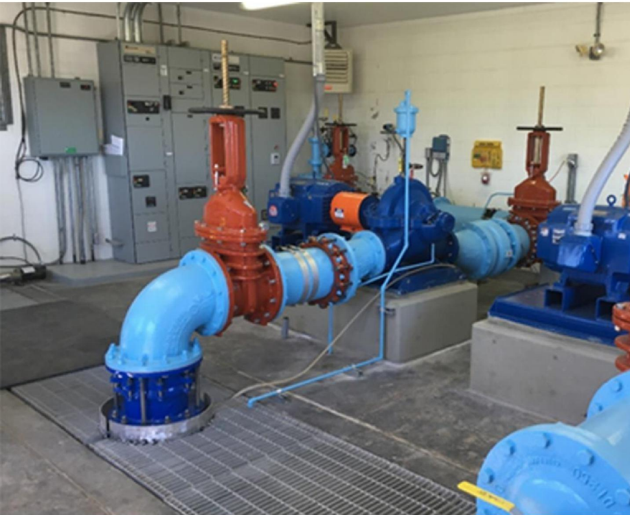
Pump Station #4 Interior
