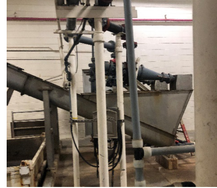
Grit washer compactor.
