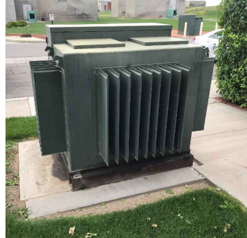
Figure 7.3 Administration Building Transformer
