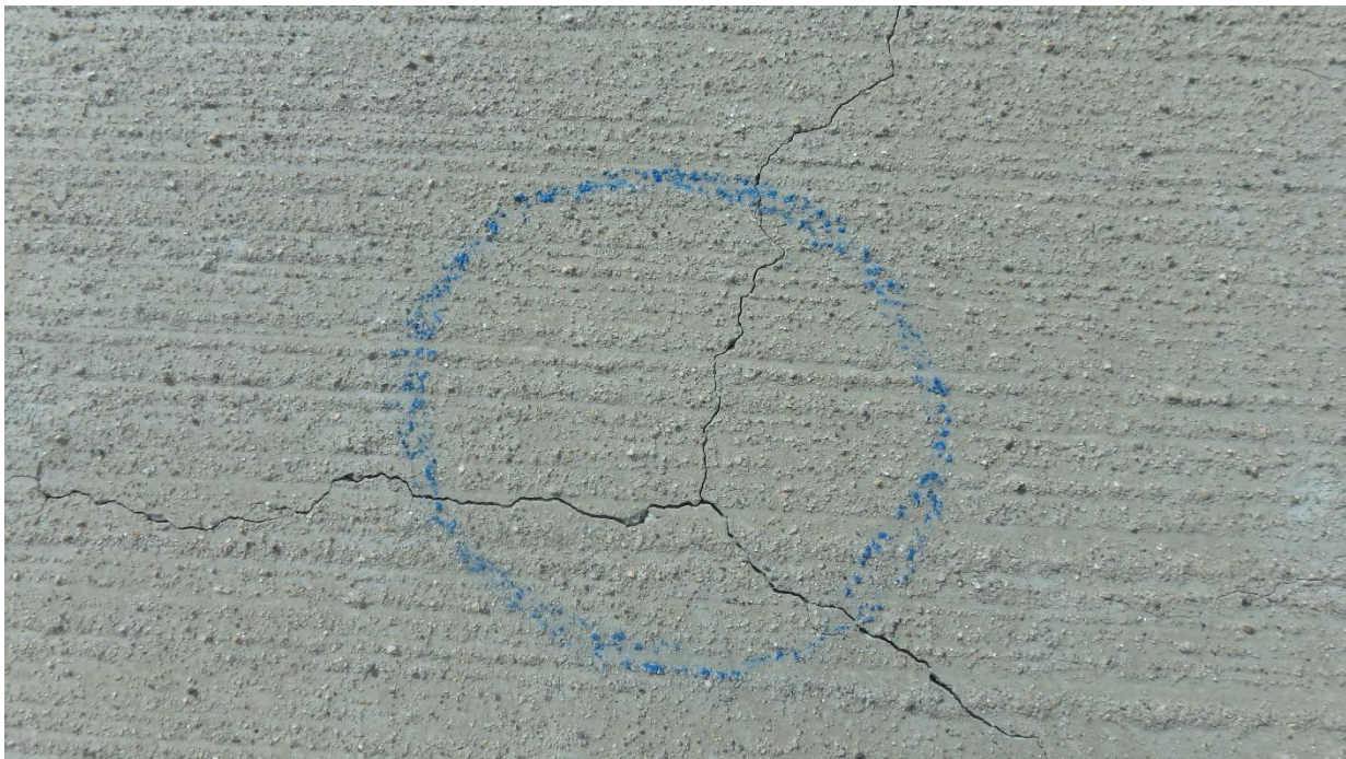
Figure 58. Core sample location at east elevation wall, intersecting multiple surface cracks
