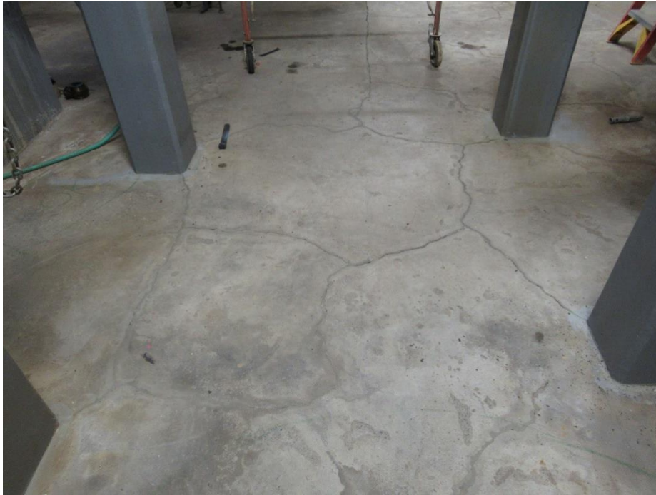
Figure 37. Typical topping slab cracking
