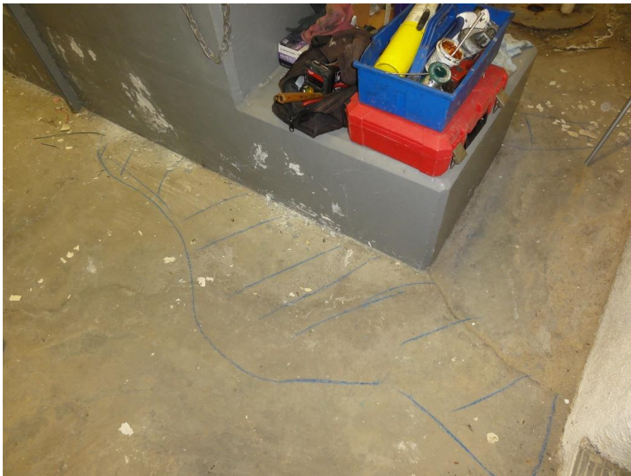
Figure 16. Noted delamination, adjacent to a pipe support pedestal, highlighted in blue
