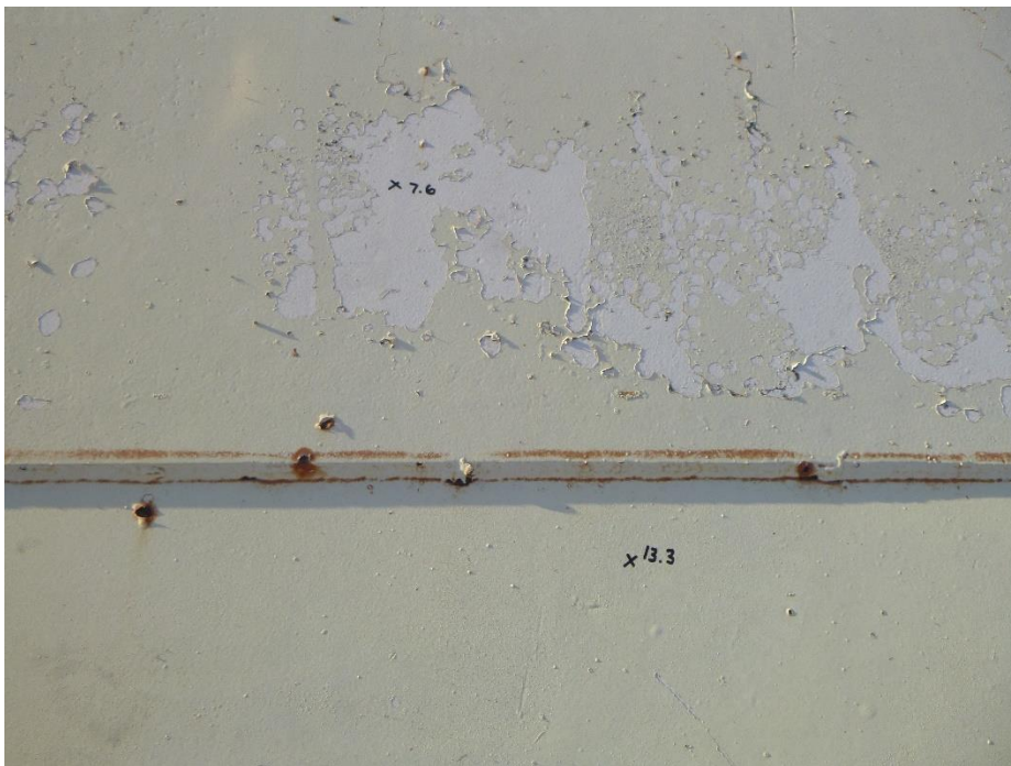
Figure 88. Peeling and flaking coating at south digester lid
