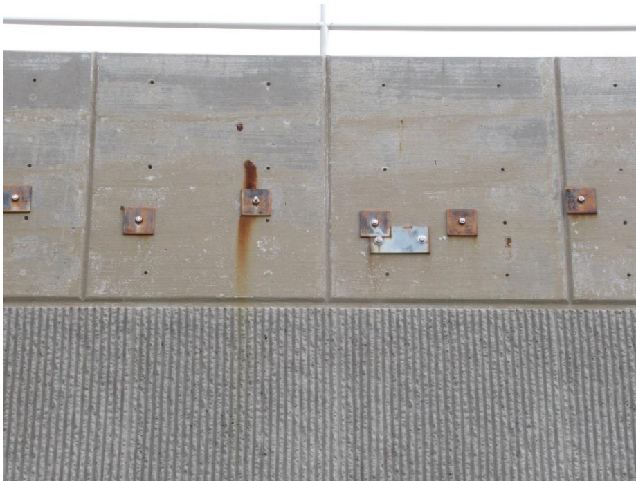
Figure 66. Corrosion of plate washers, as viewed from the exterior of the blending tank walls
