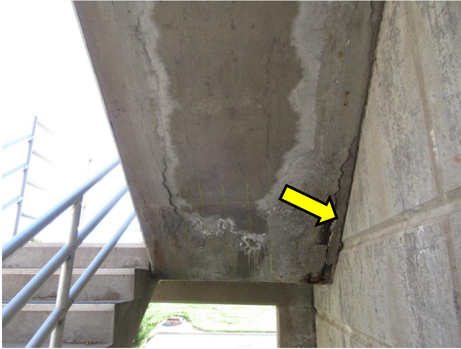
Figure 49. Overall view of the soffit of the ground level stairwell, with noted cracking, spalls, and exposed corroded reinforcing
