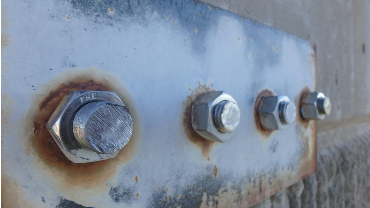
Figure 67. Corrosion of plate washers adjacent to bolt attachments, as viewed from the exterior of the blending tank walls
