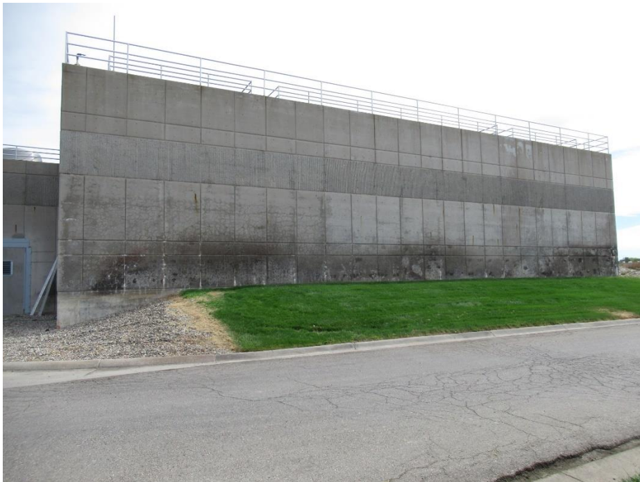
Figure 10. Typical surface staining at base of wall, adjacent to landscaping irrigation
