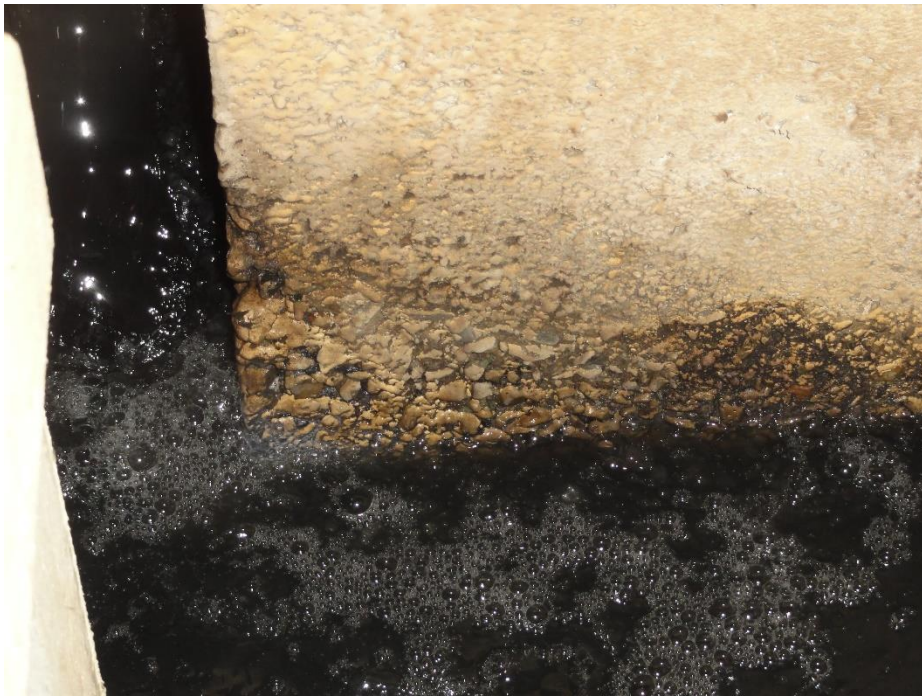
Figure 28. Paste erosion within the scum pit
