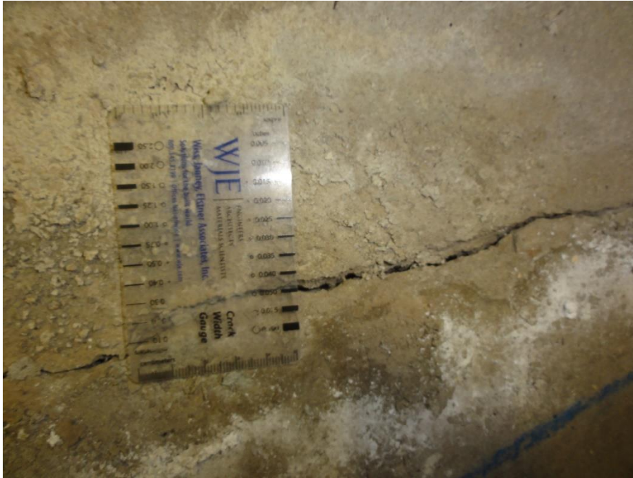
Figure 15. Measurement of a crack at the topping slab of the pump room
