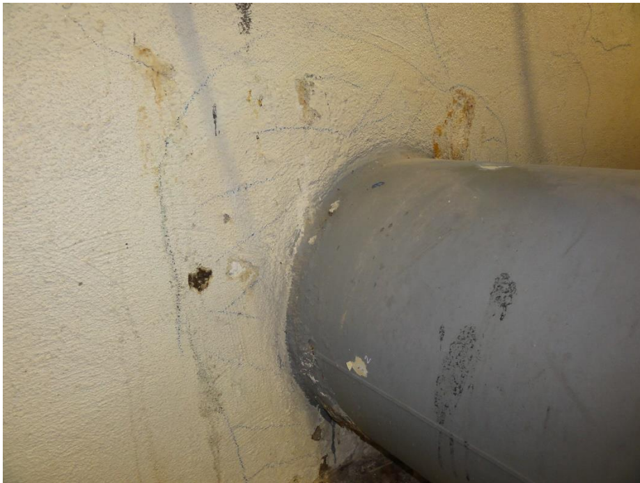
Figure 4. Sounded delaminated coating adjacent to inlet pipe
