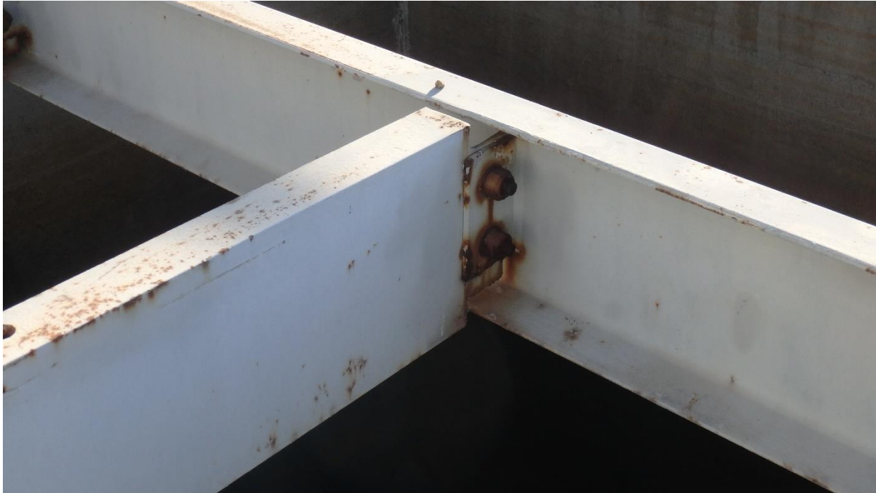
Figure 69. Corrosion on bolted connection for the interior framing support
