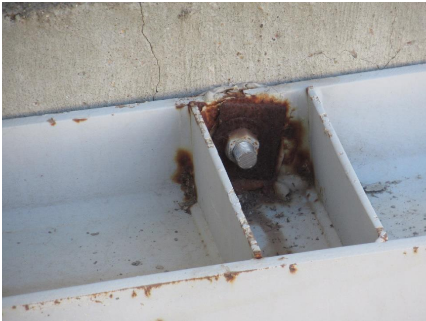
Figure 68. Corrosion of plate washers adjacent to bolt attachments, as viewed from the interior of the blending tank walls
