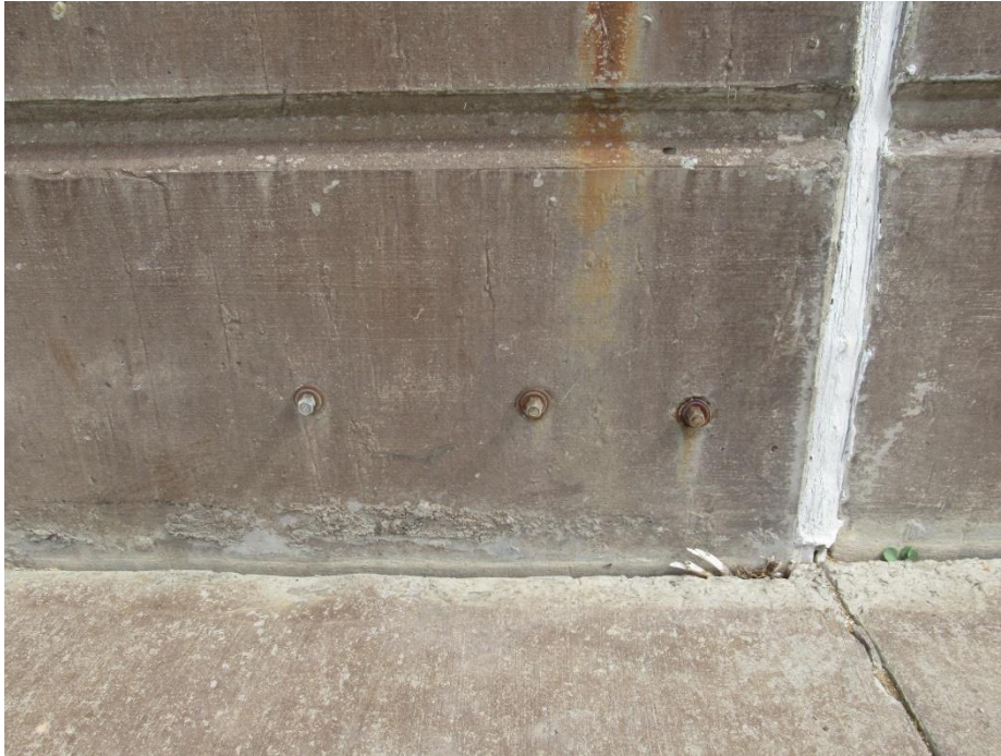
Figure 82. Supplemental attachment bolts at one panel at the south digester
