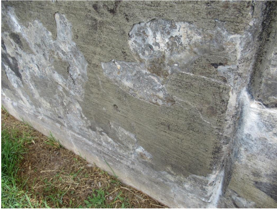
Figure 9. Flaking of surface applied purge coat at Aerobic Digester perimeter wall
