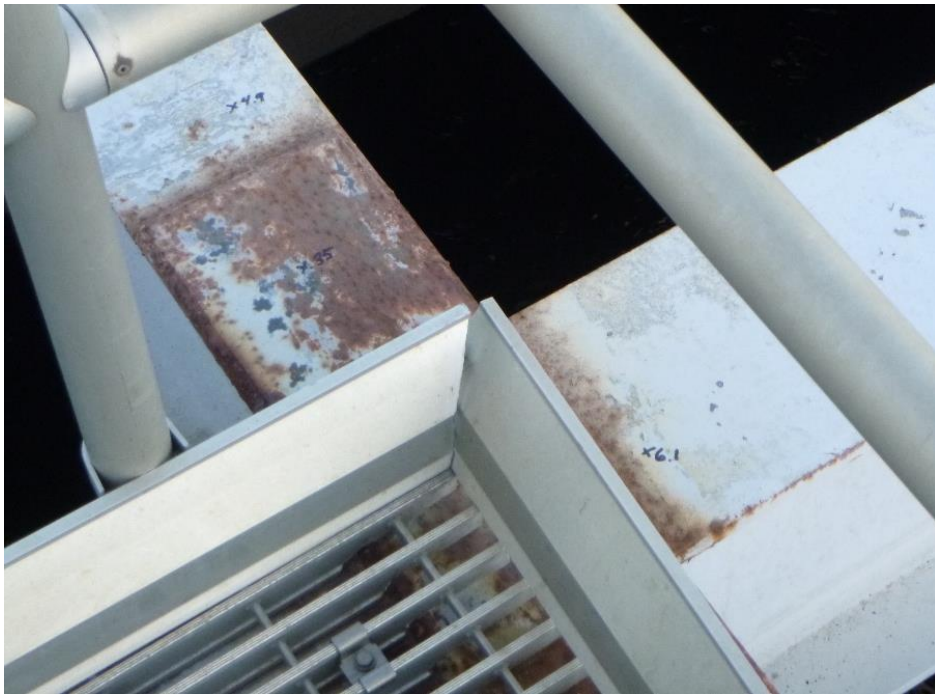
Figure 72. Coating thickness correlated to corrosion distress, note black coating thickness measurements in mils
