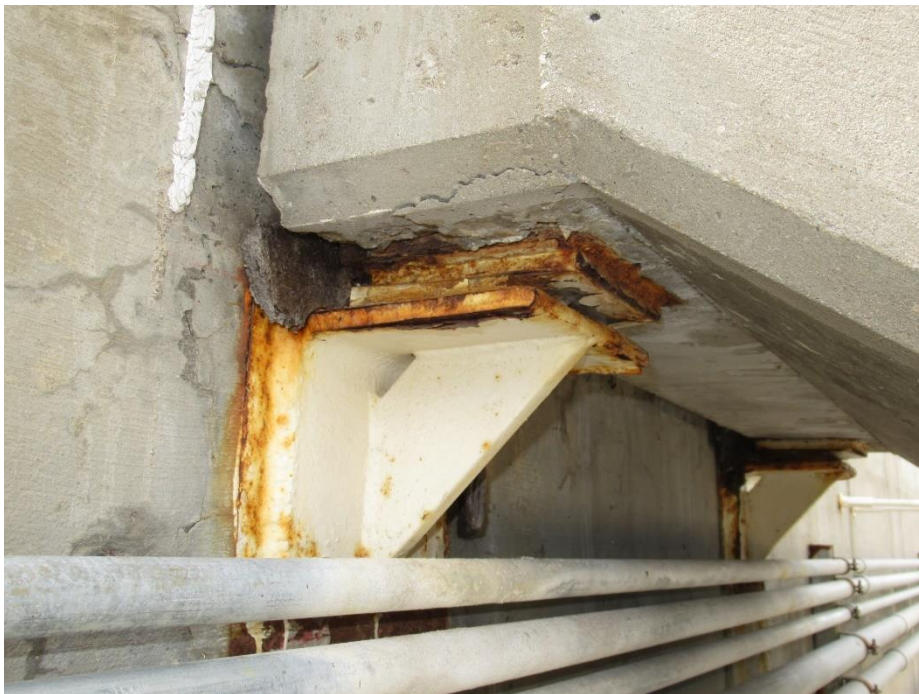
Figure 52. Surface corrosion on the upper support bearing angles and plates for the roof level stairwell
