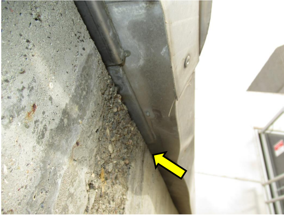
Figure 29. Underside of roof attachment, with a 1-inch wide gap (arrow) between the roof framing and the top surface of the clarifier walls
