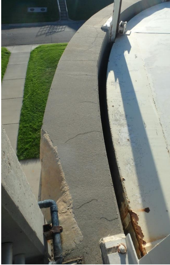
Figure 84. Transverse cracking at the concrete coping cap
