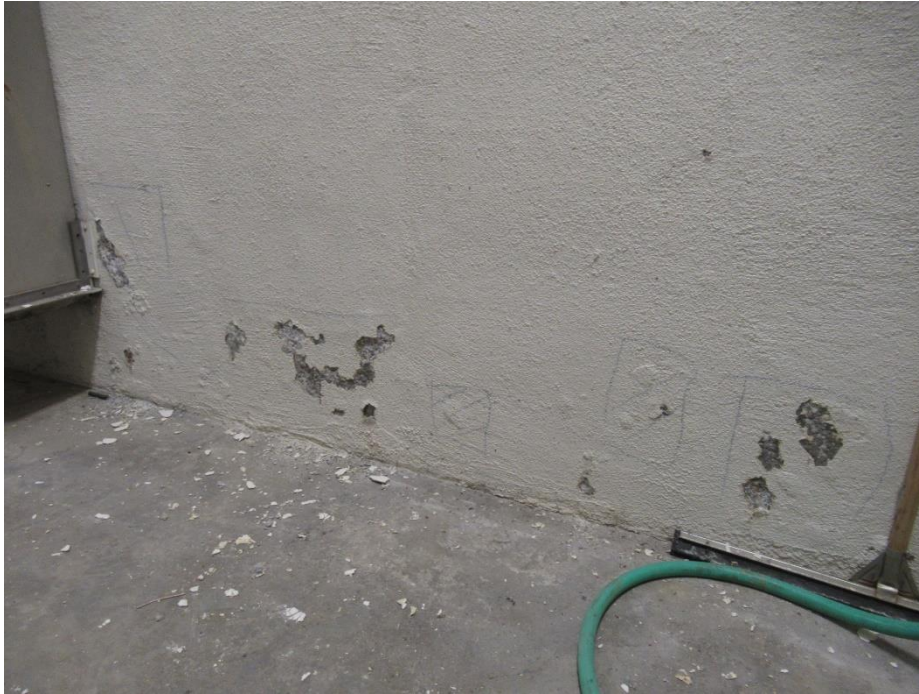
Figure 13. Coating delaminations at the base of the interior walls
