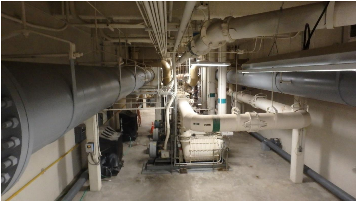
Figure 32. Overall view of the blower room, looking south
