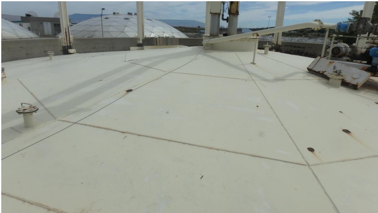
Figure 86. Overall view of the coating on the top surface of the south digester lid
