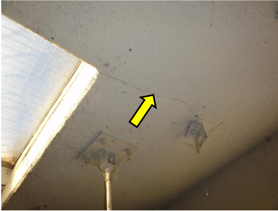
Figure 35. Re-entrant corner cracking at blower room skylight, as observed on the soffit of the ground floor slab
