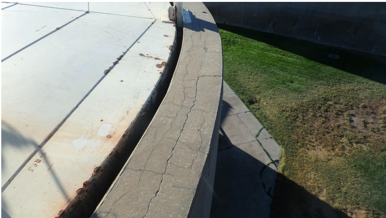
Figure 83. Longitudinal crack at the centerline of the concrete coping cap
