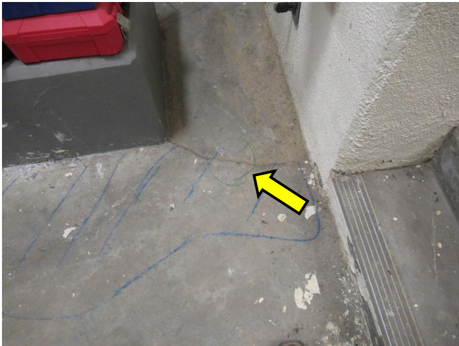
Figure 22. Core location through topping slab crack
