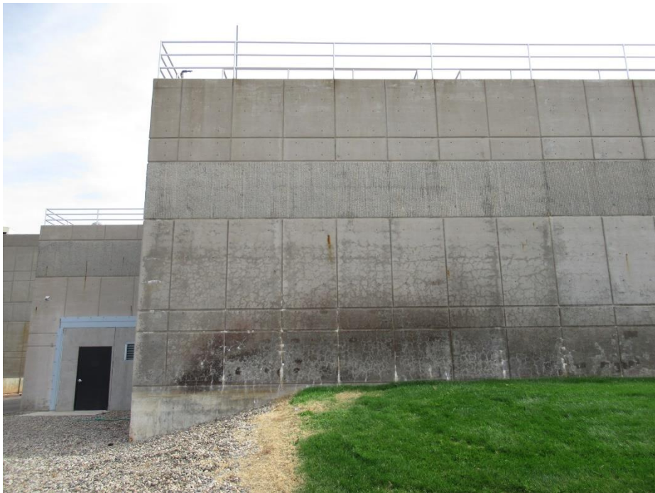
Figure 6. Map patterned cracking at lower half of Aerobic Digester perimeter walls
