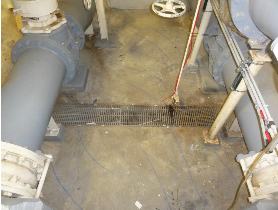
Figure 17. Noted delamination, adjacent to the central trench drain, highlighted in blue
