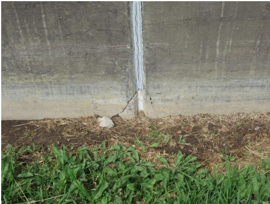
Figure 81. Spalled concrete at lower corner of exterior panel
