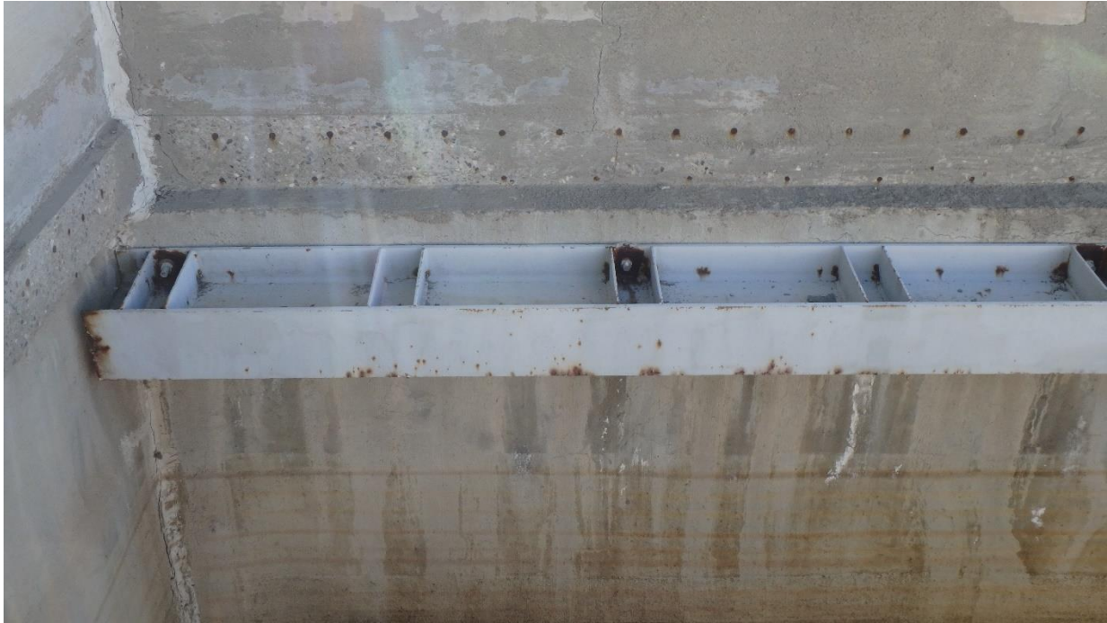
Figure 63. Typical steel framing and attachment at north and west walls of blending tank
