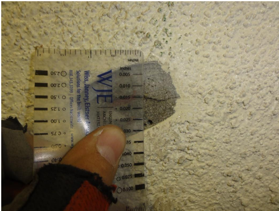
Figure 12. 15 mil crack observed in concrete substrate, that had not yet propagated through the wall coating
