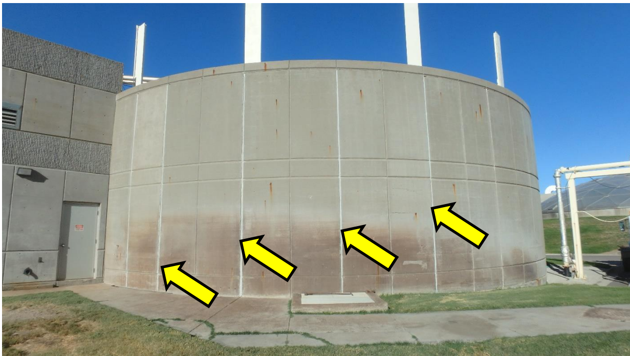
Figure 74. Overall view of the south digester, with exterior panels delineated by sealant joints (arrows)
