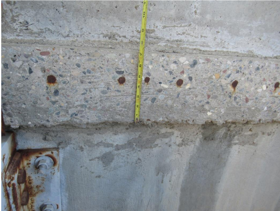
Figure 65. Surface corrosion on previously sawcut reinforcing, which was abandoned when concrete lid/roof was removed
