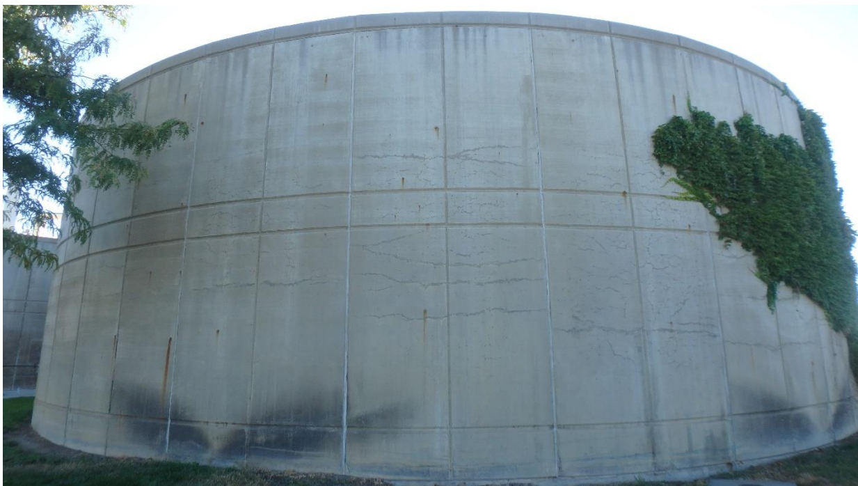
Figure 79. Transverse cracking observed on multiple panels
