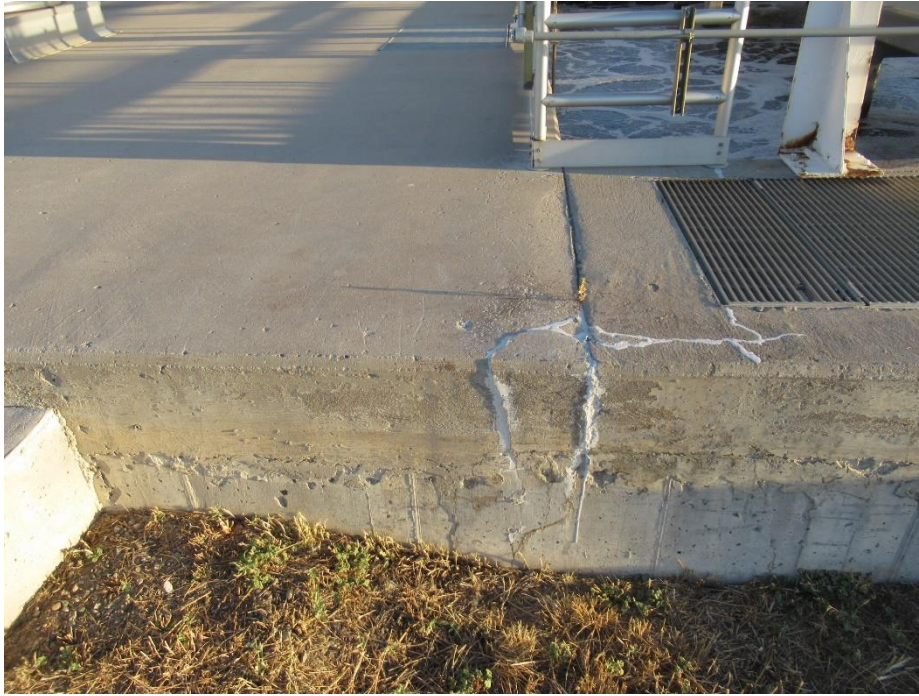
Figure 41. Previously installed sealant at incipient spall location
