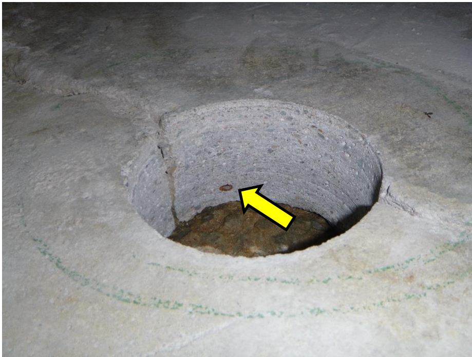
Figure 24. WWR observed near the bottom surface of the extracted core
