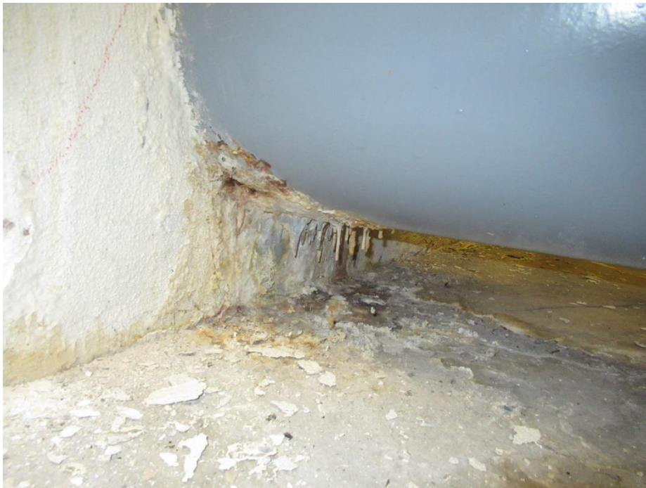
Figure 14. Efflorescence and mineral deposits beneath inlet piping
