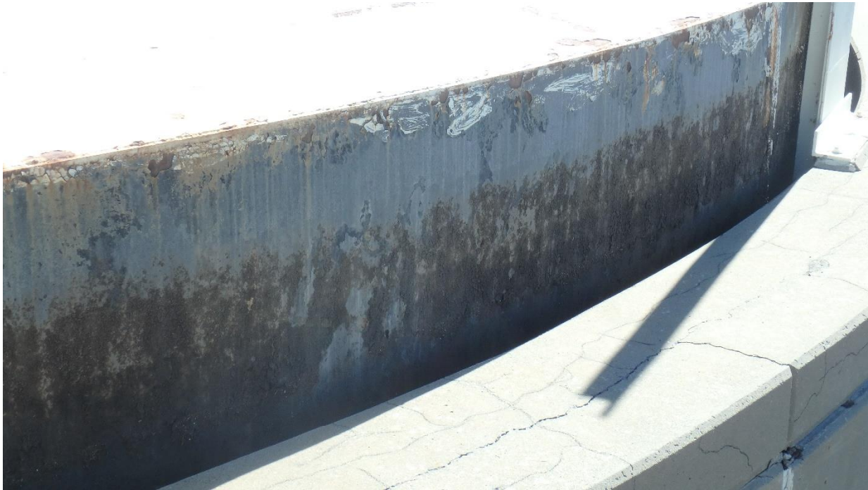
Figure 87. Overall view of the coating on the vertical surface "rim skirt" of the south digester lid
