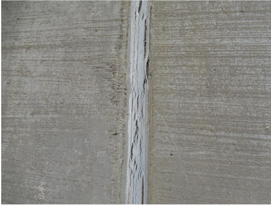
Figure 85. Sealant joint that had failed in both adhesion and cohesion
