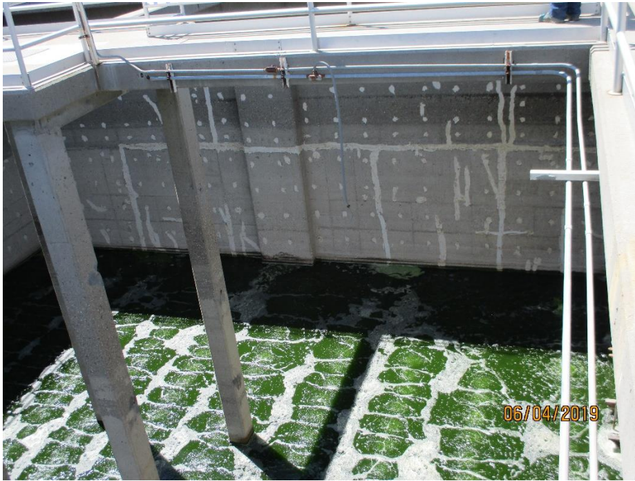
Figure 45. Previous crack repair attempt at the digester basin walls
