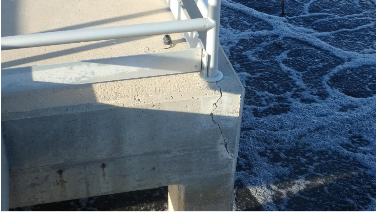
Figure 39. Incipient spall at guardrail post embed
