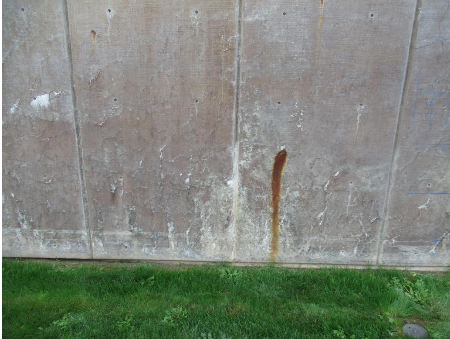
Figure 71. Noted efflorescence at panel reveal joint
