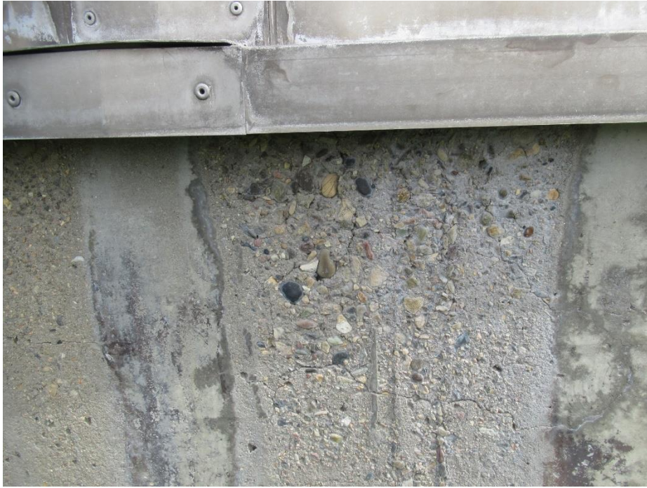
Figure 31. Paste erosion at exterior of clarifier walls
