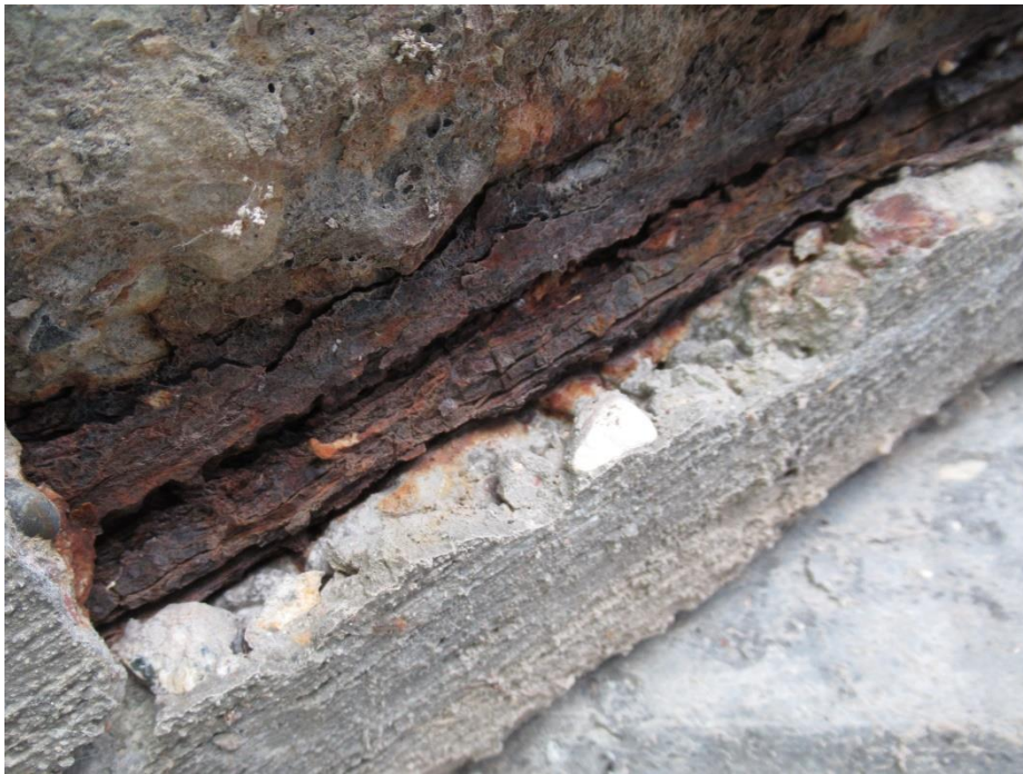
Figure 50. Up-close view of exposed corroded reinforcing at the soffit of the ground level stairs
