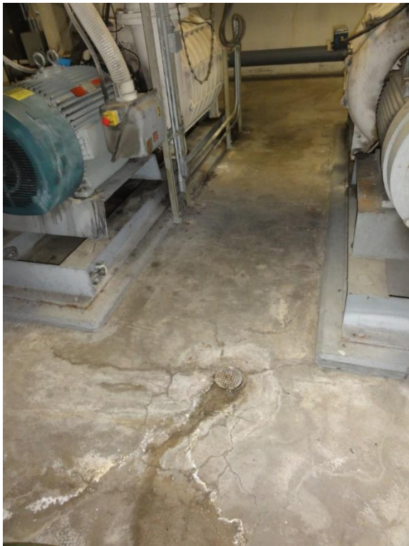
Figure 38. Evidence of ponding water at existing floor drain
