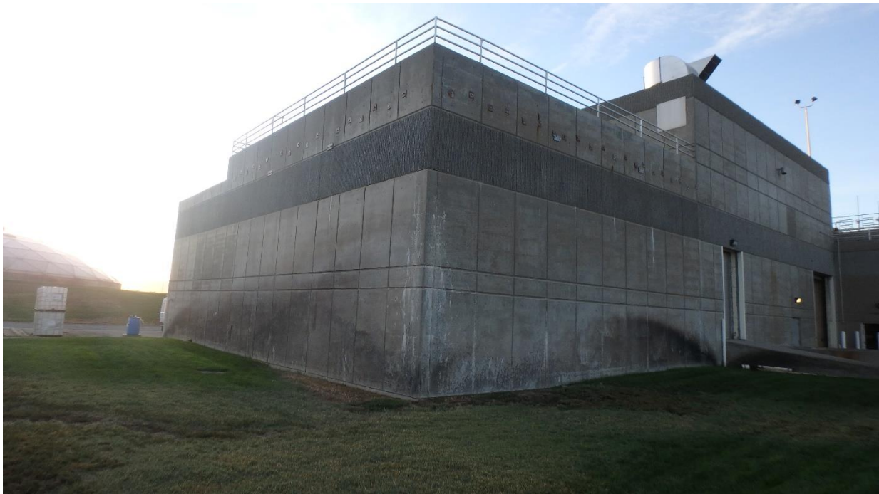
Figure 70. Noted efflorescence and staining at northwest corner of blending tank
