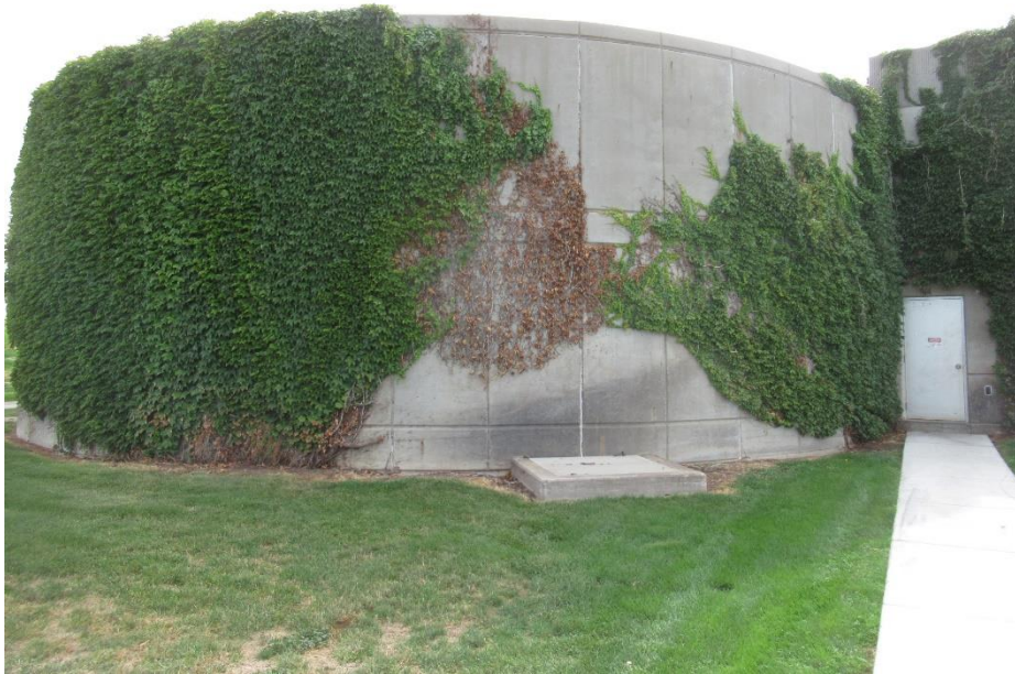
Figure 76. Plant growth on north digester exterior
