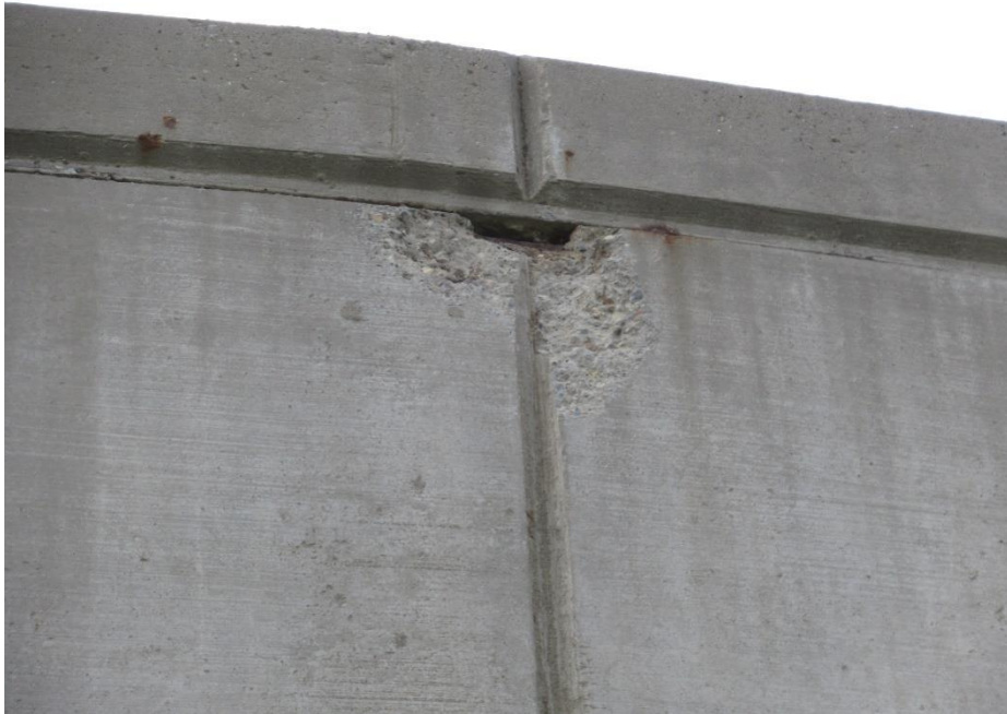
Figure 80. Spalled concrete at upper corner of exterior panel
