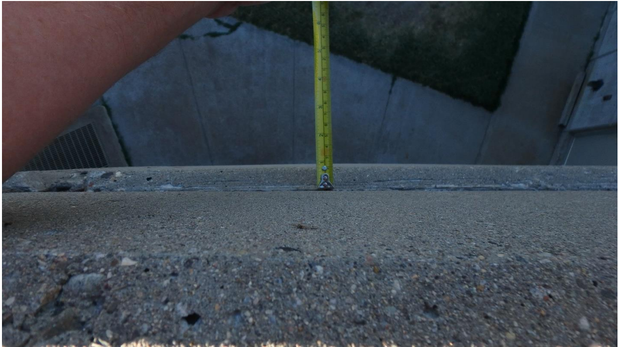
Figure 78. Panel top edge that had bowed approximately 1-inch outboard from concrete coping cap
