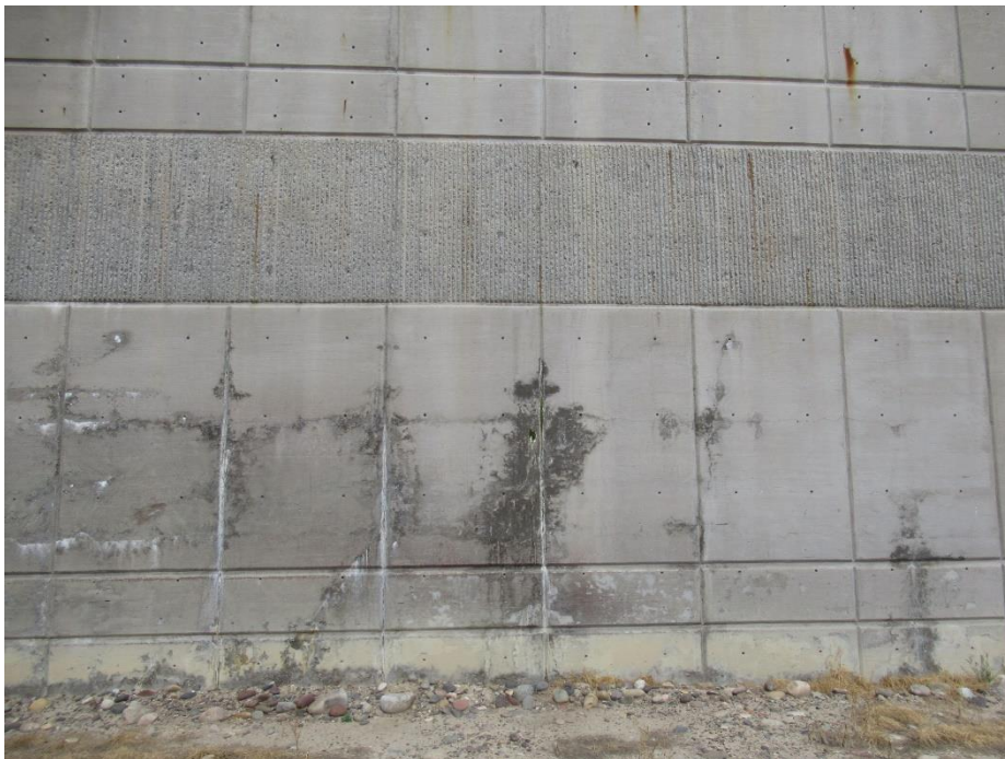
Figure 46. Evidence of moisture intrusion and efflorescence staining at reveal joints
