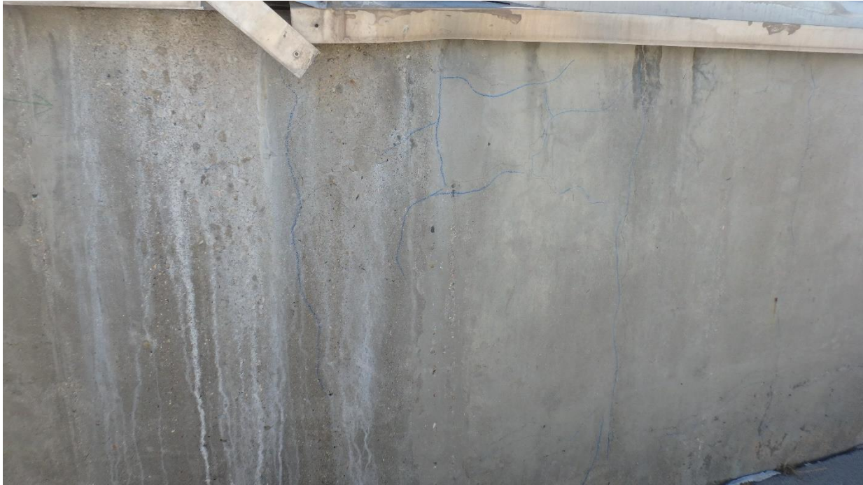
Figure 5. Map patterned cracking at exterior of Primary Clarifier walls
