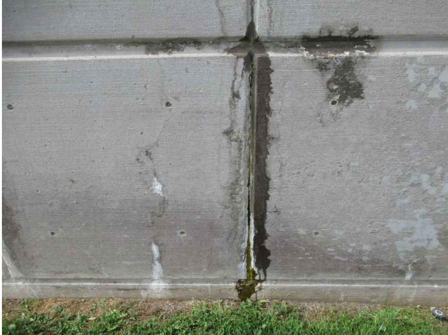
Figure 48. Actively leaking crack within reveal joint
