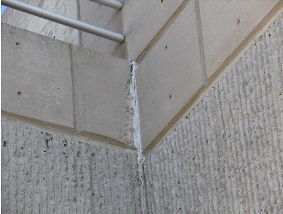
Figure 53. Failed sealant joint between Aerobic Digester and Sludge Processing Unit
