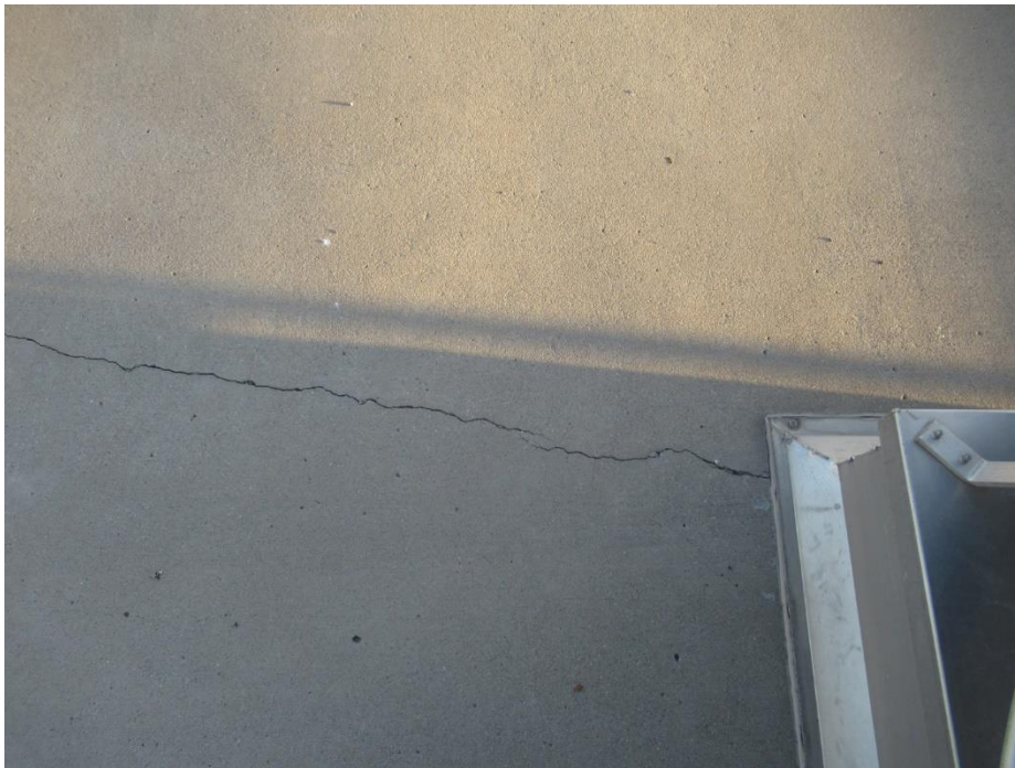
Figure 36. Re-entrant corner cracking at blower room skylight, as observed on the top surface of the ground floor slab
