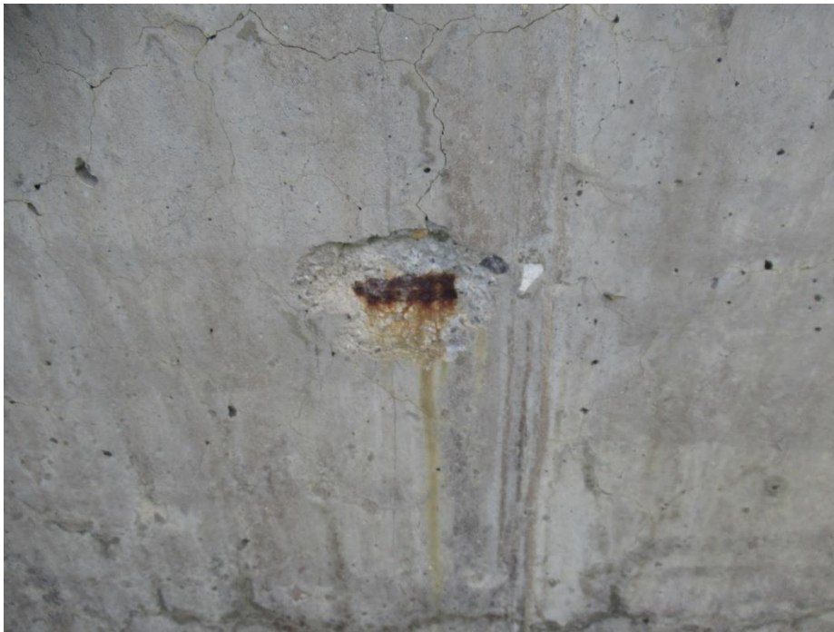
Figure 30. Isolated exposed and corroded reinforcing bar
