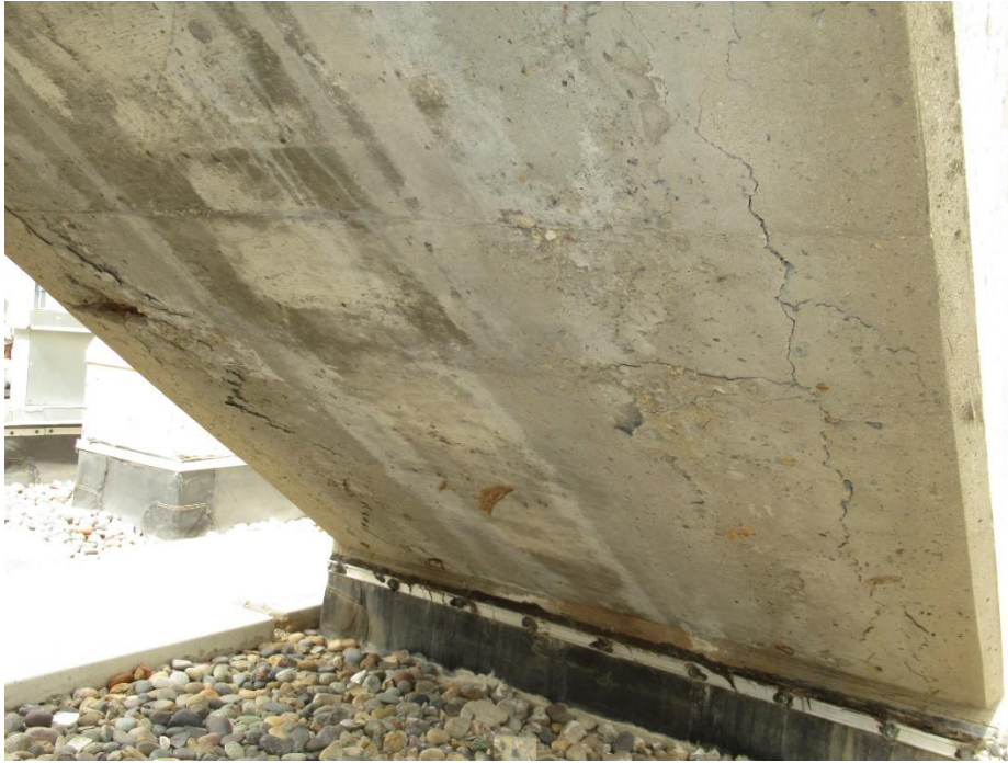
Figure 51. Overall view of the soffit of the roof level stairwell, with noted cracking and spalls
