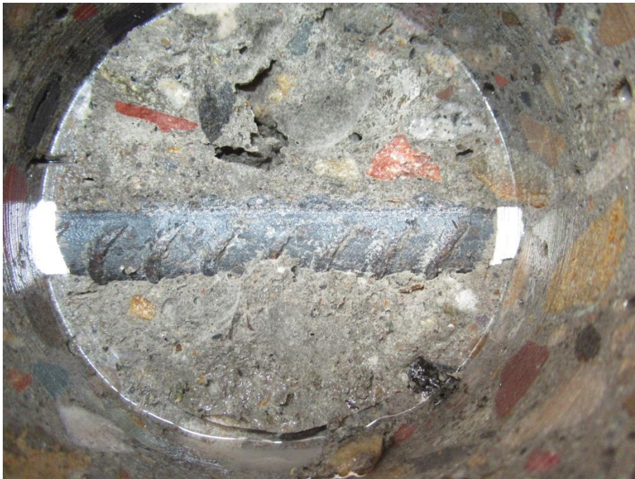
Figure 60. Exposed embedded reinforcing bar, with little to no surface corrosion present
