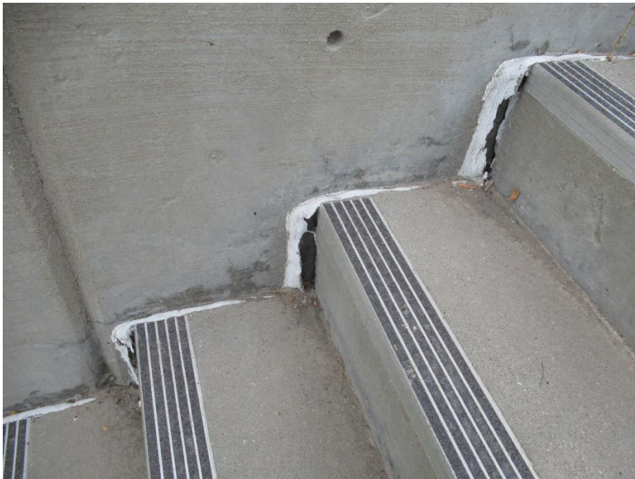
Figure 54. Sealant joint between the ground level stairs and the adjacent building face that had failed and was no longer in contact with both substrate surfaces
