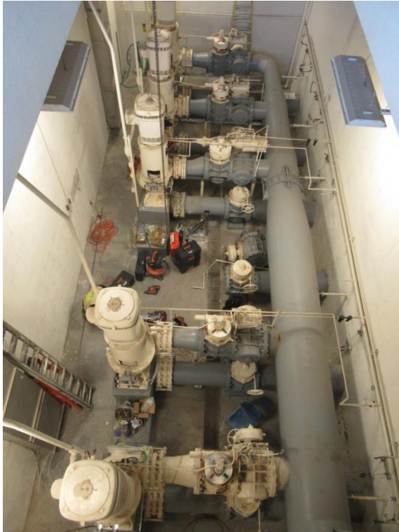
Figure 11. Overall view of the pump slab room, as viewed from the ground floor slab
