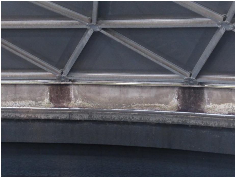
Figure 26. Moisture staining present beneath roof attachment locations
