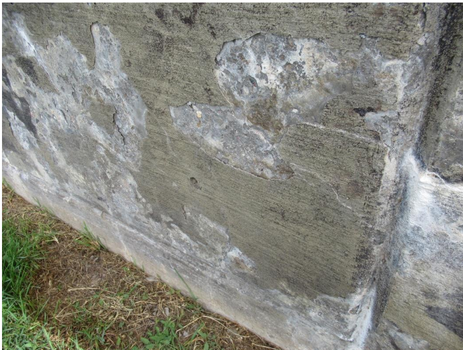
Figure 63. Flaking of surface applied skim coat
