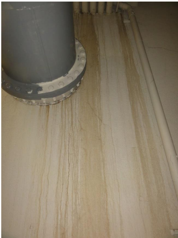
Figure 45. Staining below through-wall penetrations at the north elevation foundation wall
