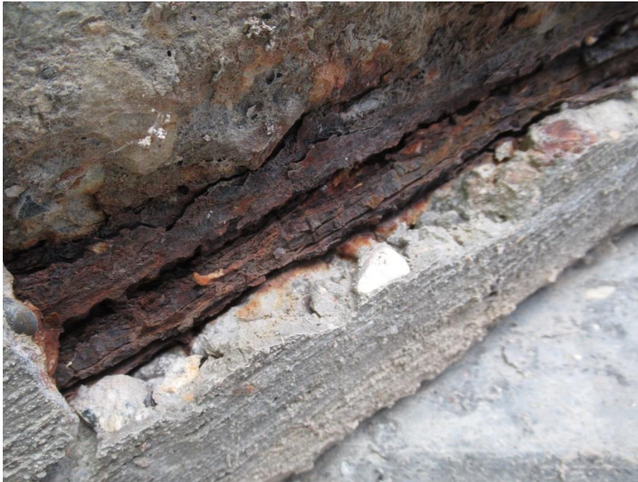
Figure 66. Up-close view of exposed corroded reinforcing at the soffit of the ground level stairs
