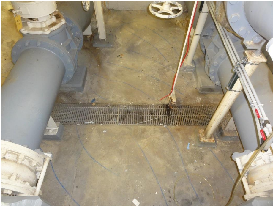
Figure 4. Noted delamination, adjacent to the central trench drain, highlighted in blue
