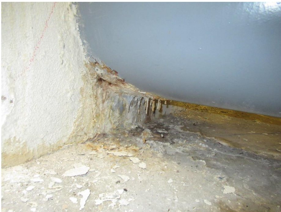
Figure 14. Efflorescence and mineral deposits beneath inlet piping
