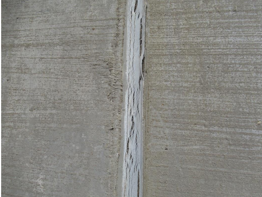
Figure 102. Sealant joint that had failed in both adhesion and cohesion
