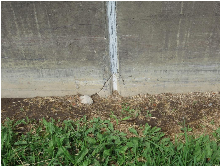
Figure 98. Spalled concrete at lower corner of exterior panel
