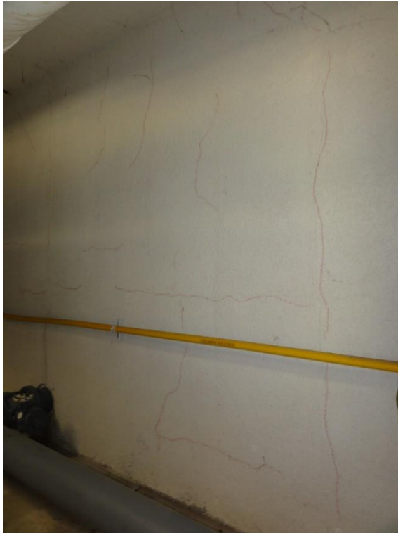
Figure 42. Interior cracking, observed on the north elevation foundation wall (traced in red)
