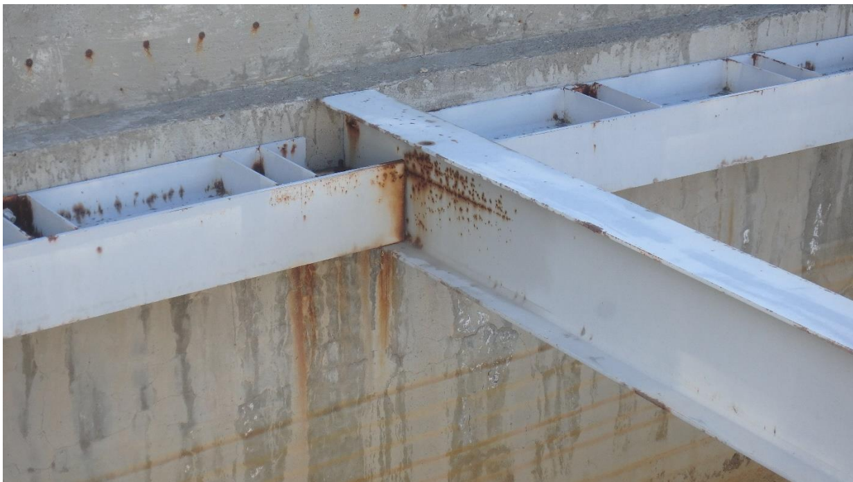
Figure 85. Surface corrosion on coated framing members
