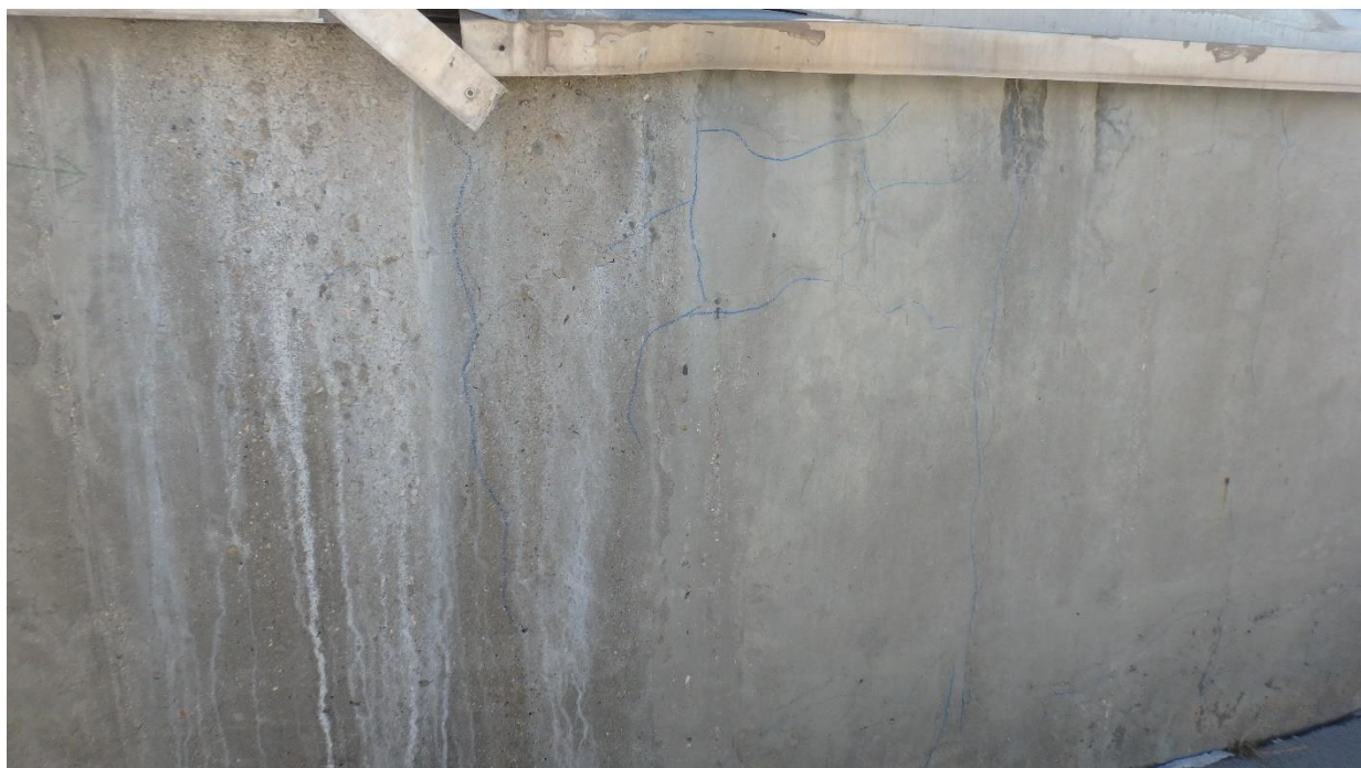
Figure 31. Map patterned cracking at exterior of clarifier walls
