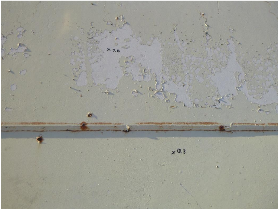
Figure 108. Flaking of coating at south digester lid
