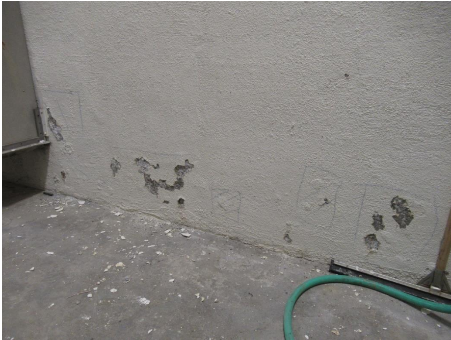
Figure 13. Coating delaminations at the base of the interior walls, note also concrete surface distress where coating was removed
