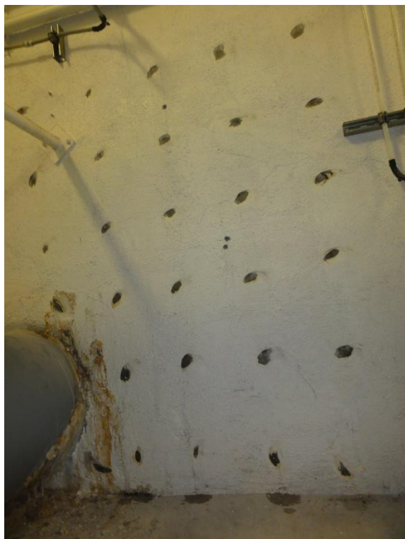
Figure 20. Corrosion Potential measurements on south wall of raw sewage pump station
