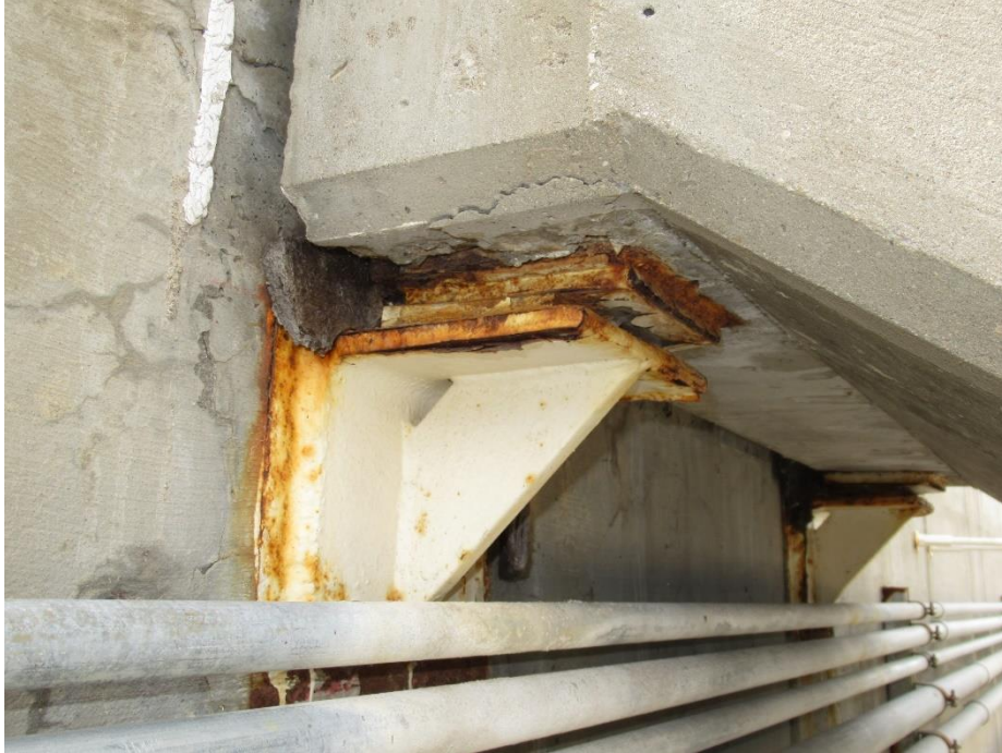
Figure 70. Surface corrosion on the upper support bearing angles and plates for the roof level stairwell
