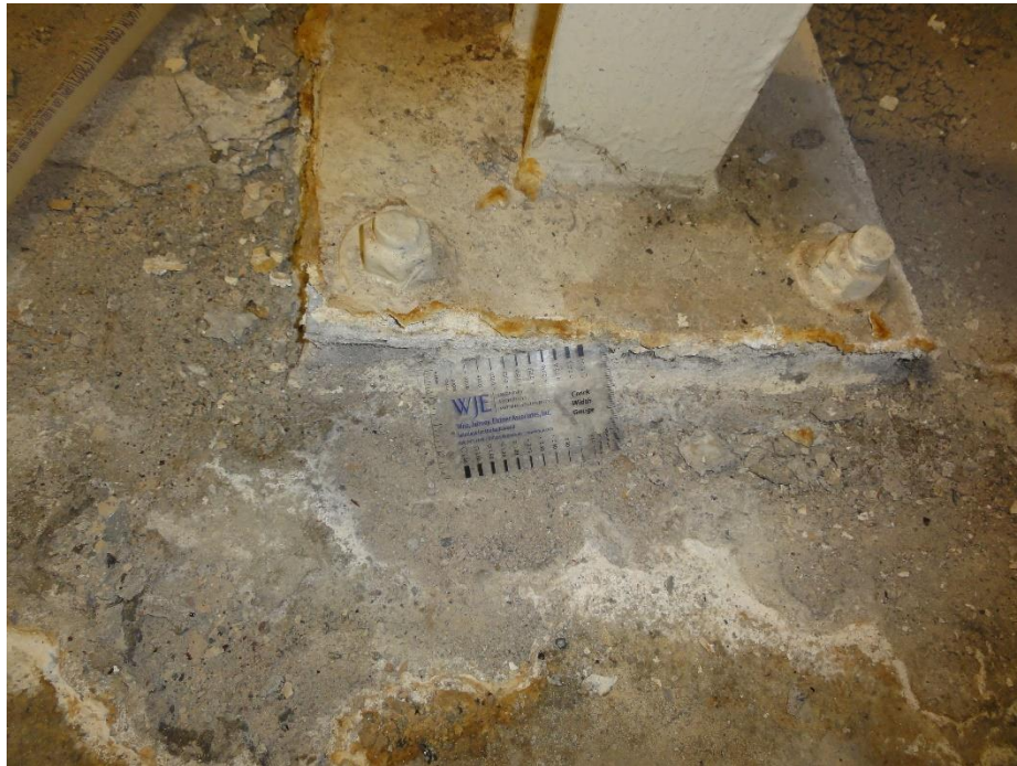
Figure 5. Observed paste erosion at piping element support
