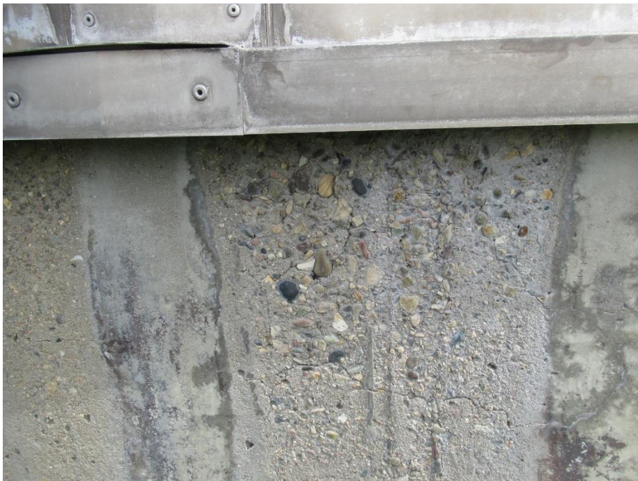
Figure 33. Paste erosion at exterior of clarifier walls at attachment node
