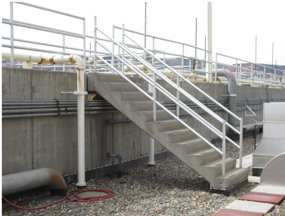
Figure 56. Stairwell leading to Aerobic Digester catwalks
