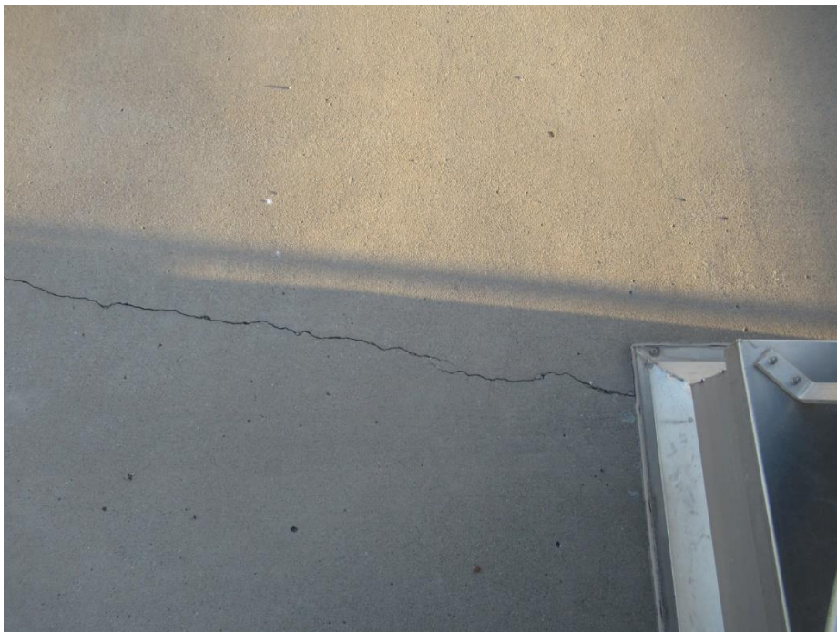
Figure 47. Re-entrant corner cracking at blower room skylight, as observed on the top surface of the ground floor slab
