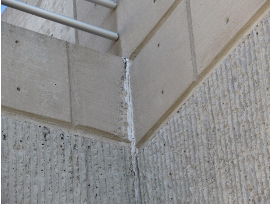
Figure 64. Failed sealant joint between Aerobic Digester and Sludge Processing Unit
