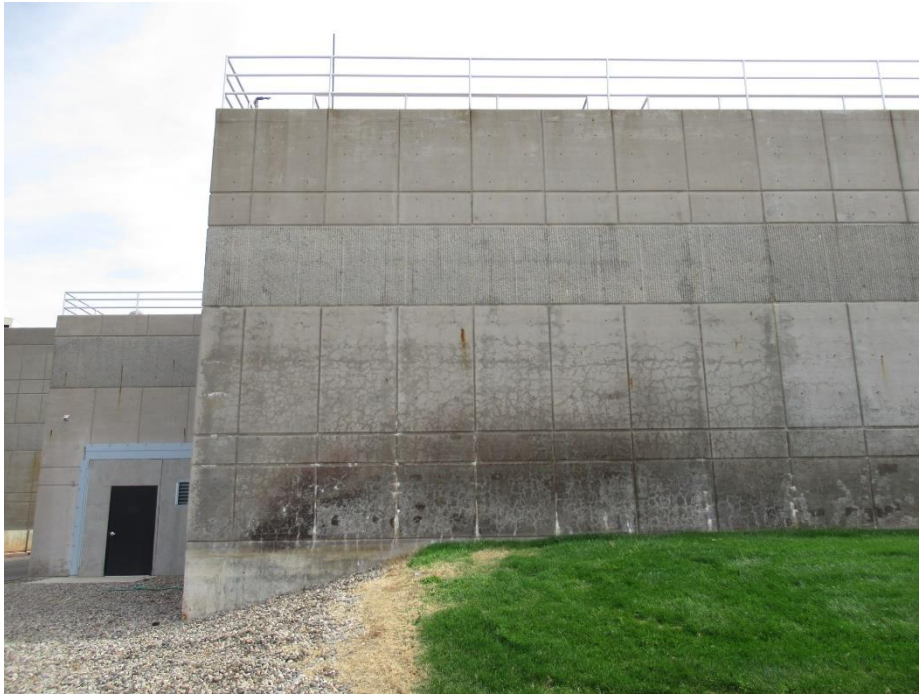
Figure 58. Map patterned cracking at lower half of perimeter walls
