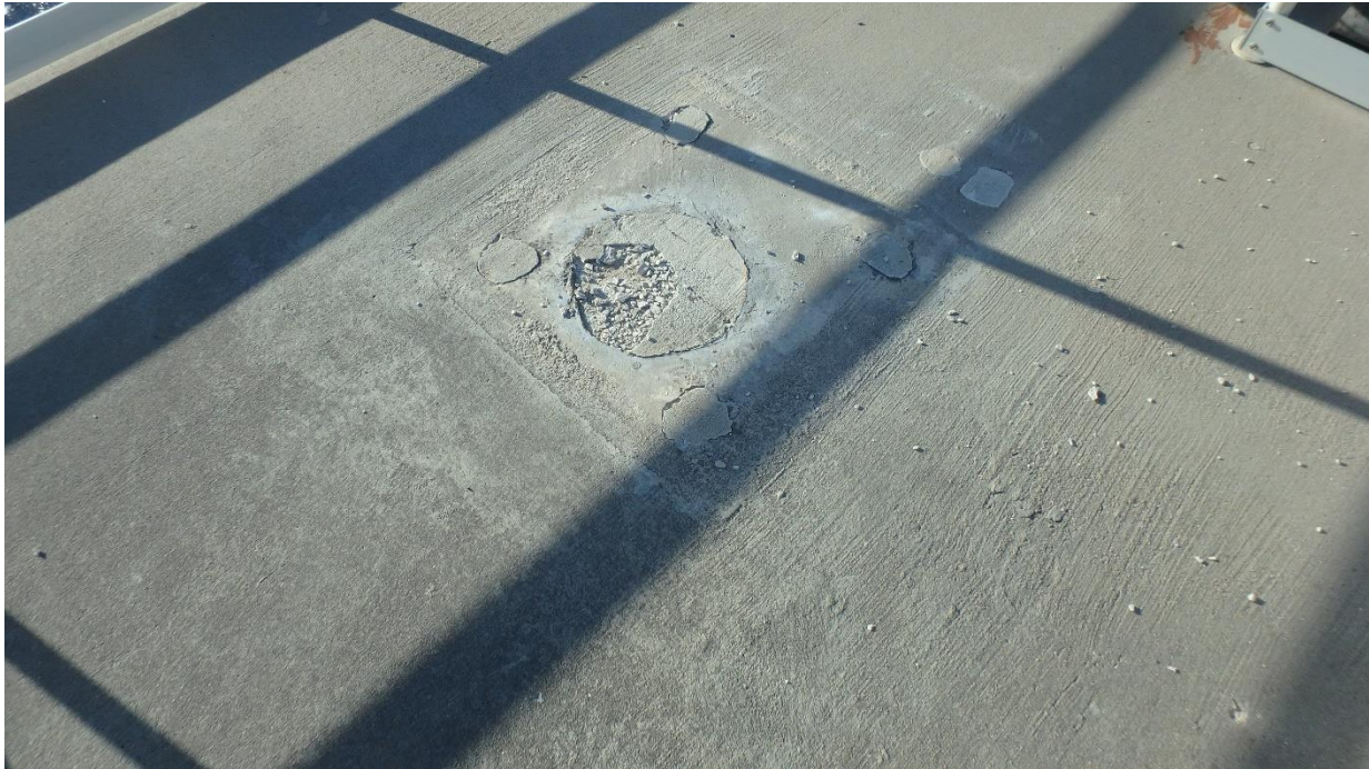
Figure 50. Distressed concrete surface at location of previously removed equipment attachment
