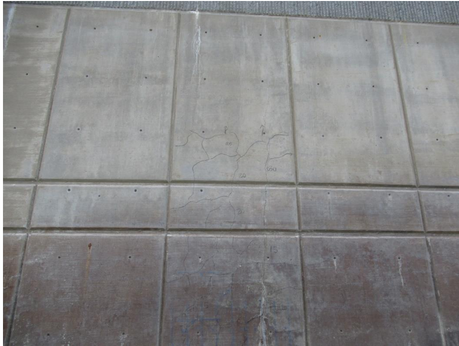
Figure 80. Map patterned cracking at lower portion of exterior walls
