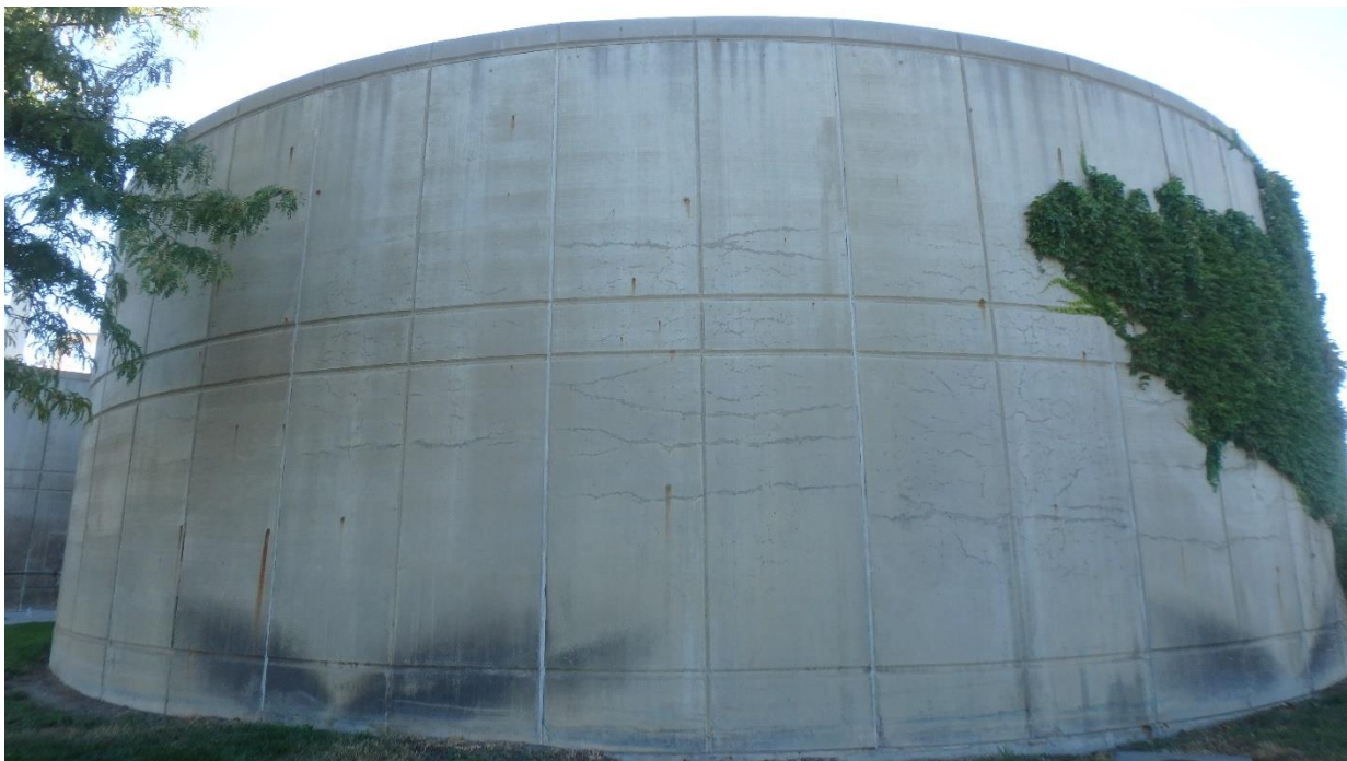
Figure 96. Transverse cracking observed on multiple panels
