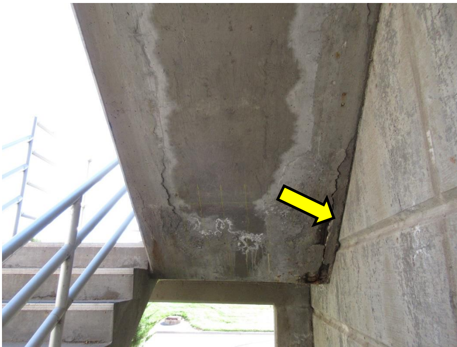
Figure 65. Overall view of the soffit of the ground level stairwell, with noted cracking, spalls, and exposed corroded reinforcing
