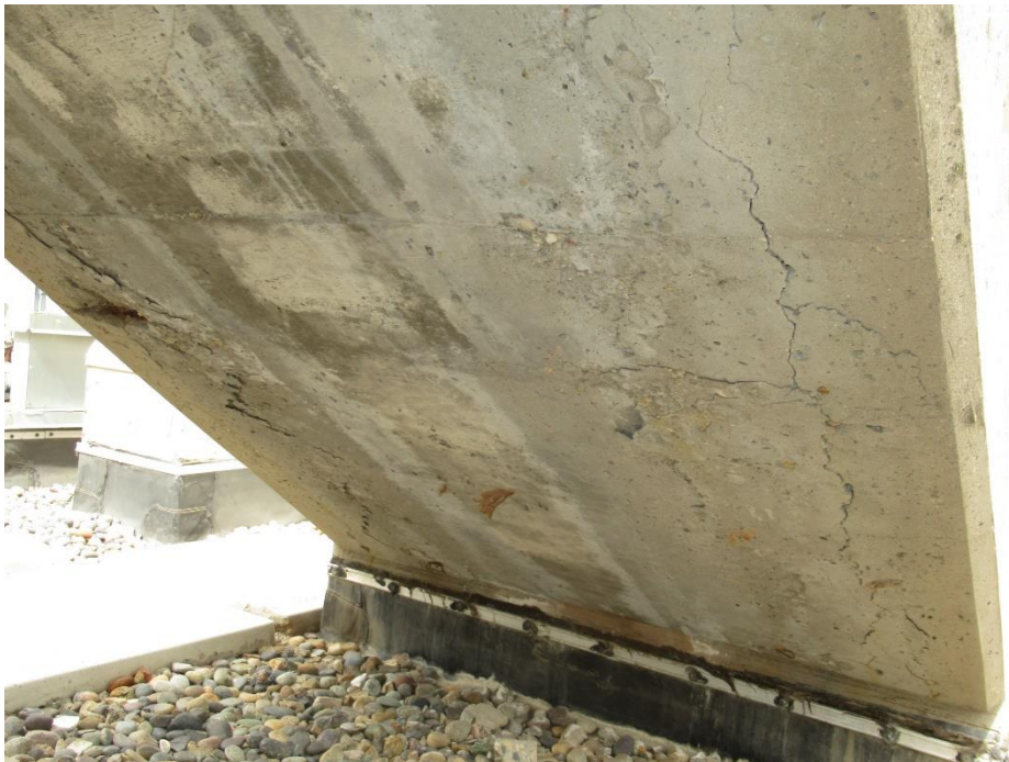
Figure 69. Overall view of the soffit of the roof level stairwell, with noted cracking and spalls
