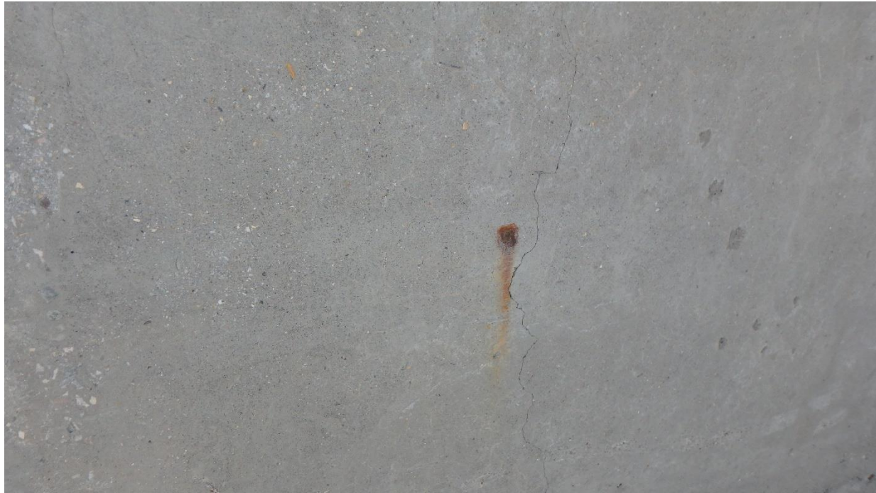
Figure 34. Typical and isolated corrosion staining at aggregate particles
