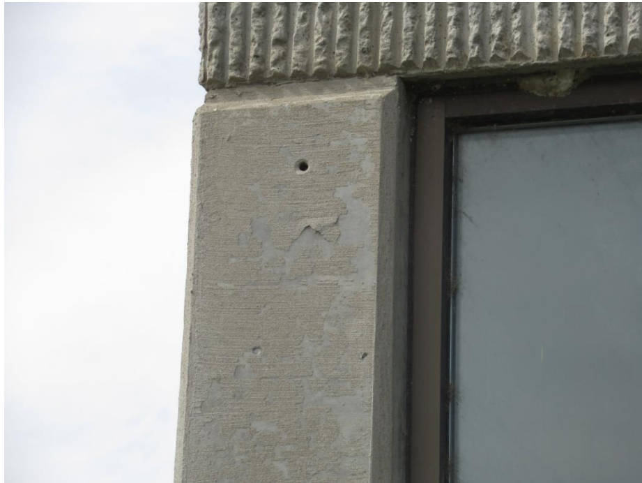
Figure 17. Isolated flaking of surface applied skim coat
