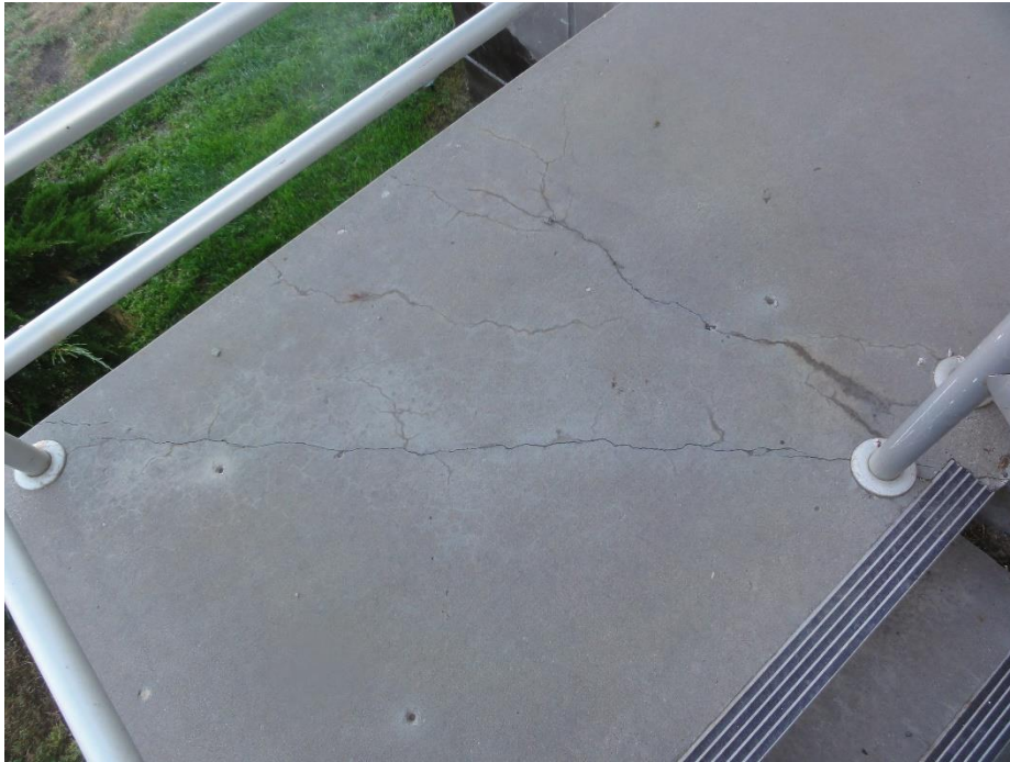
Figure 68. Cracking at ground level stair intermediate landing
