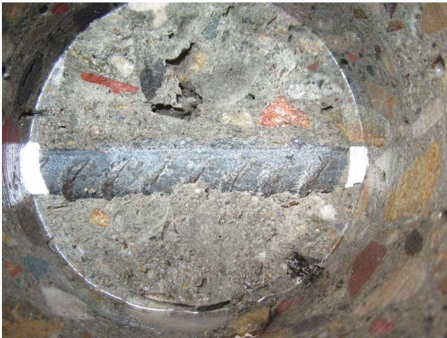
Figure 77. Exposed embedded reinforcing bar, with little to no surface corrosion present
