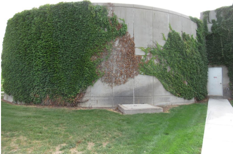
Figure 95. Plant overgrowth on north digester exterior
