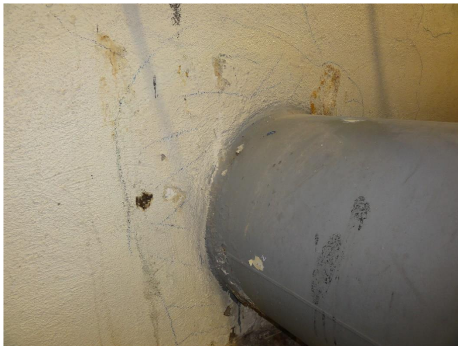
Figure 12. Sounded coating delamination adjacent to inlet pipe, noted in blue
