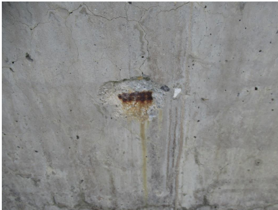
Figure 35. Isolated exposed and corroded reinforcing bar
