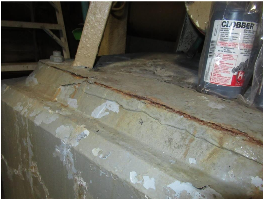
Figure 41. Isolated corrosion on pipe support pedestal framing plate
