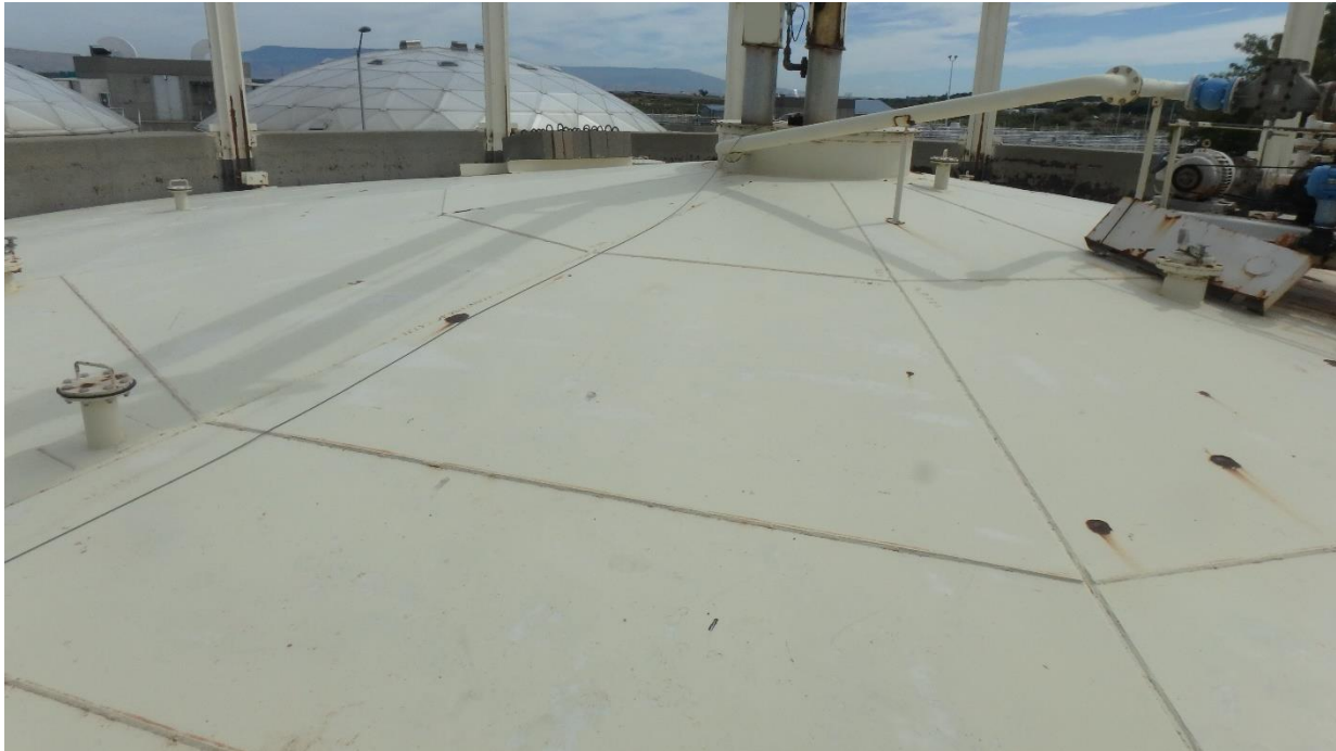
Figure 106. Overall view of the coating on the top surface of the south digester lid
