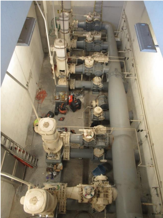
Figure 1. Overall view of the pump slab room, as viewed from the ground floor slab above
