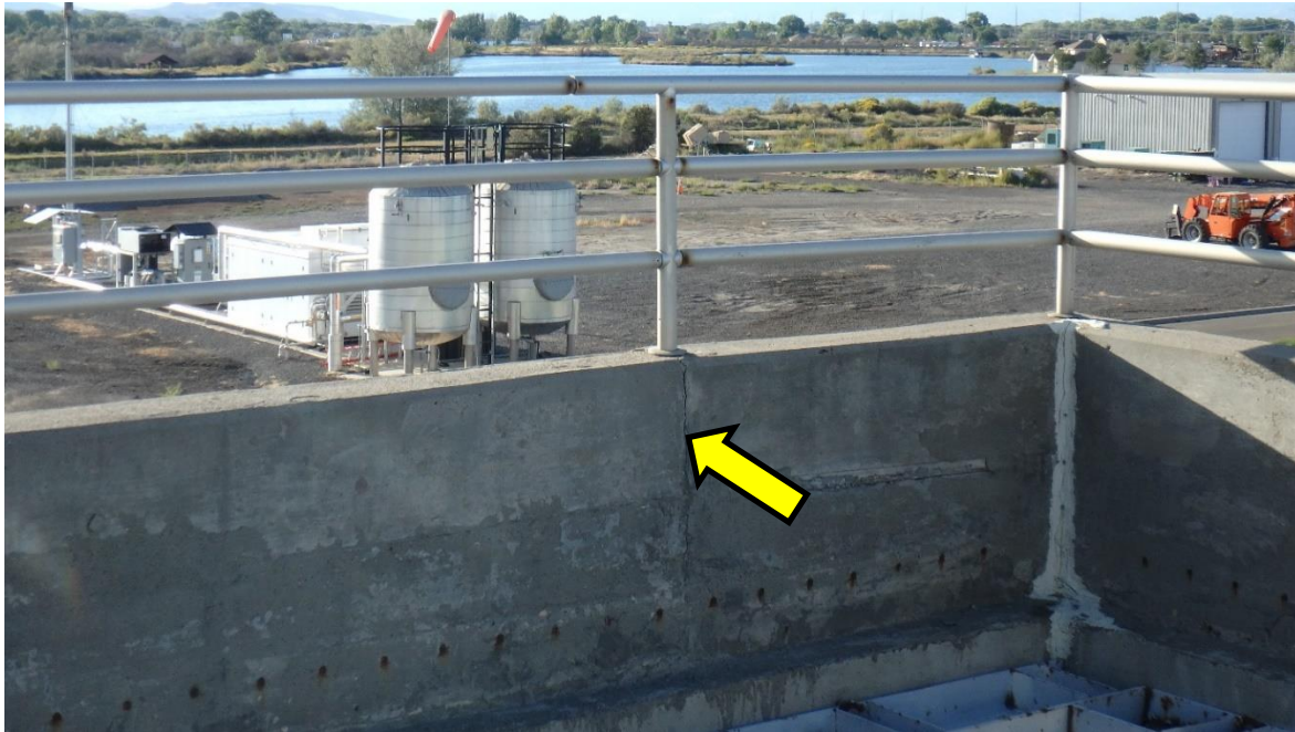
Figure 88. Vertical cracking on interior face of exterior wall, aligning with the guardrail post above
