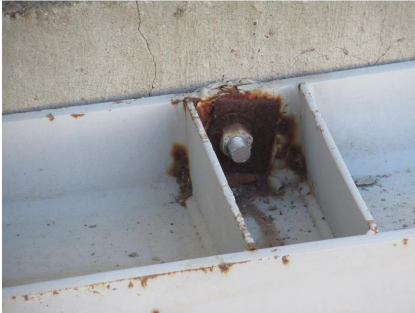
Figure 84. Corrosion of plate washers adjacent to bolt attachments, as viewed from the interior of the blending tank walls
