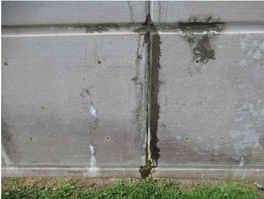
Figure 62. Actively leaking crack within reveal joint
