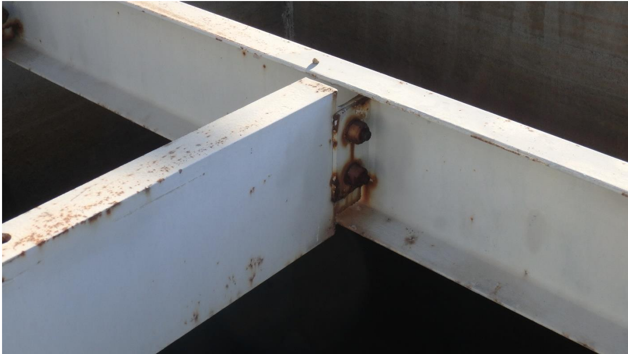
Figure 86. Corrosion on bolted connection for the interior framing support
