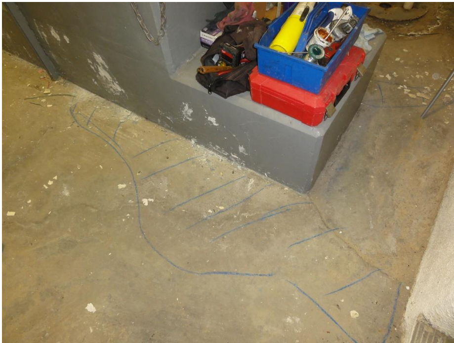
Figure 3. Noted delamination, adjacent to a pipe support pedestal, highlighted in blue
