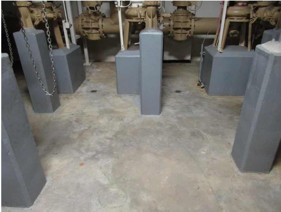
Figure 40. Overall view of concrete framed pipe support pedestals at south end of blower room
