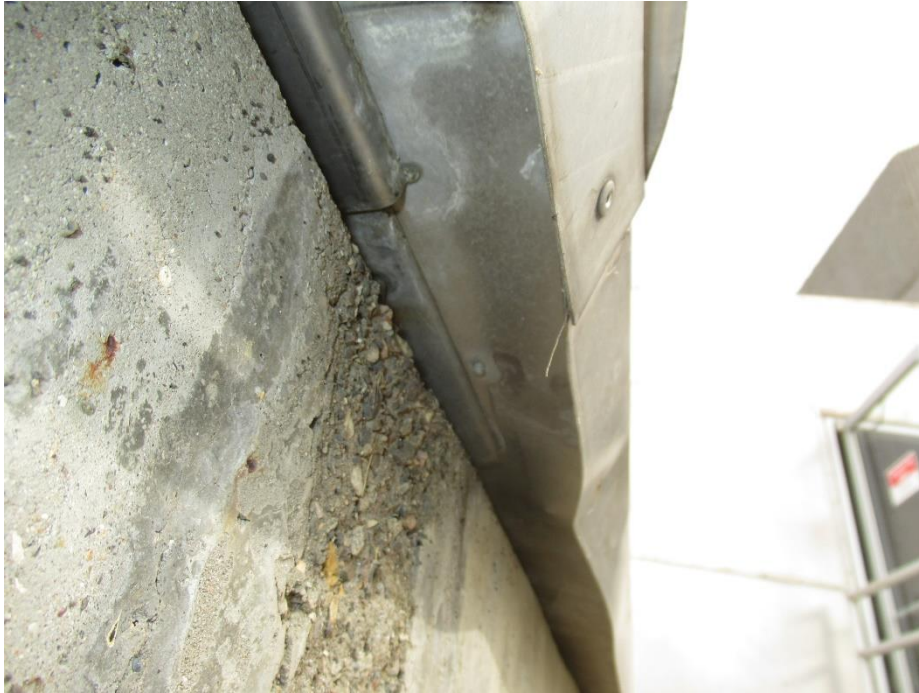
Figure 32. Underside of roof attachment, with a 1-inch wide gap between the roof framing and the top surface of the clarifier walls
