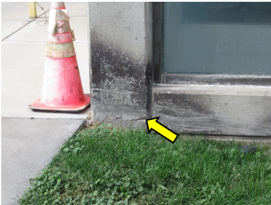
Figure 16. Isolated cracking at base of wall location
