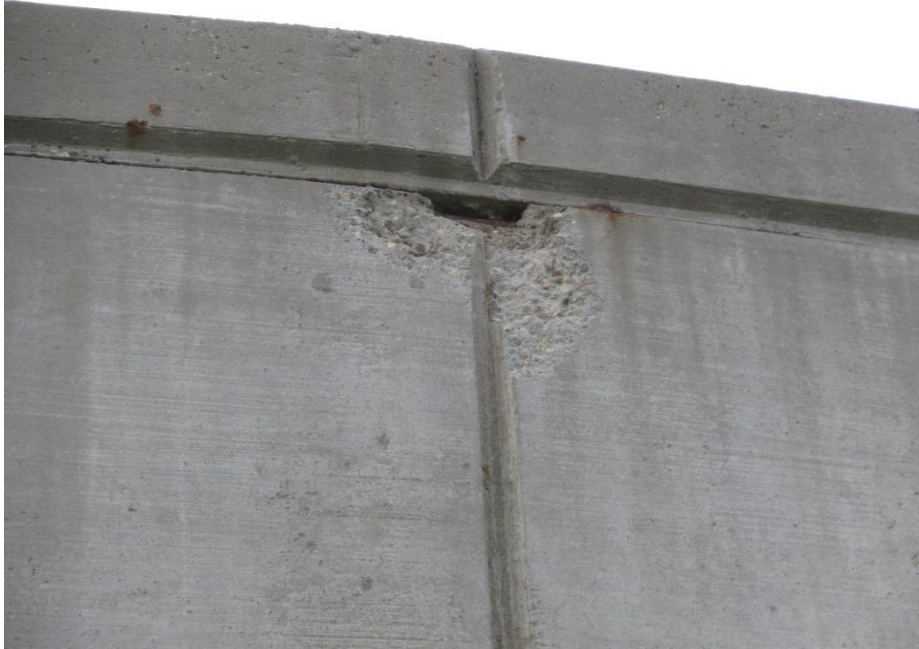
Figure 97. Spalled concrete at upper corner of exterior panel
