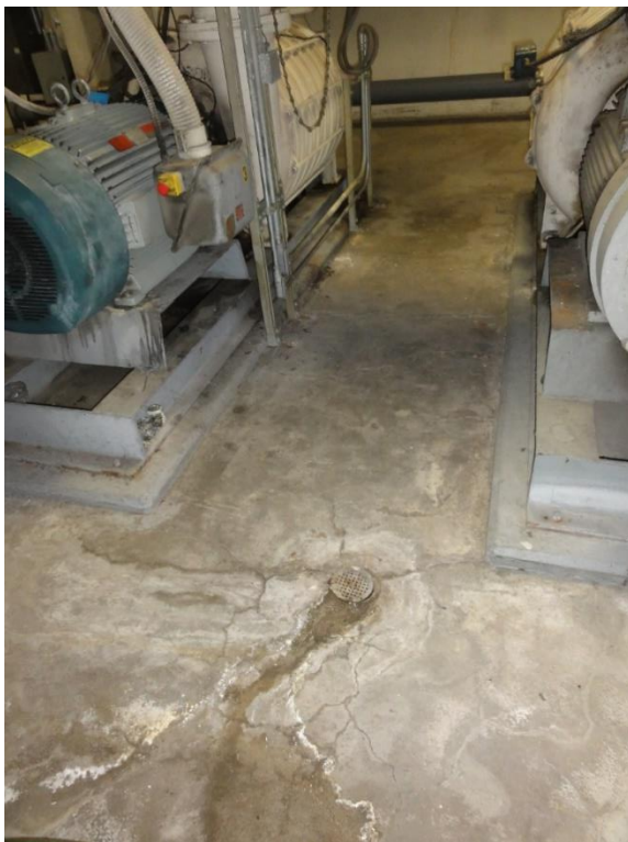
Figure 39. Evidence of ponding water at existing floor drain
