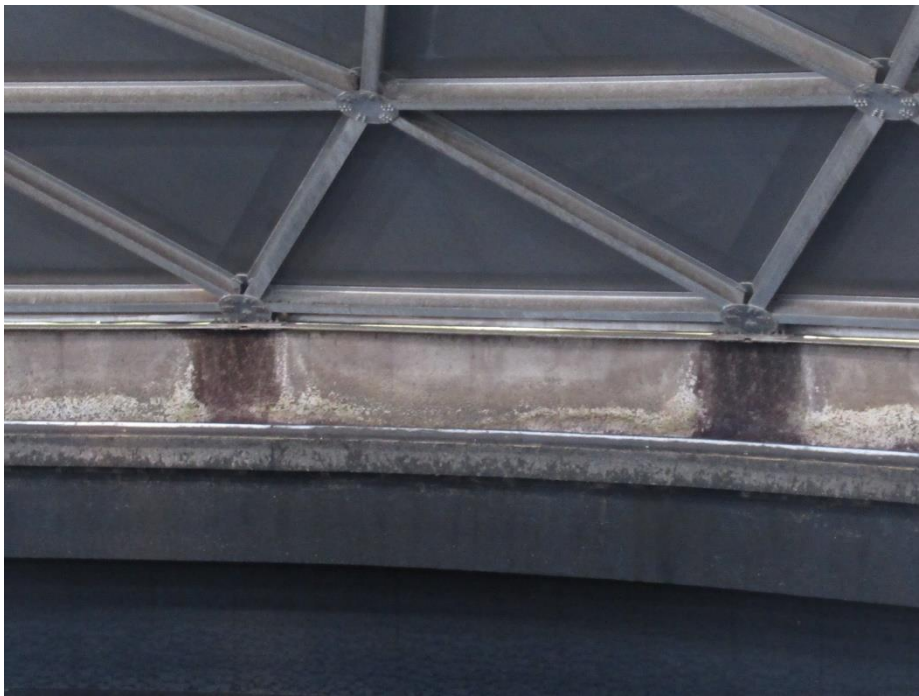
Figure 27. Moisture staining present beneath roof attachment locations
