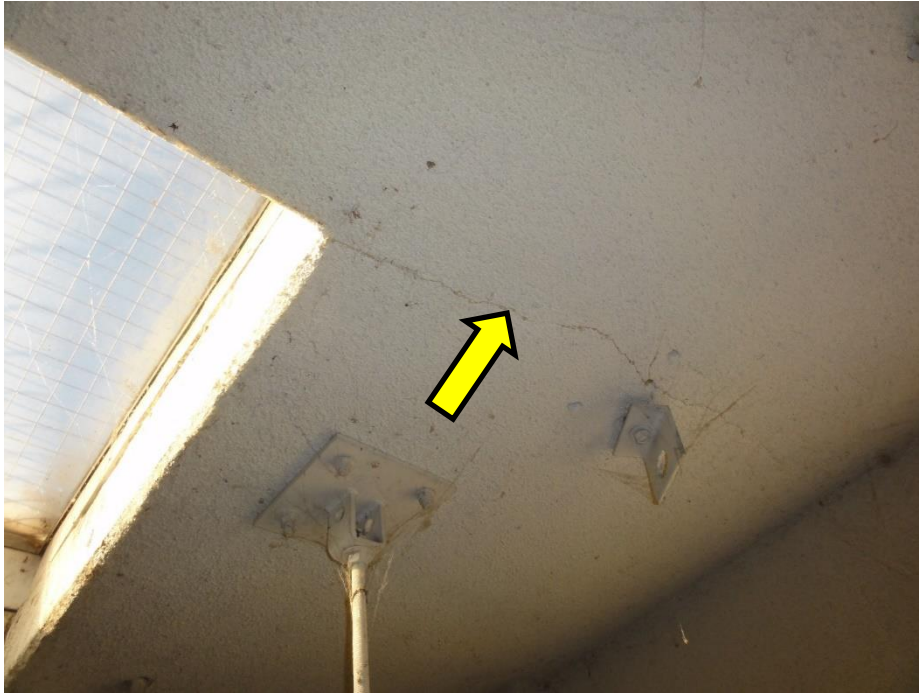
Figure 46. Re-entrant corner cracking at blower room skylight, as observed on the soffit of the ground floor slab
