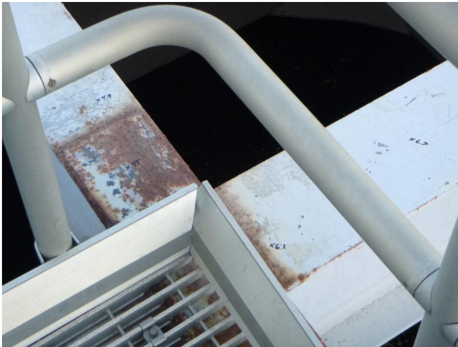
Figure 92. Coating thickness correlated to corrosion distress, note black coating thickness measurements in mils
