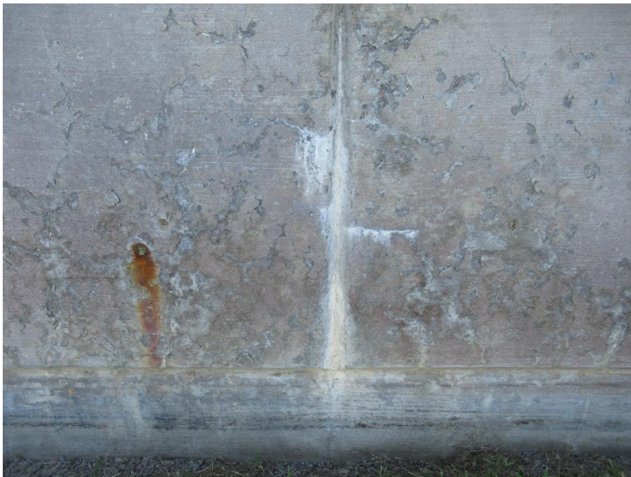
Figure 59. Evidence of moisture intrusion and efflorescence staining at reveal joint
