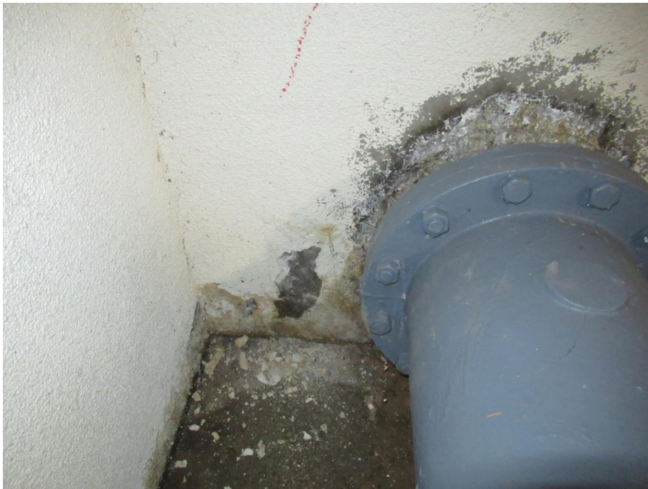
Figure 43. Sounded delaminated coating adjacent to piping element at the north elevation wall
