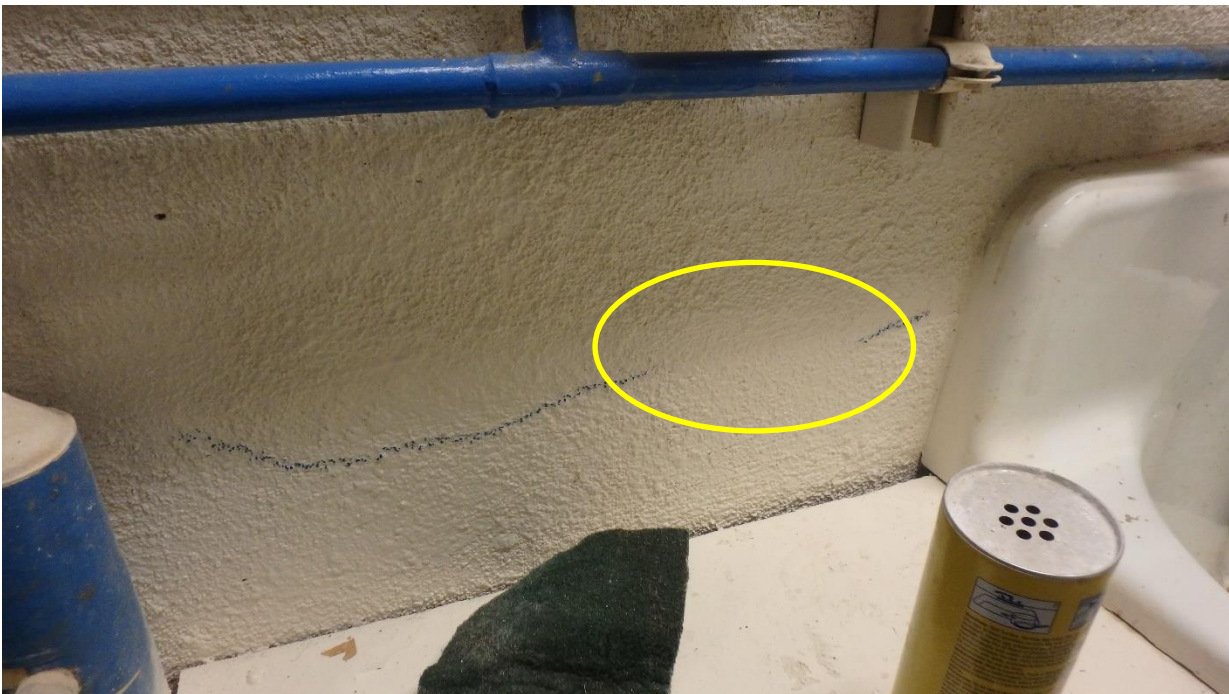
Figure 105. Previous coating repair location at the south digester interior wall
