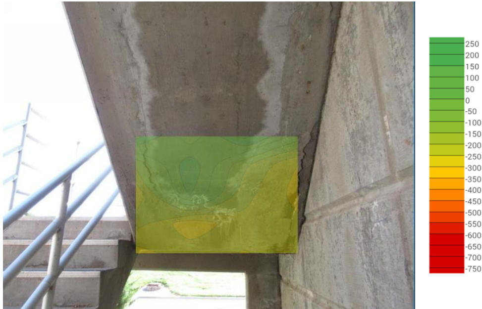
Figure 72. Half-cell potential data overlaid on top of photo documenting spalling and staining at underside of ground level staircase. The color scale is in mV and the reference electrode is a CSE
