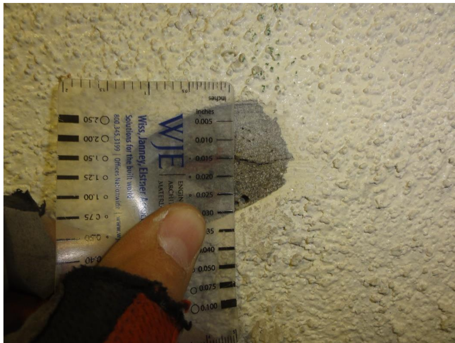
Figure 11. 15 mil crack observed in concrete substrate, that had not yet propagated through the wall coating
