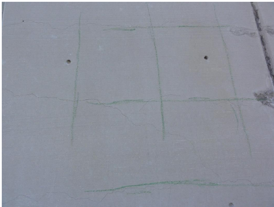
Figure 57. Typical longitudinal and transverse cracking, aligning with locations of embedded reinforcing (reinforcing traced in green)
