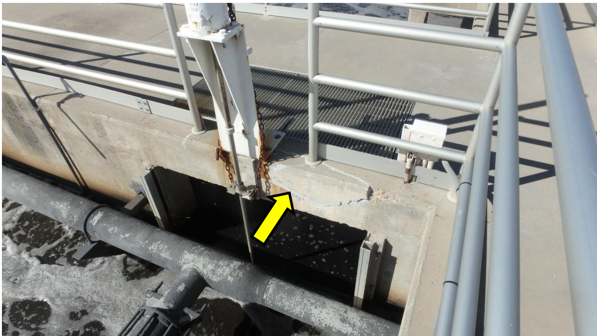
Figure 49. Previously installed sealant at incipient spall location
