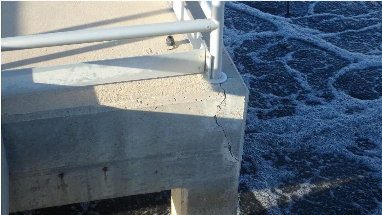
Figure 48. Incipient spall at guardrail post embed
