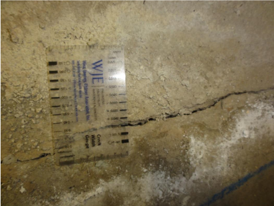
Figure 2. Measurement of a crack at the topping slab.
