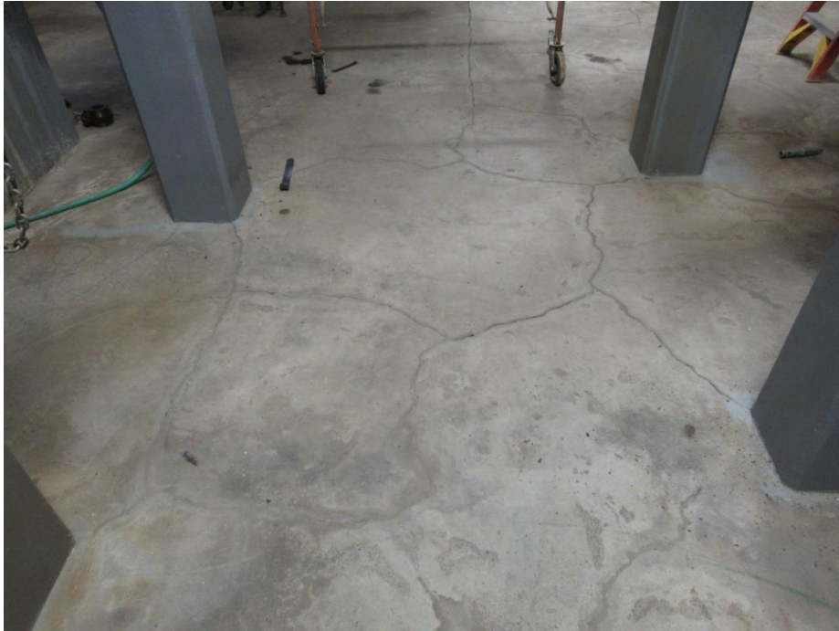
Figure 38. Typical topping slab cracking
