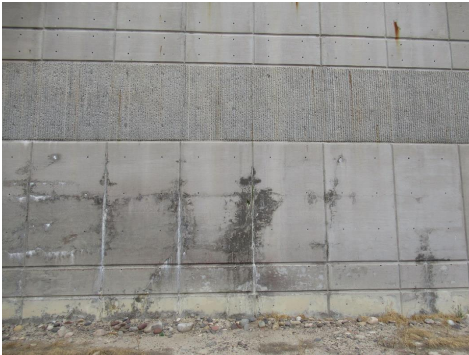
Figure 60. Evidence of moisture intrusion and efflorescence staining at reveal joints
