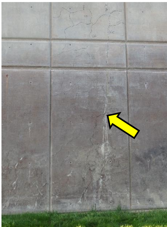
Figure 89. Vertical cracking at exterior of blending tank
