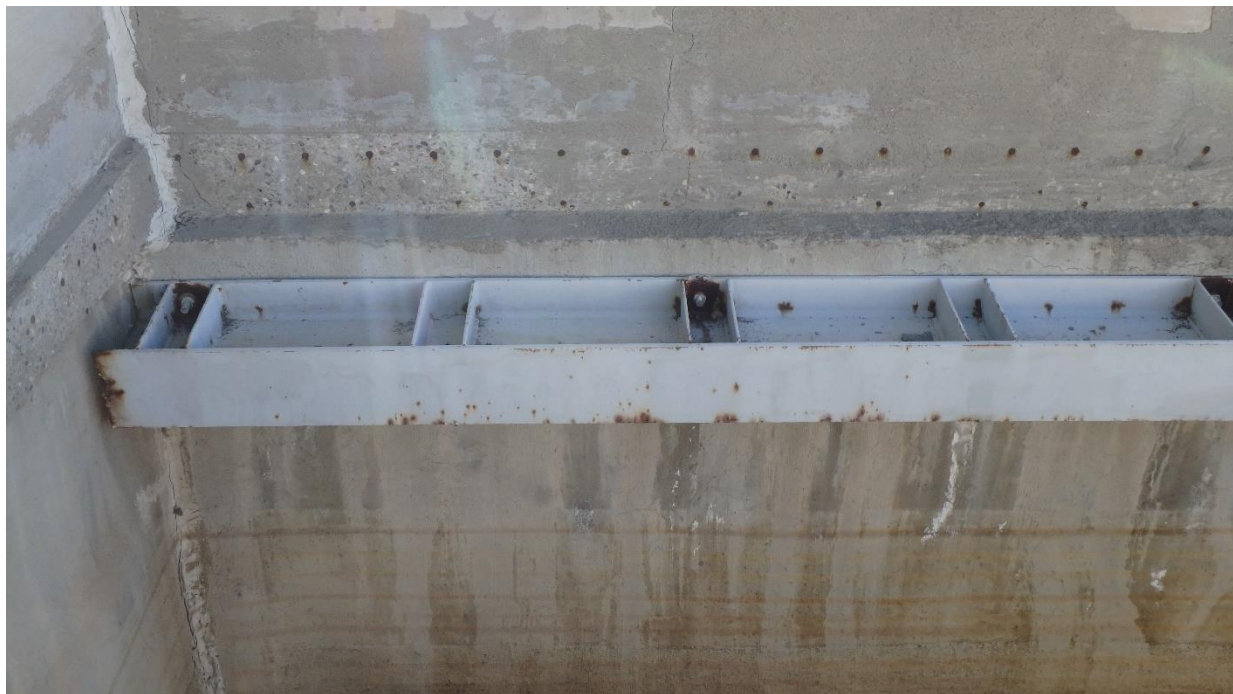
Figure 81. Typical steel framing and attachment at north and west walls of blending tank
