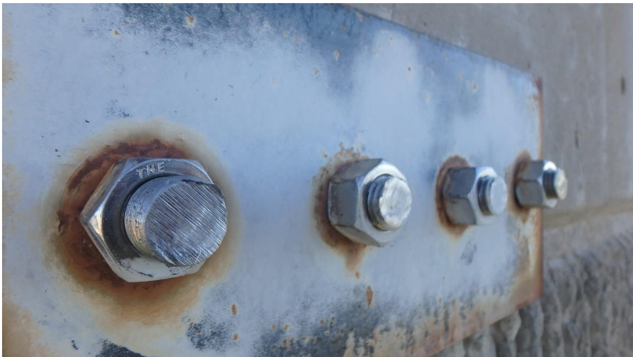
Figure 83. Corrosion of plate washers adjacent to bolt attachments, as viewed from the exterior of the blending tank walls
