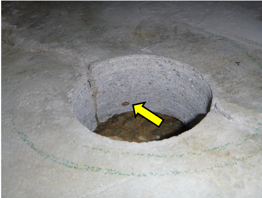
Figure 25. WWR observed near the bottom surface of the extracted core
