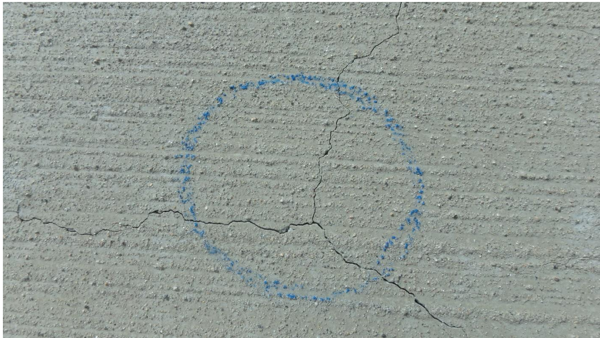
Figure 75. Core sample location at east elevation wall, intersecting multiple surface cracks
