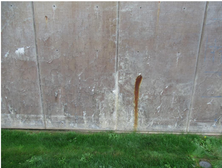
Figure 91. Noted efflorescence at panel reveal joint
