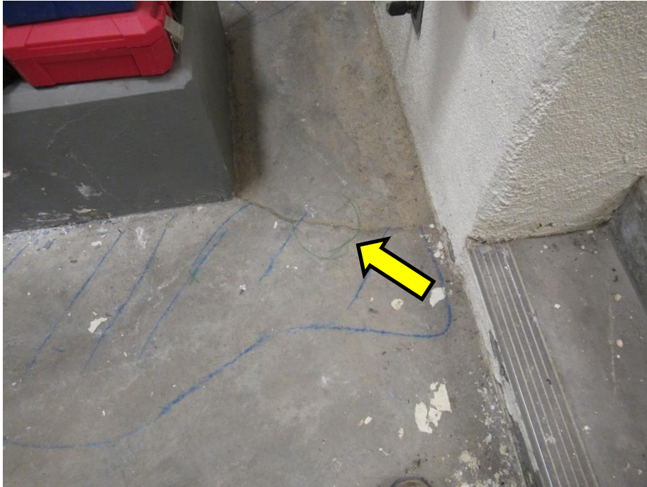
Figure 23. Core location through topping slab crack
