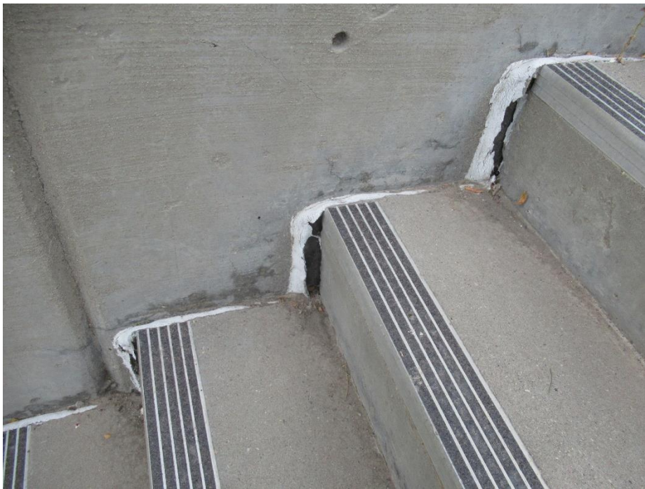
Figure 67. Sealant joint between the ground level stairs and the adjacent building face that had failed and was no longer in contact with both substrate surfaces
