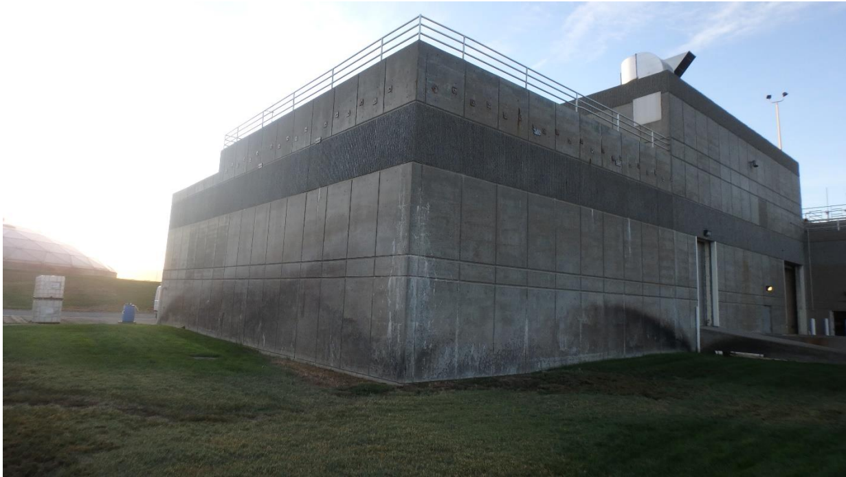
Figure 90. Noted efflorescence and staining at northwest corner of blending tank
