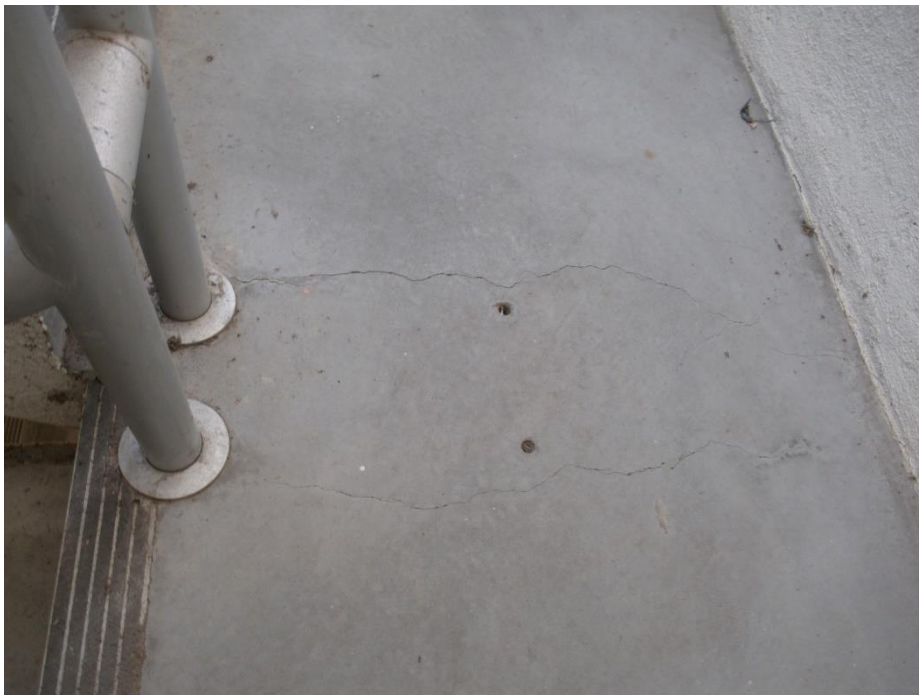
Figure 8. Isolated stair landing cracks
