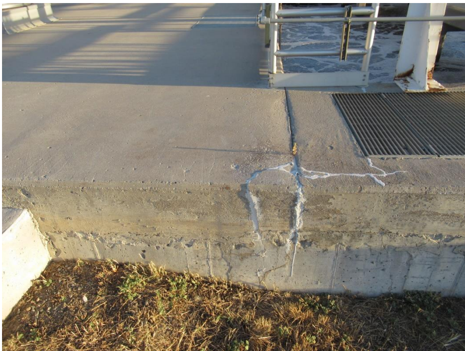
Figure 53. Previously installed sealant at incipient spall location
