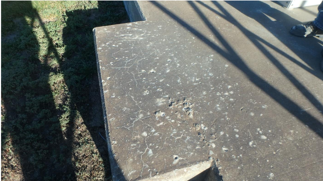
Figure 52. Map pattern cracking and scaling at catwalk topside
