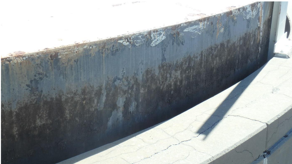
Figure 107. Overall view of the coating on the vertical surface "rim skirt" of the south digester lid
