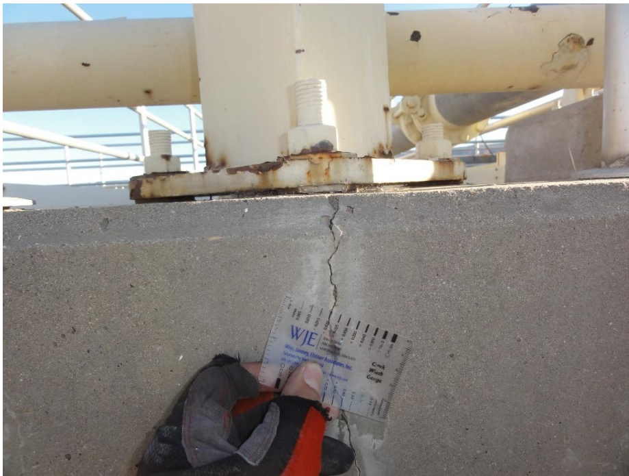
Figure 71. Isolated transverse cracking aligning with guardrail post embeds for the catwalks above
