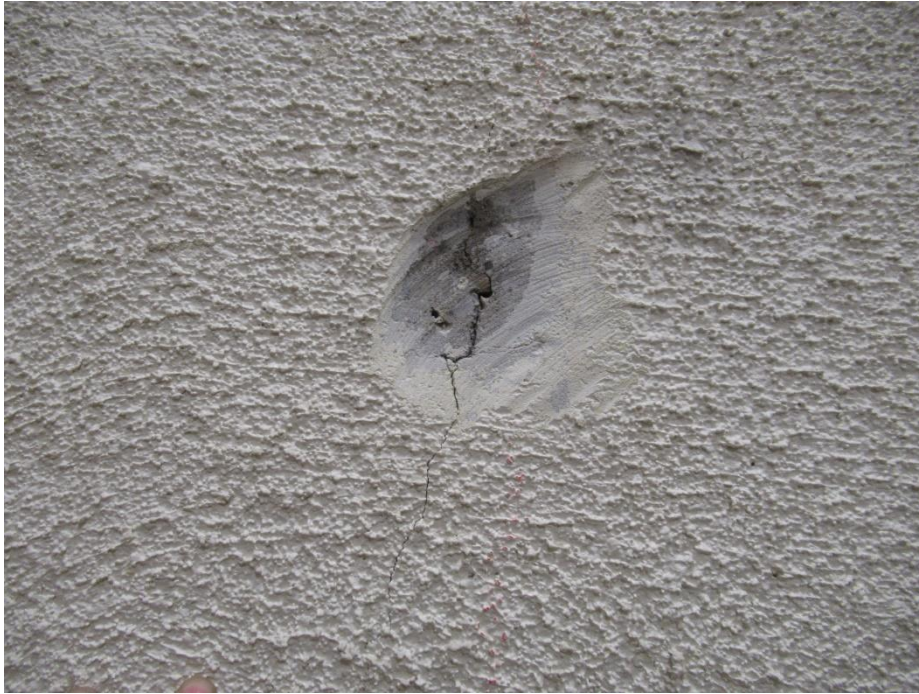
Figure 9. Typical coating installation at interior wall surfaces, with crack highlighted where coating was removed.
