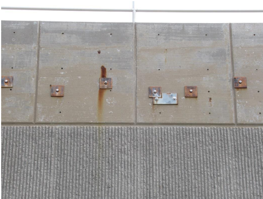
Figure 82. Corrosion of plate washers, as viewed from the exterior of the blending tank walls
