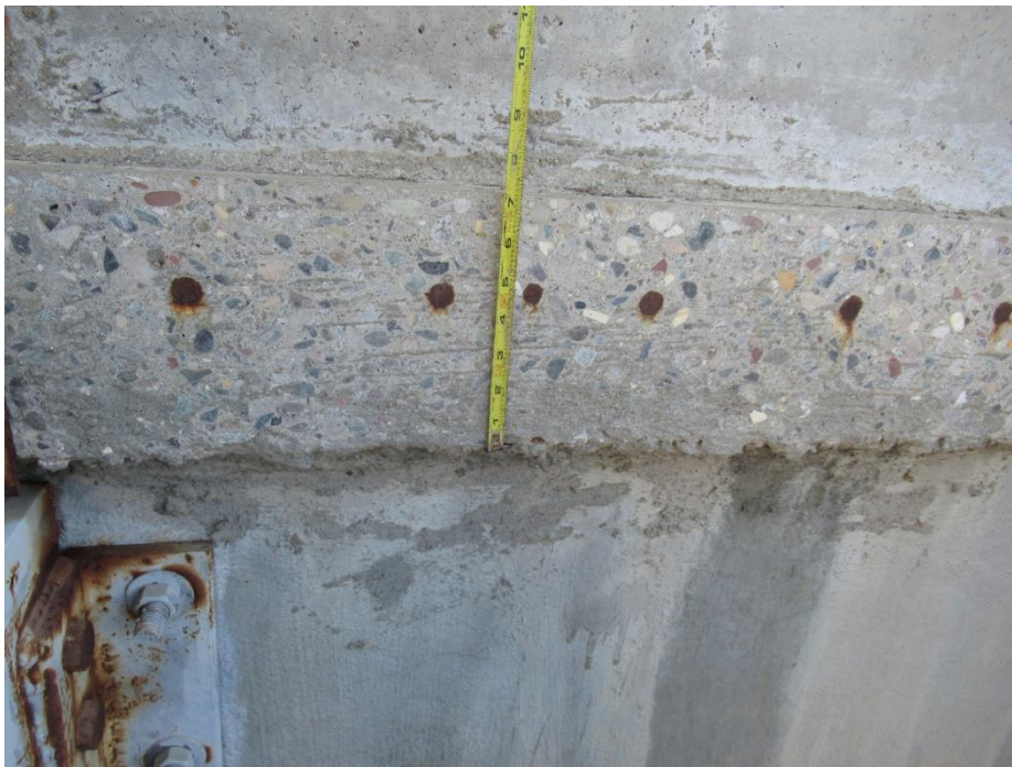
Figure 87. Surface corrosion on previously sawcut reinforcing, which was abandoned when concrete lid/roof was removed
