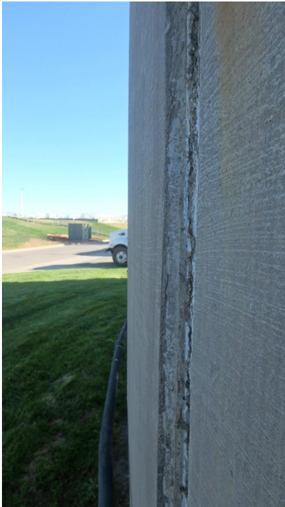
Figure 99. Outward bowing of panel in the background at a vertical sealant joint, with respect to the panel in the foreground
