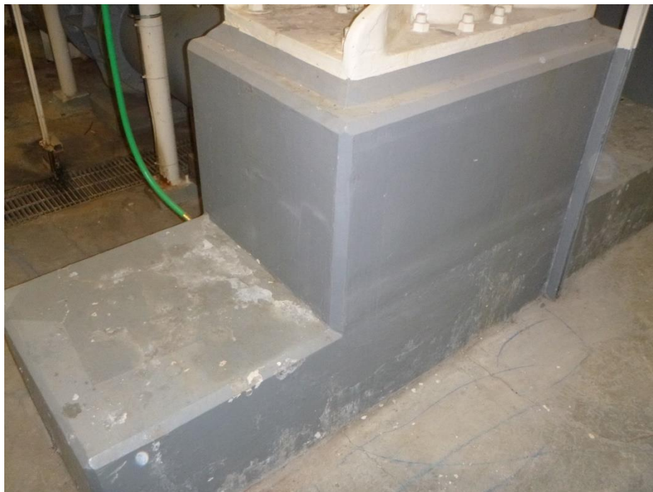
Figure 6. Typical concrete support pedestal
