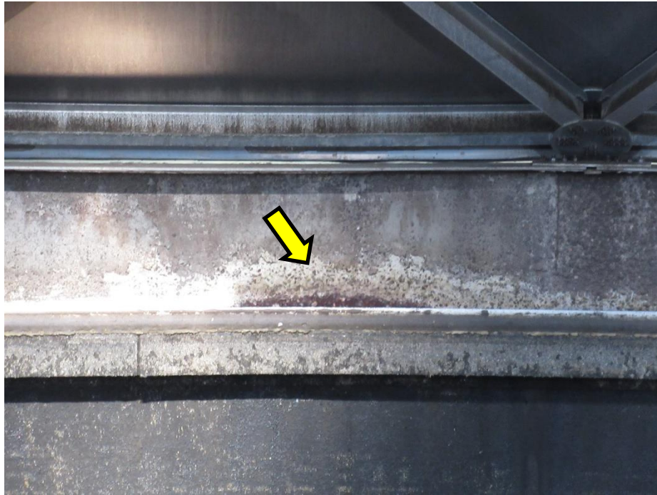
Figure 28. Paste erosion within the effluent trough
