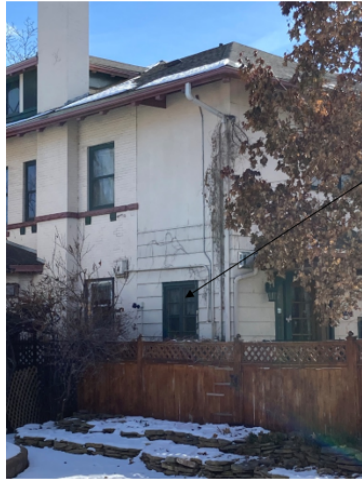
These windows to be replaced.
