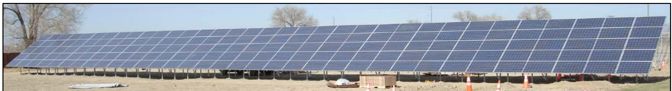
Solar Plant at the Persigo Wastewater Treatment Facility
