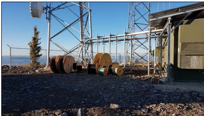
Grand Mesa Tower Site
