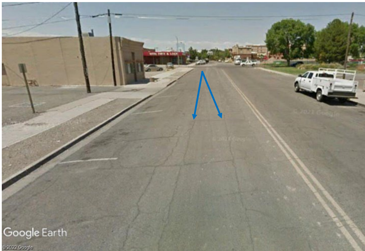
Figure 47. 5ME.24074.1. Parallel cracks can be seen in the pavement along the 300 block of 2nd Street between Ute and Pitkin Avenues. View north. Image courtesy of Google Earth.
