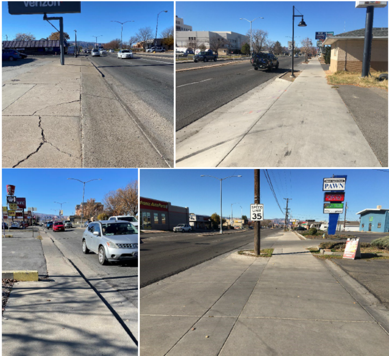
FIGURE 8: CURB CUTS AND SIDEWALK CONDITIONS ON NORTH AVENUE
