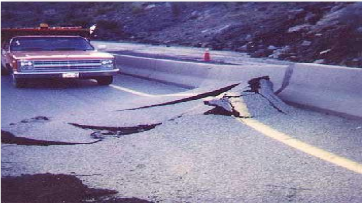
FIGURE 12 PHOTO OF DEBEQUE CANYON SLIDE AREA- INTERSTATE 70
