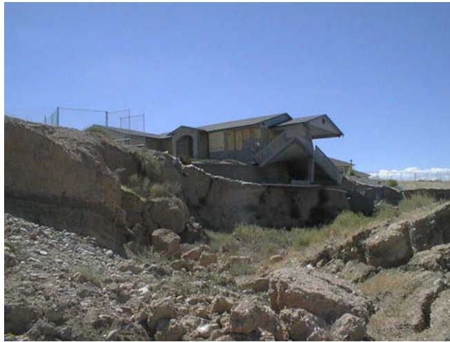
Unstable slopes along the bluffs south of the Colorado River, west of the Redlands Parkway
