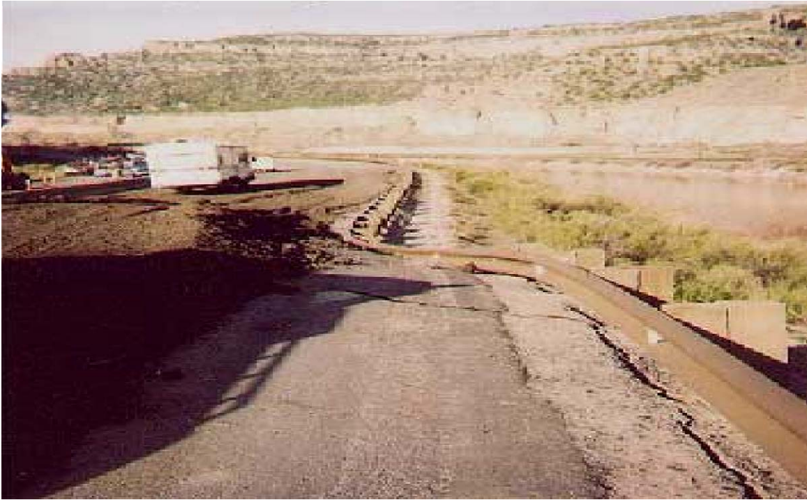
Figure 11: Photo of DeBeque Canyon Slide Area – Interstate 70
