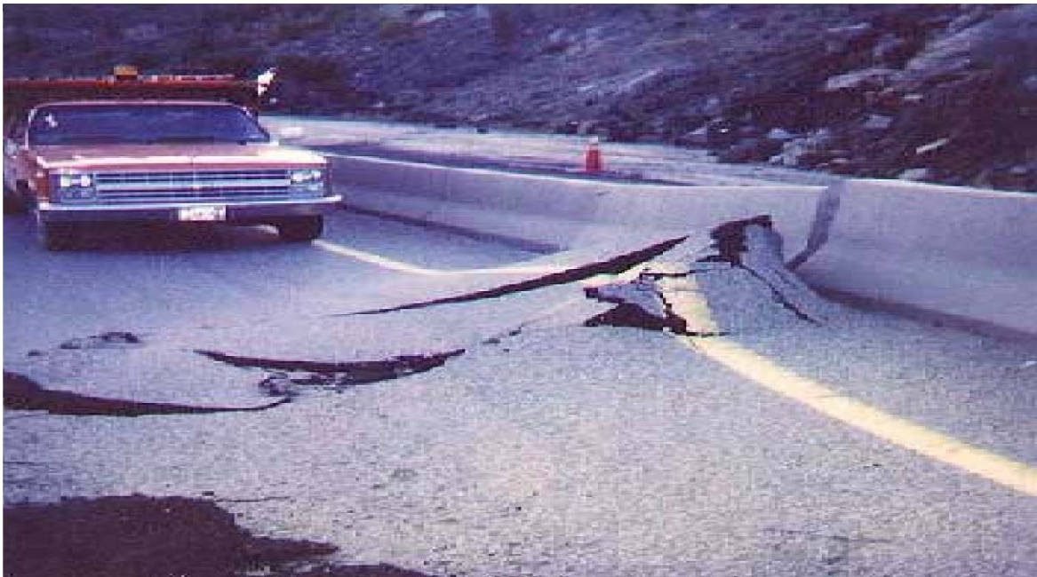
Figure 12: Photo of DeBeque Canyon Slide Area – Interstate 70
