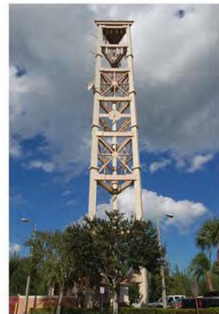
Modified Lattice Tower
