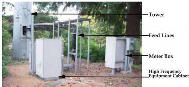
Figure 1: Example of High Band Wireless Infrastructure Ground Equipment
