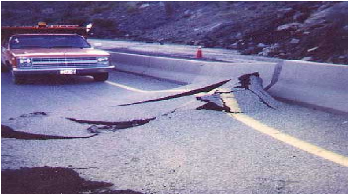
Figure 12: Photo of DeBeque Canyon Slide Area – Interstate 70
