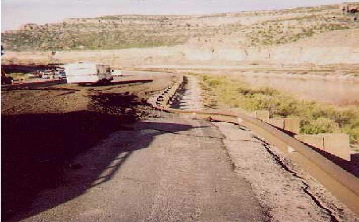
Figure 11: Photo of DeBeque Canyon Slide Area – Interstate 70
