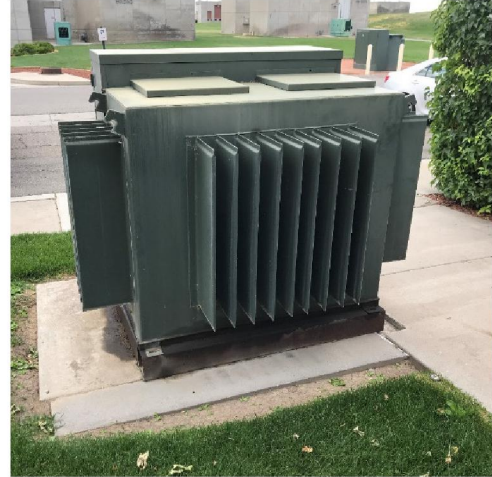
Figure 7.3 Administration Building Transformer
