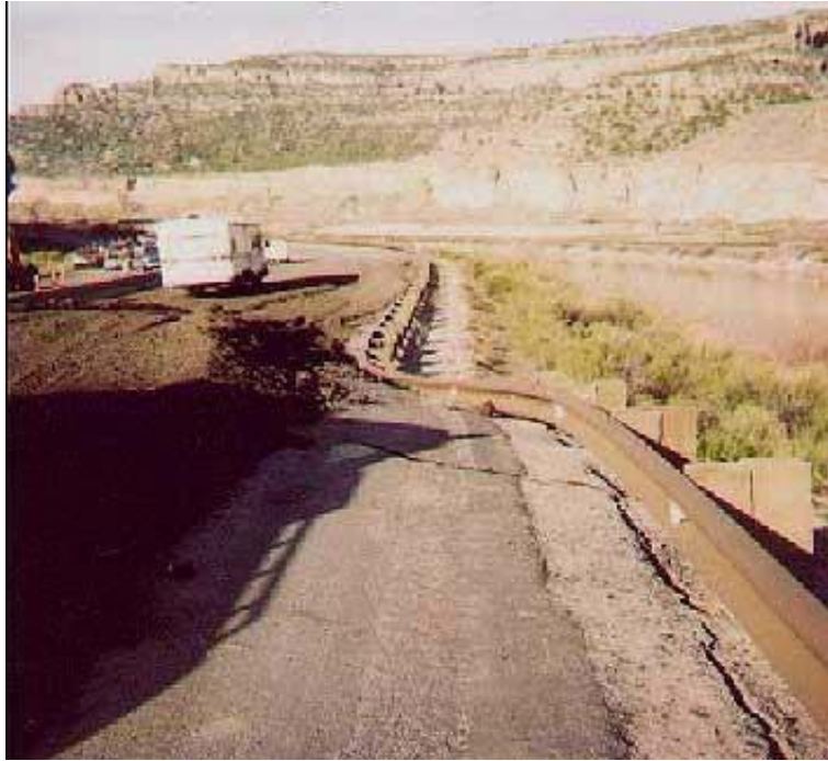
Figure 11: Photo of DeBeque Canyon Slide Area – Interstate 70
