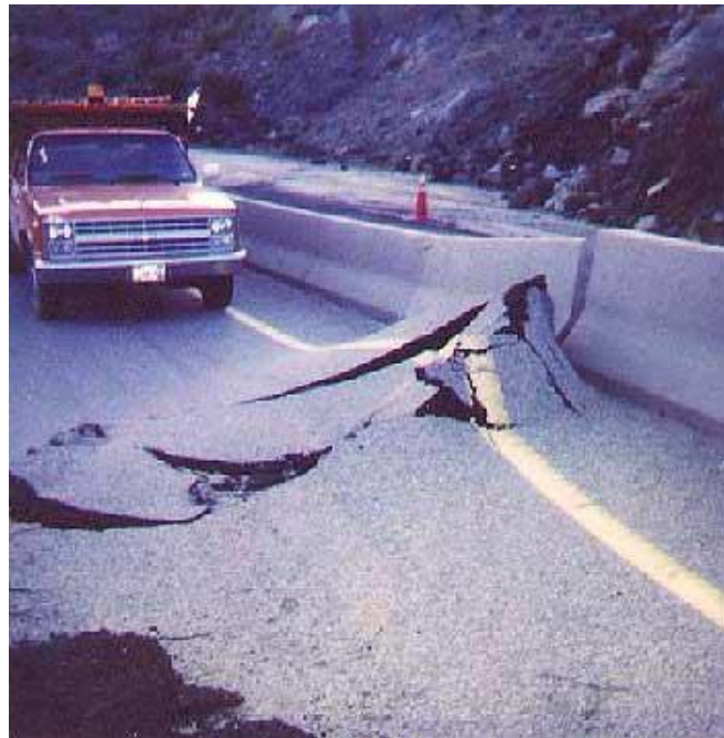
Figure 12: Photo of DeBeque Canyon Slide Area – Interstate 70
