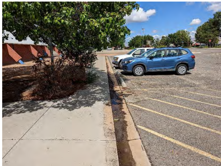
Picture 2, Non-Functional curbing
