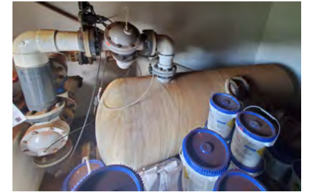
EXISTING POOL FILTER
