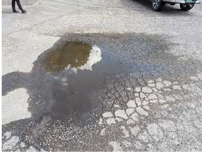
Picture 1, Pavement failure near northern area inlet
