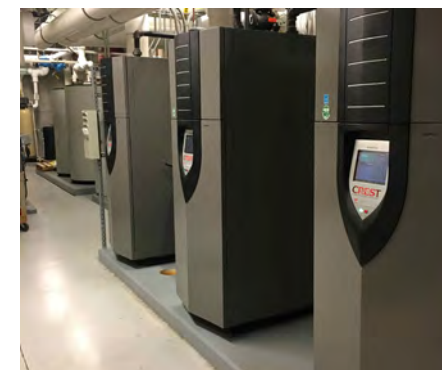
NEW POOL HEATER
