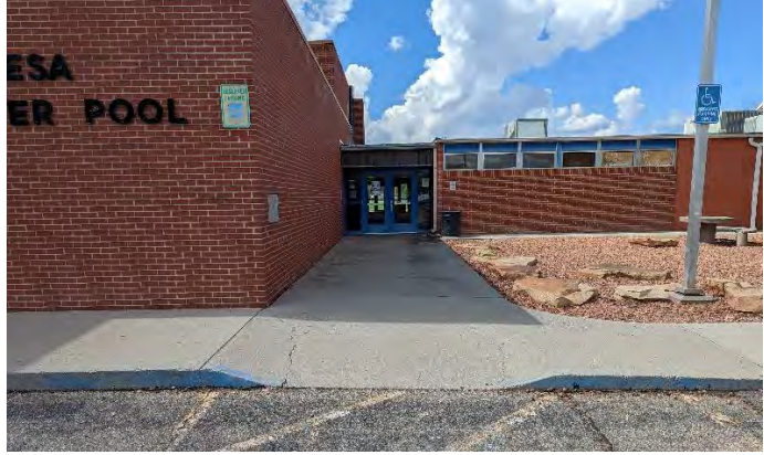
Picture 4, Non-conforming ADA access to Pool
