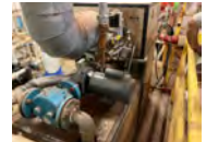
EXISTING POOL HEATER
