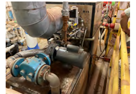
EXISTING POOL HEATER
