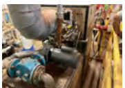
EXISTING POOL HEATER
