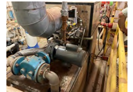
EXISTING POOL HEATER
