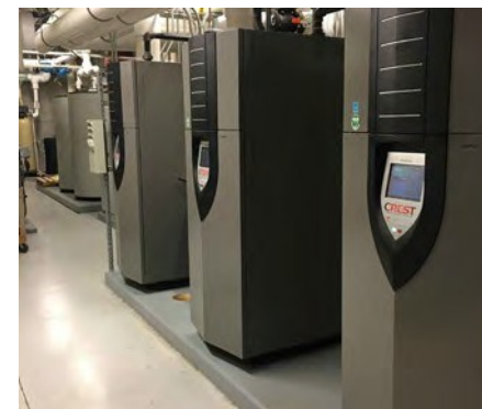
NEW POOL HEATER
