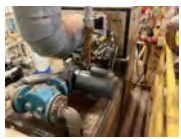
EXISTING POOL HEATER
