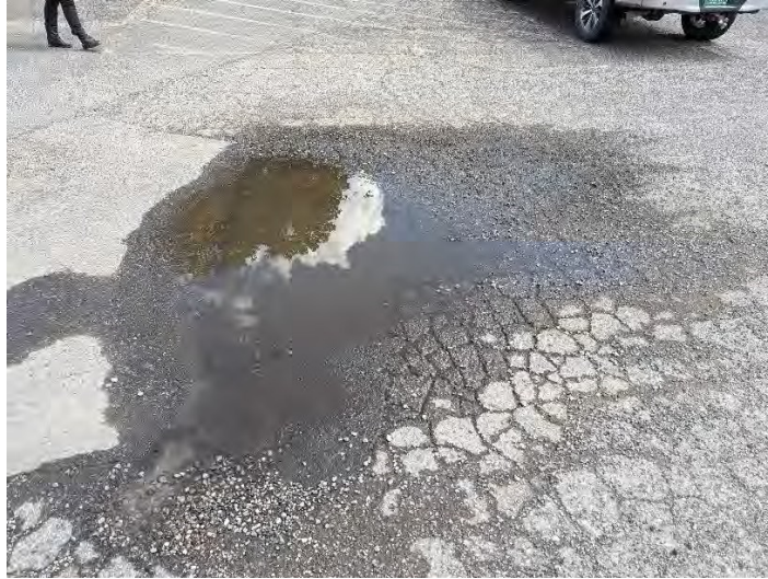
Picture 1, Pavement failure near northern area inlet
