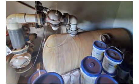
EXISTING POOL FILTER
