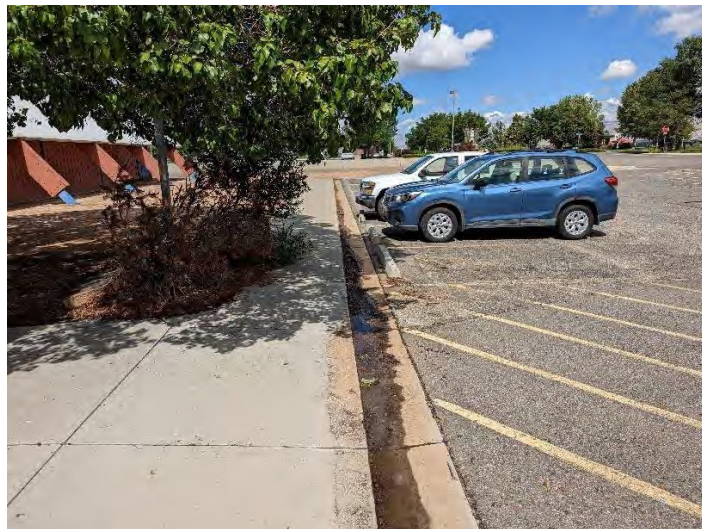
Picture 2, Non-Functional curbing
