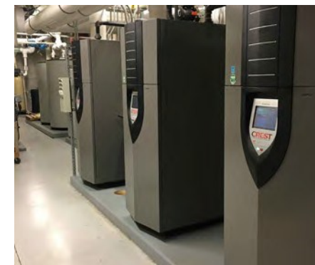
NEW POOL HEATER
