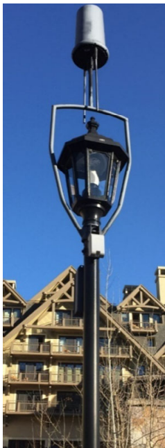
Streetlight 4G transmitter in Vail
