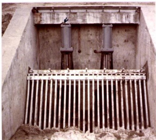
LOW LEVEL GATES ← POCKET CAUSED BY DIRT IN FORMS
