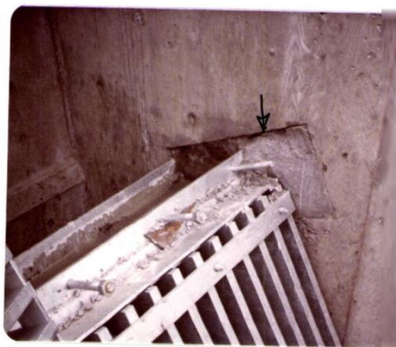
POORLY GROUTED BEAM POCKET ON UPPER LEVEL INTAKE.
