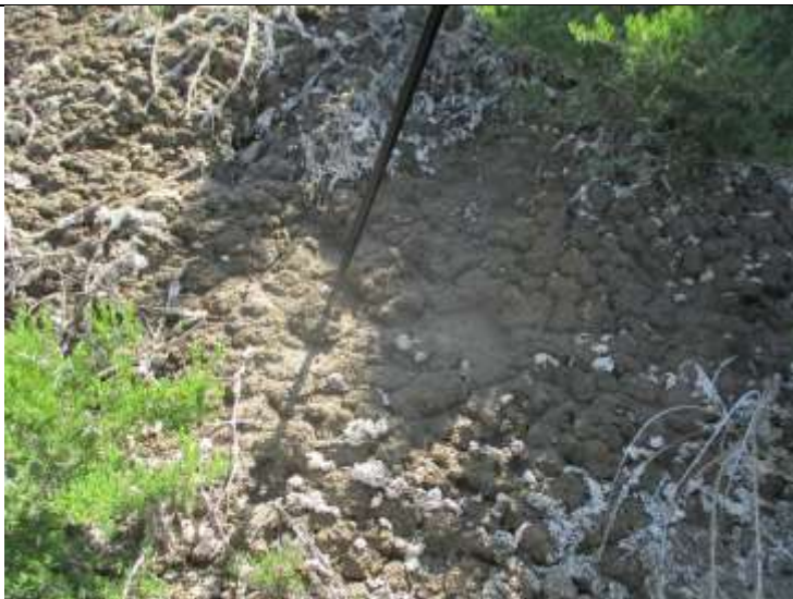
Seepage area, marked by moist soils and alkali salts. Recommend to visually observe as reservoir levels continue to rise.
