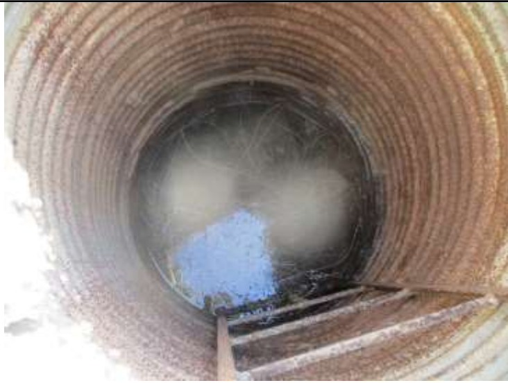
VCP runs through bottom of manhole.
