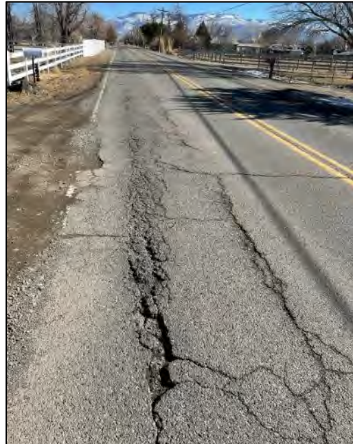
Figure 9. High severity fatigue cracking in wheel path
