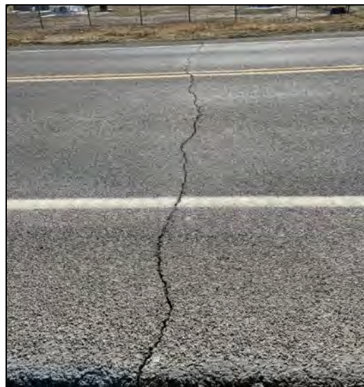
Figure 6. Typical infrequent and low severity transverse cracking along D ½ Road.
