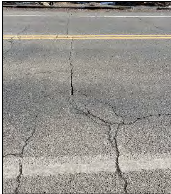
Figure 12. Typical pavement distress along 26 ½ Rd
