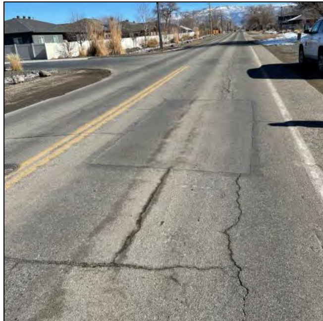
Figure 3. Typical longitudinal and transverse cracking along B 1/2 Road with fatigue cracking in wheel path and minor patch deterioration along the perimeter.
