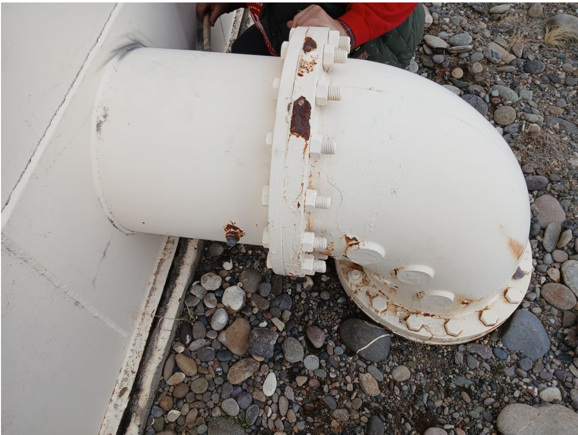
Photo 29. Exterior view of shell outlet nozzle
