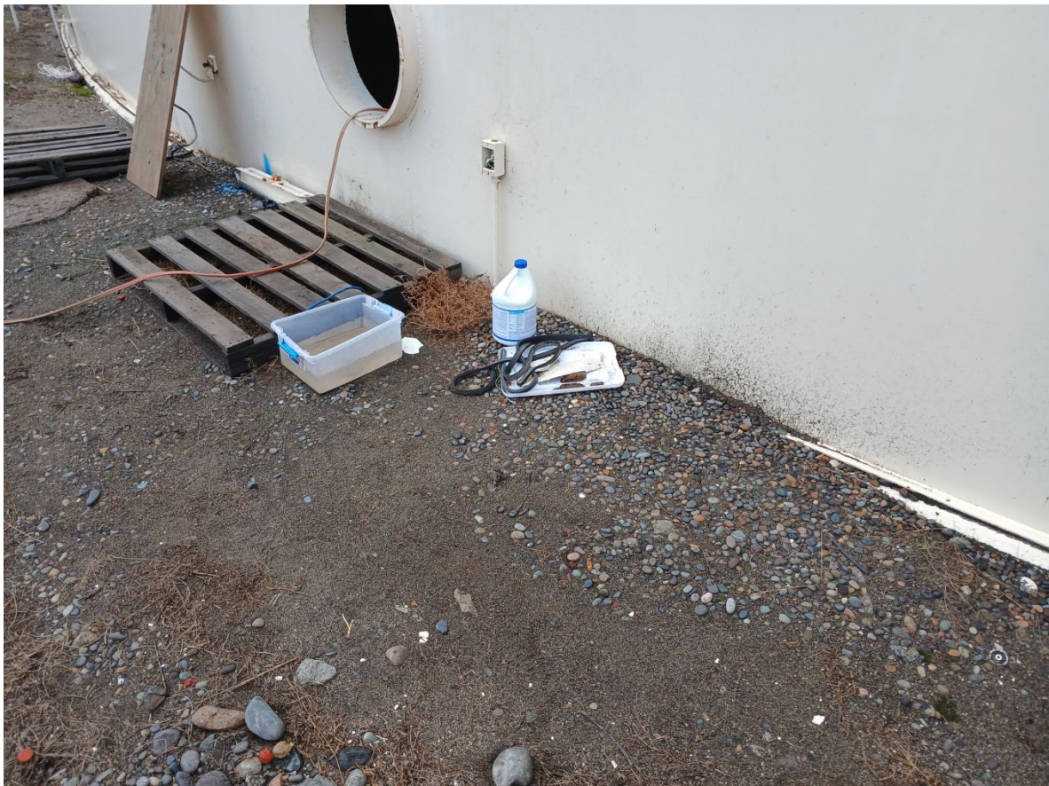
Photo 10. Surrounding grade higher than bottom plate projection
