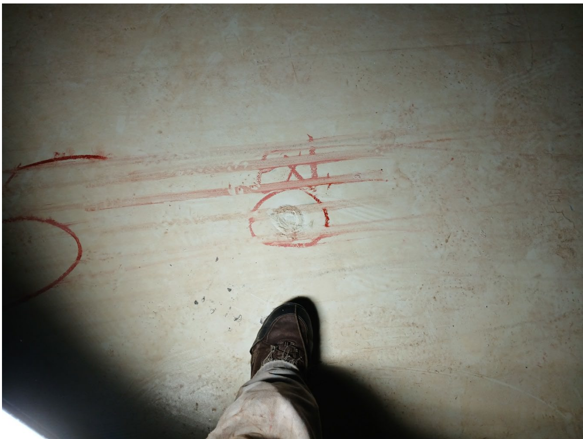
Photo 58. Example of extraneous weld on tank bottom plate
