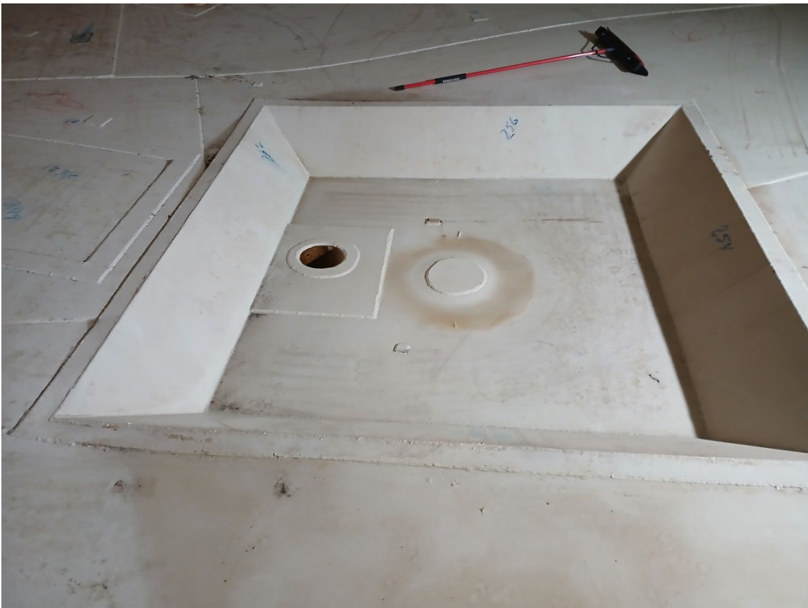
Photo 35. Sump and drain configuration
