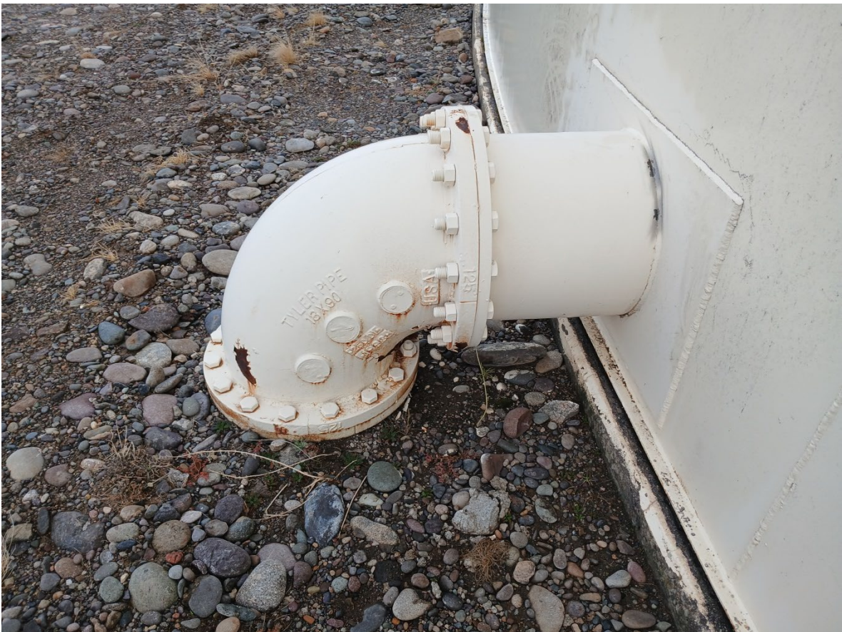
Photo 30. Exterior view of shell outlet nozzle
