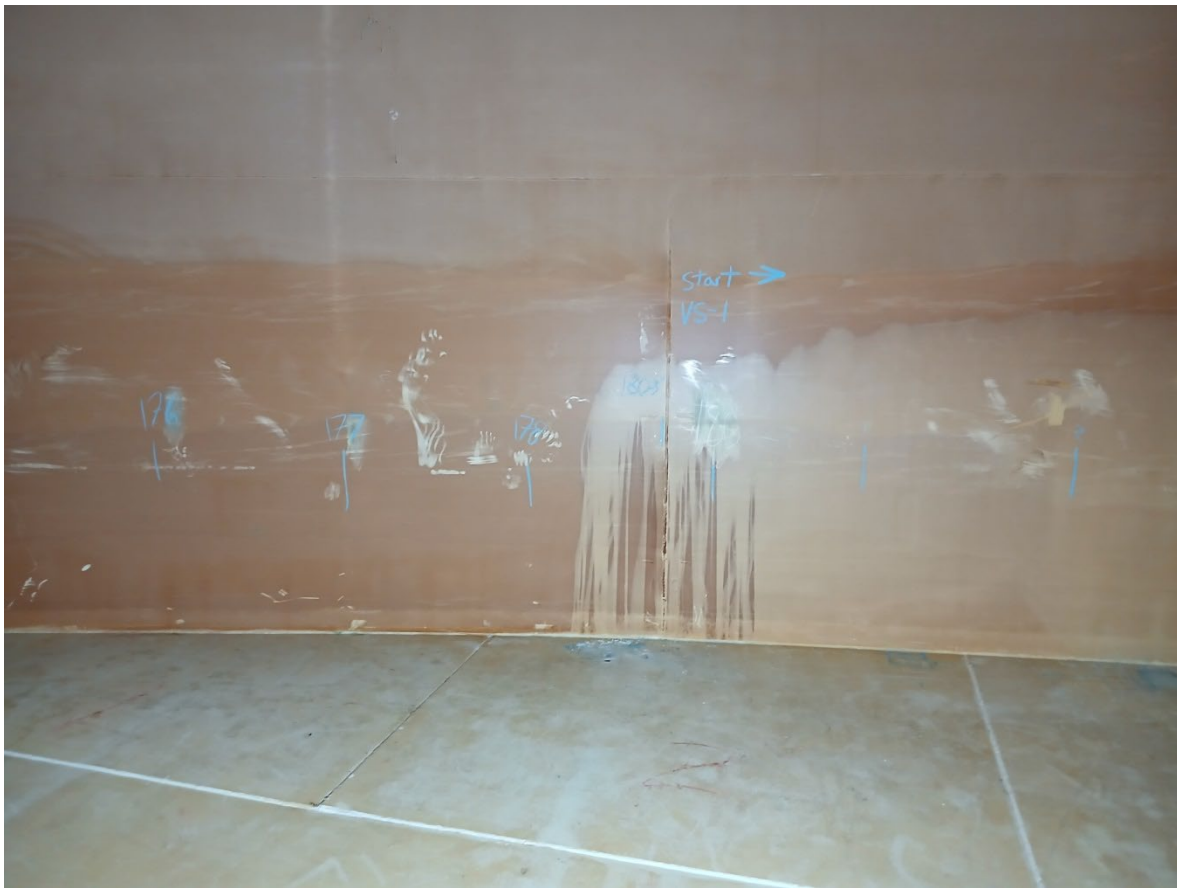
Photo 63. Bottom course vertical weld seam VS-1, starting point for critical zone and shell UT readings
