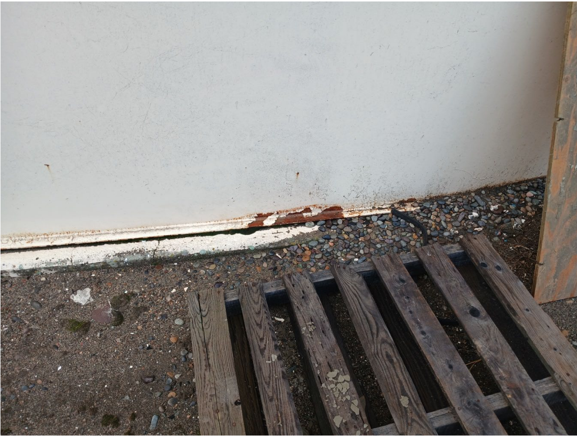
Photo 11. Area of paint failure with rust at bottom plate projection
