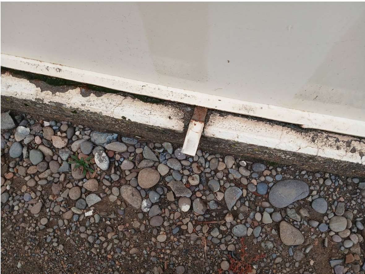
Photo 16. As found corroded piece of flat steel bar between concrete ring wall and bottom
