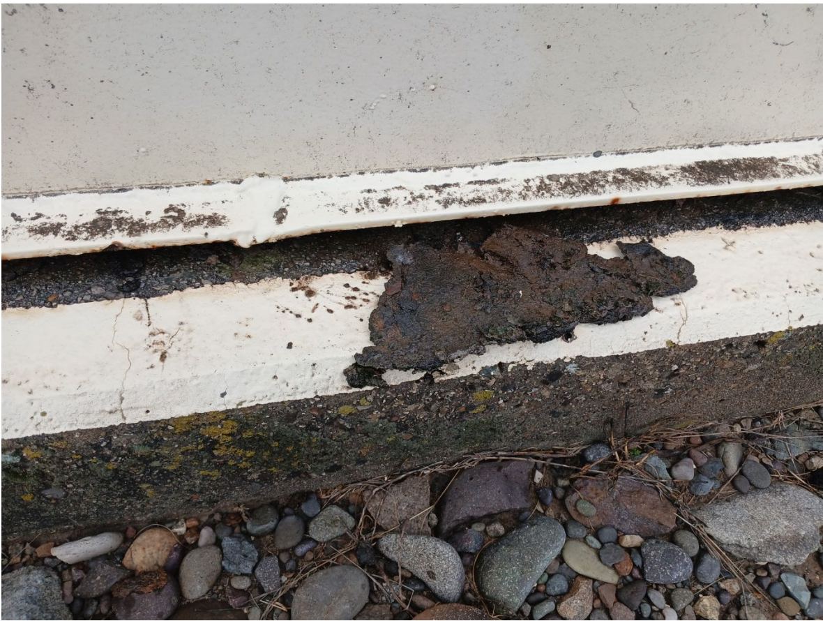
Photo 15. Remnant of asphalt impregnated fiberboard between concrete ring wall and bottom
