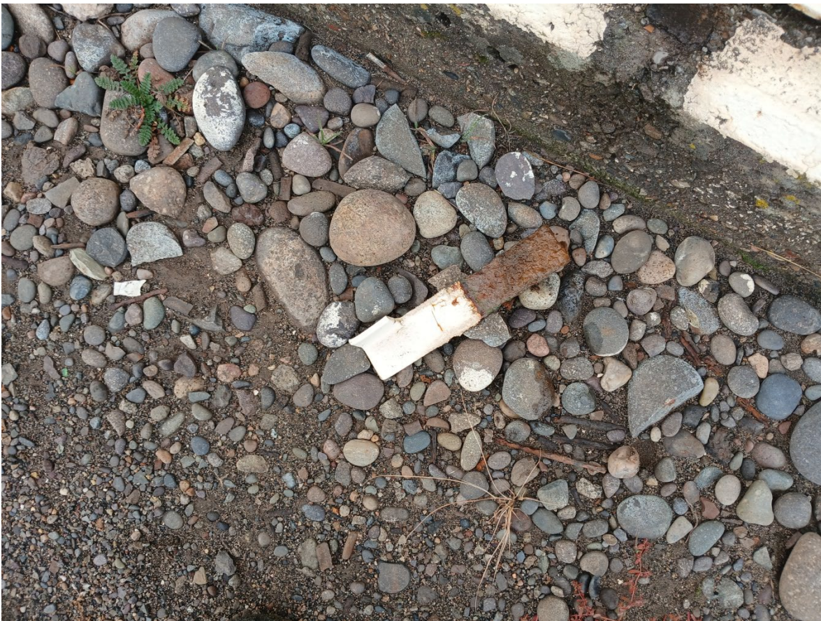
Photo 17. Corroded piece of flat steel bar between concrete ring wall and bottom
