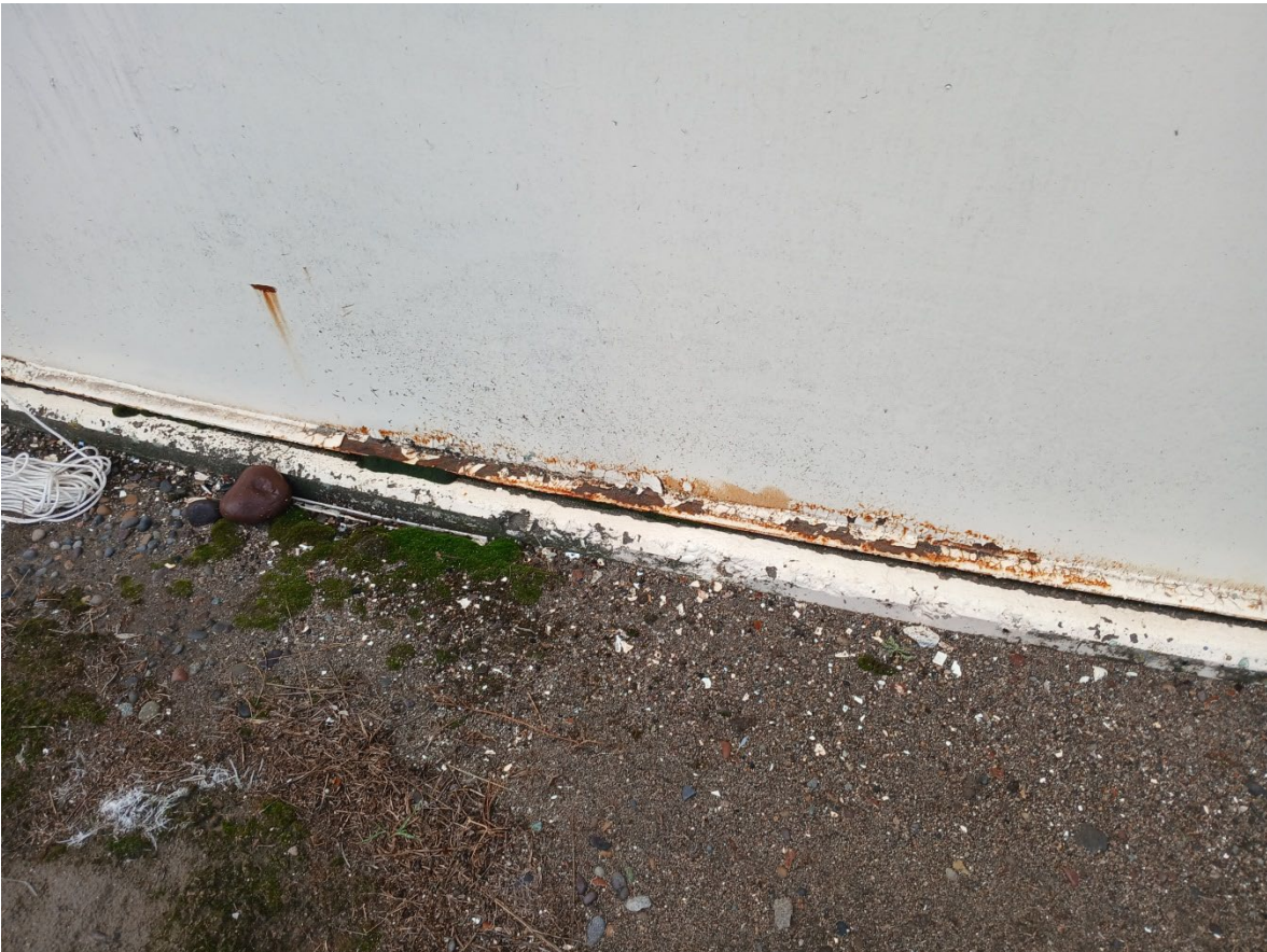
Photo 12. Area of paint failure with rust at bottom plate projection
