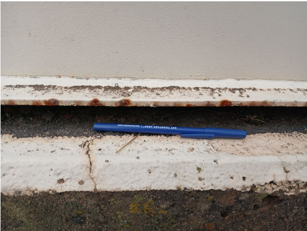
Photo 14. Air gap between concrete ring wall and bottom plate projection
