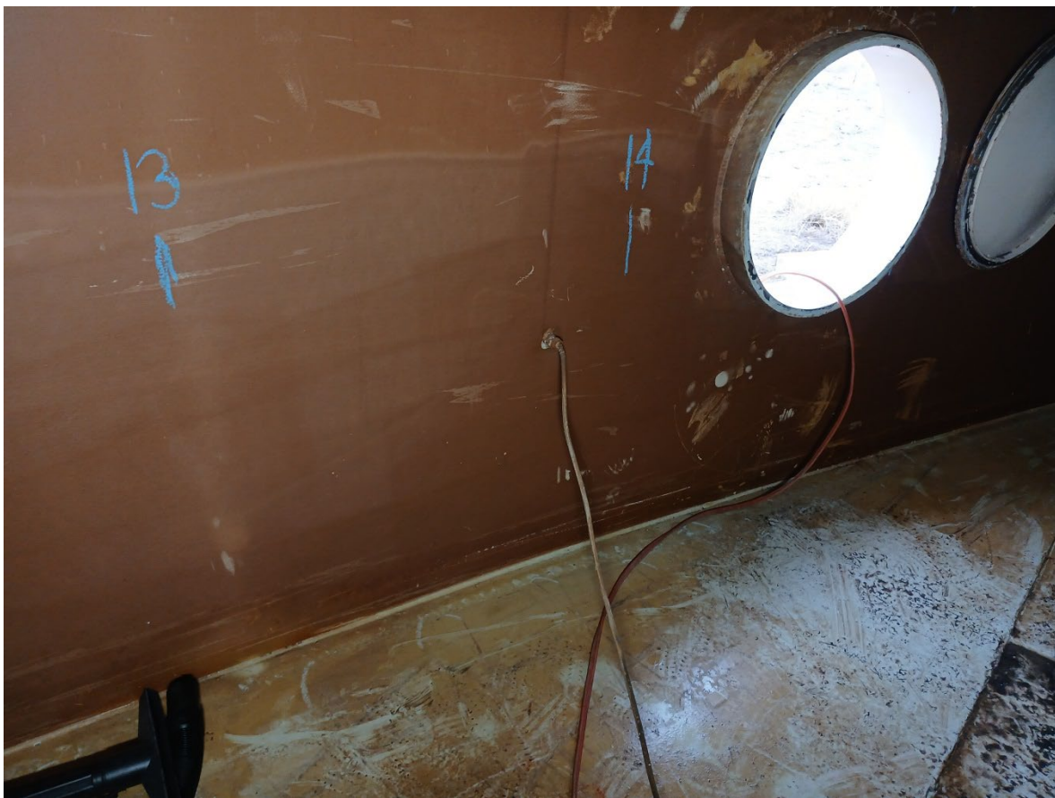
Photo 21. Shell connection for internal impressed current CP system
