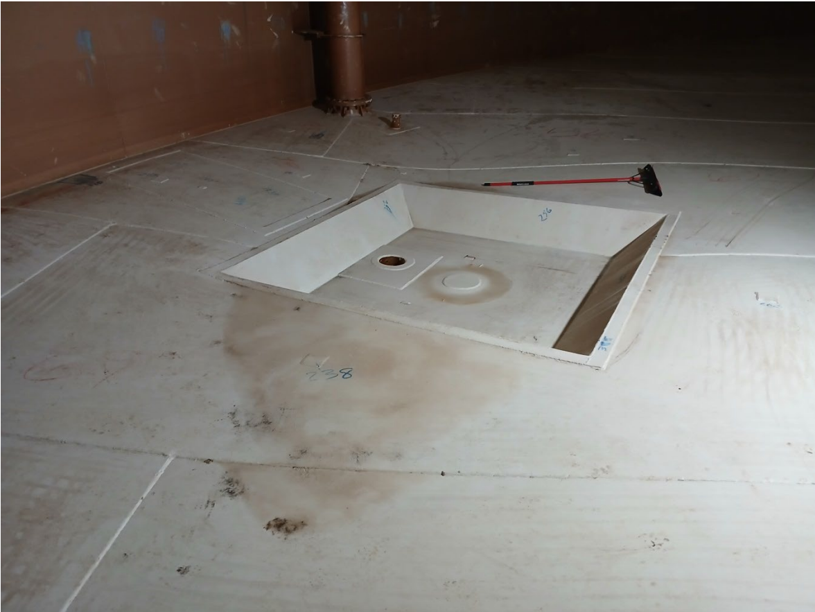
Photo 34. Sump and drain configuration
