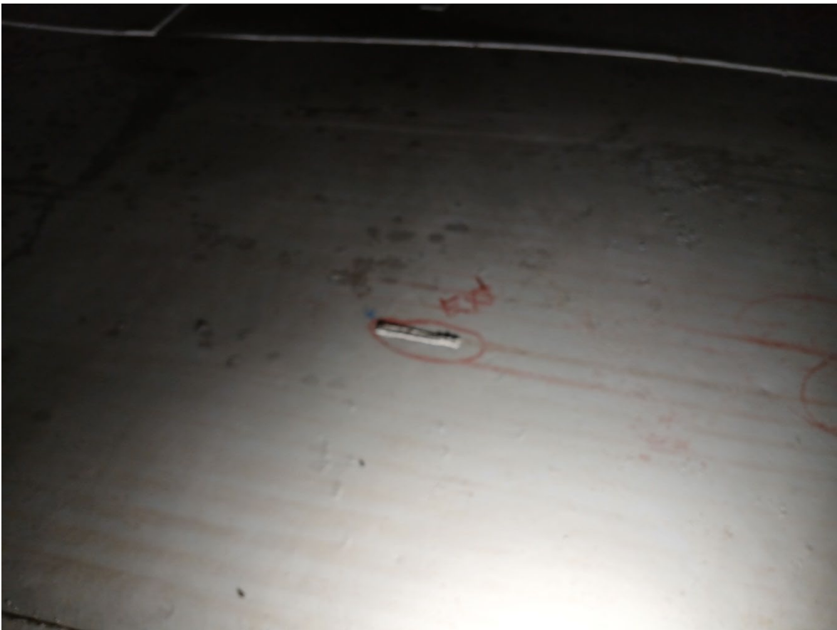
Photo 60. Example of extraneous weld on tank bottom plate
