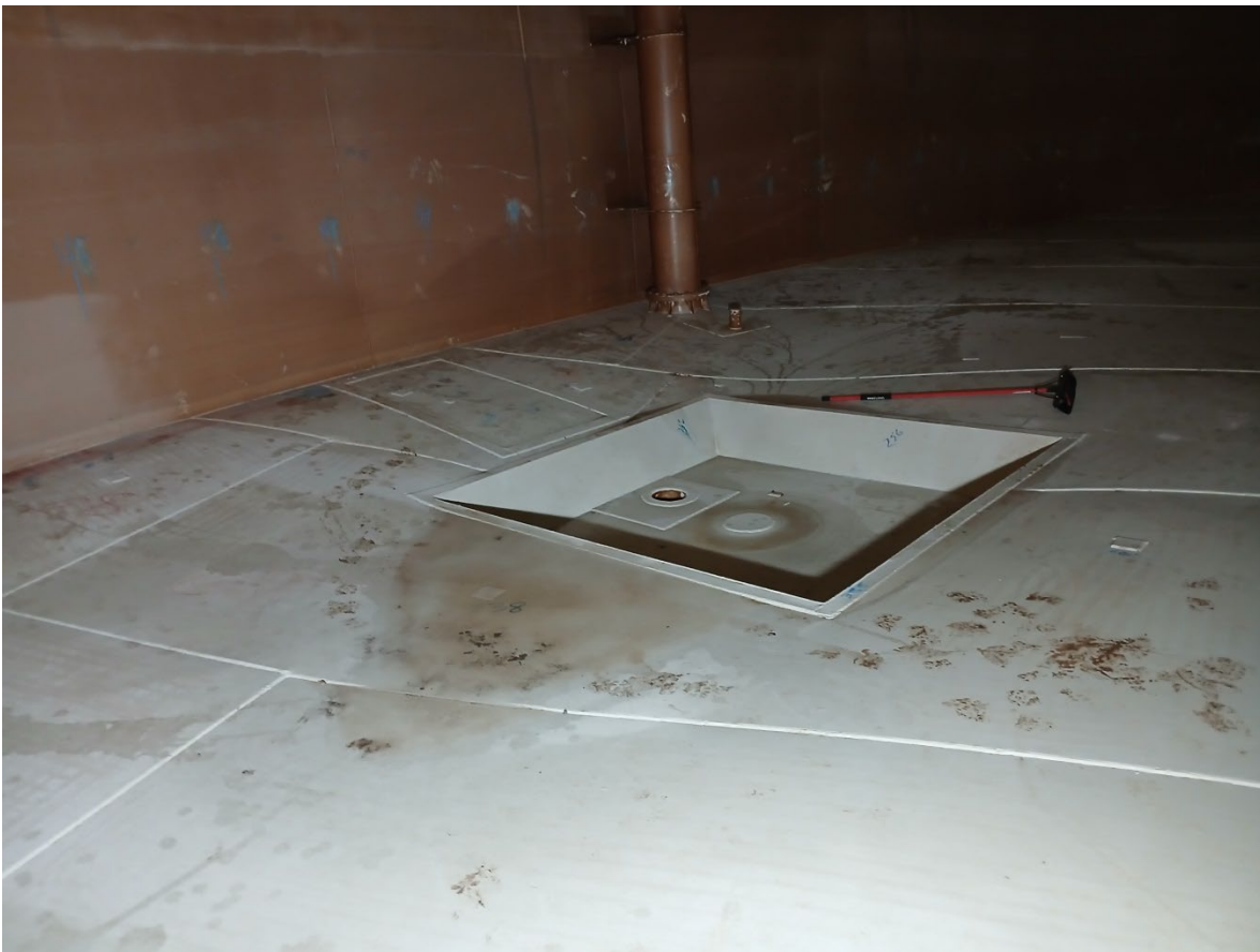
Photo 37. Sump and drain configuration, scattered small fillet welded patches on tank bottom
