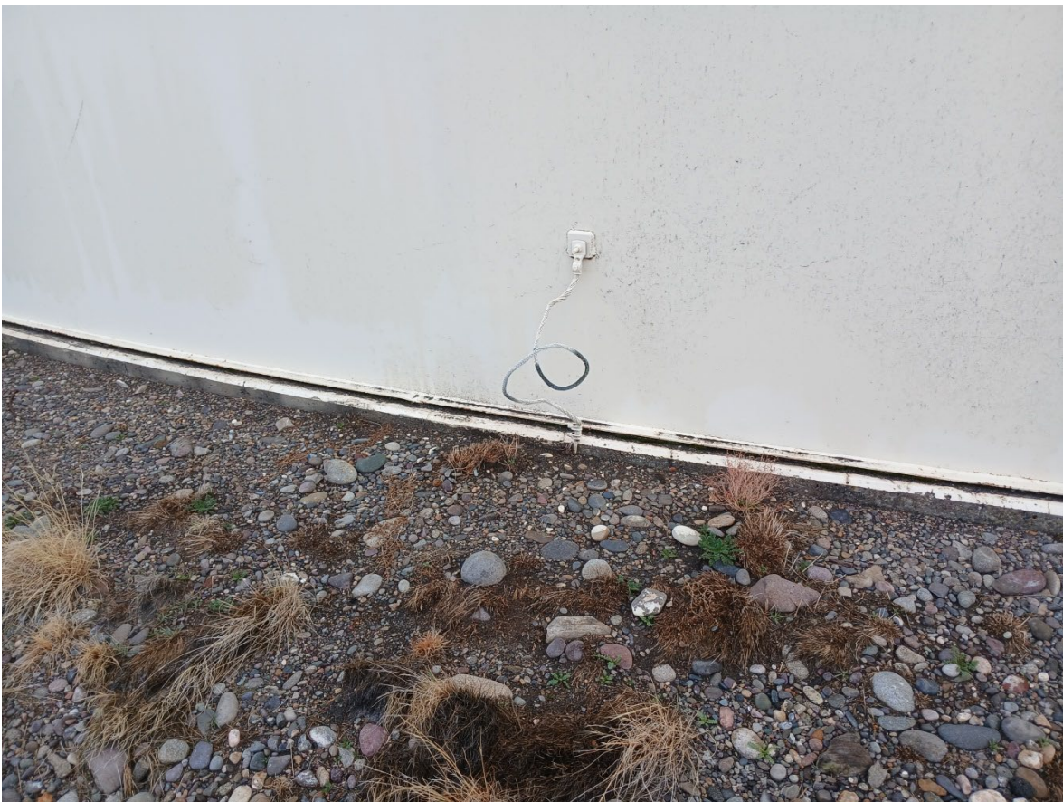
Photo 18. One (1) of two (2) grounding wires at bottom of tank
