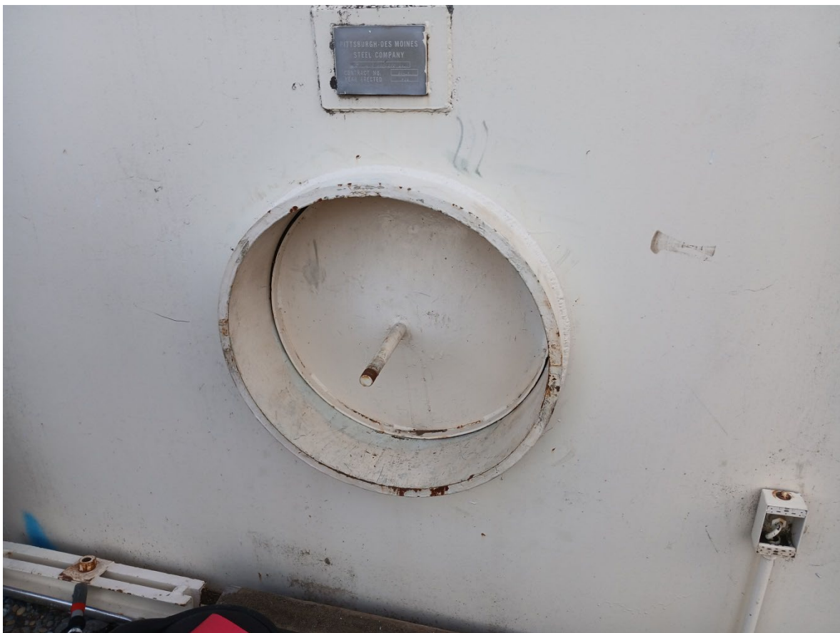
Photo 05. Exterior view of 24" shell manway
