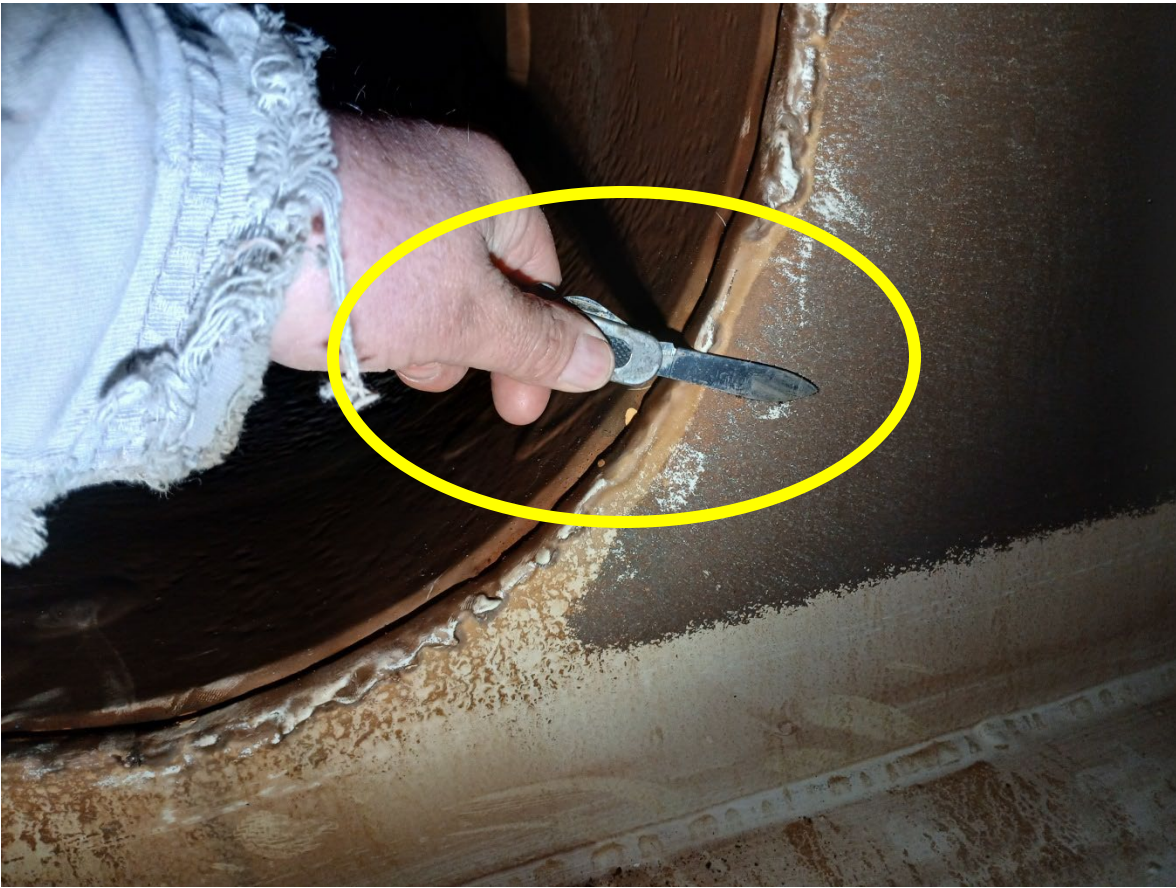
Photo 33. Air gap between shell outlet nozzle and shell
