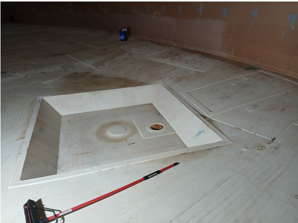
Photo 36. Sump and drain configuration
