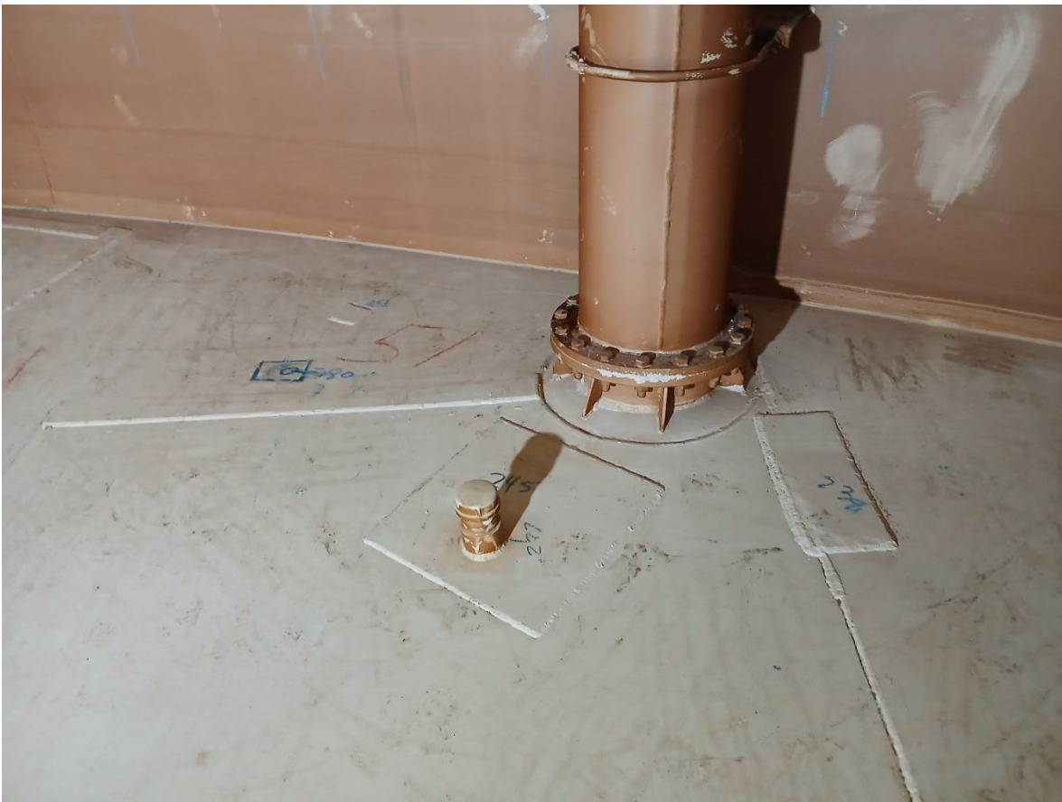
Photo 45. 16" overflow and patches on bottom
