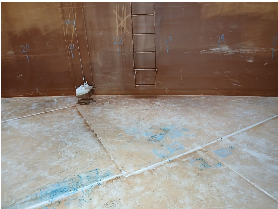
Photo 54. Internal ladder and level float configuration
