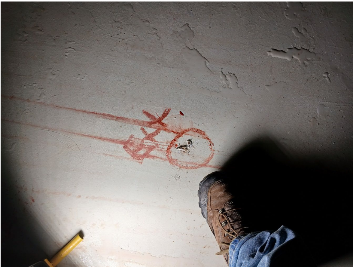
Photo 59. Example of extraneous weld on tank bottom plate
