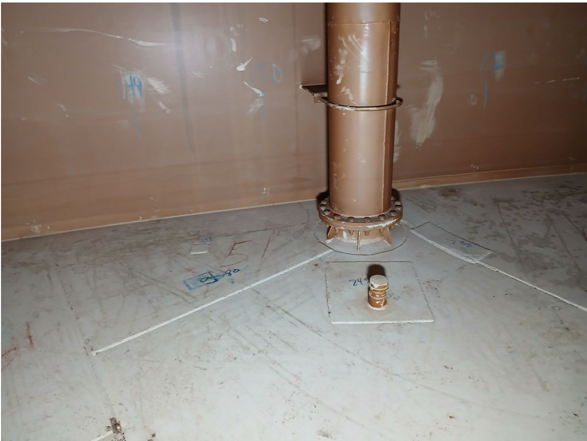
Photo 42. Patch plates around the sump and 16" overflow
