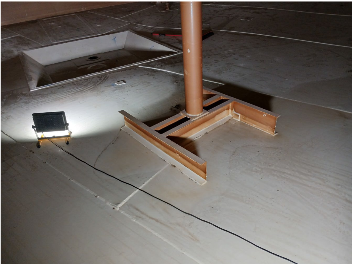
Photo 38. Sump and drain configuration, scattered small fillet welded patches on tank bottom
