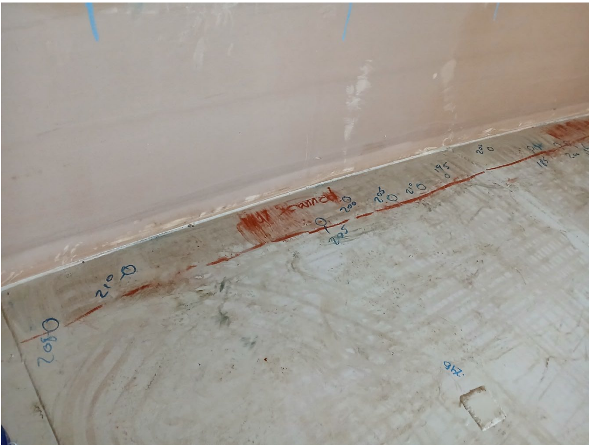
Photo 55. Example soil side corrosion / pitting at suspected edge of concrete ring wall
