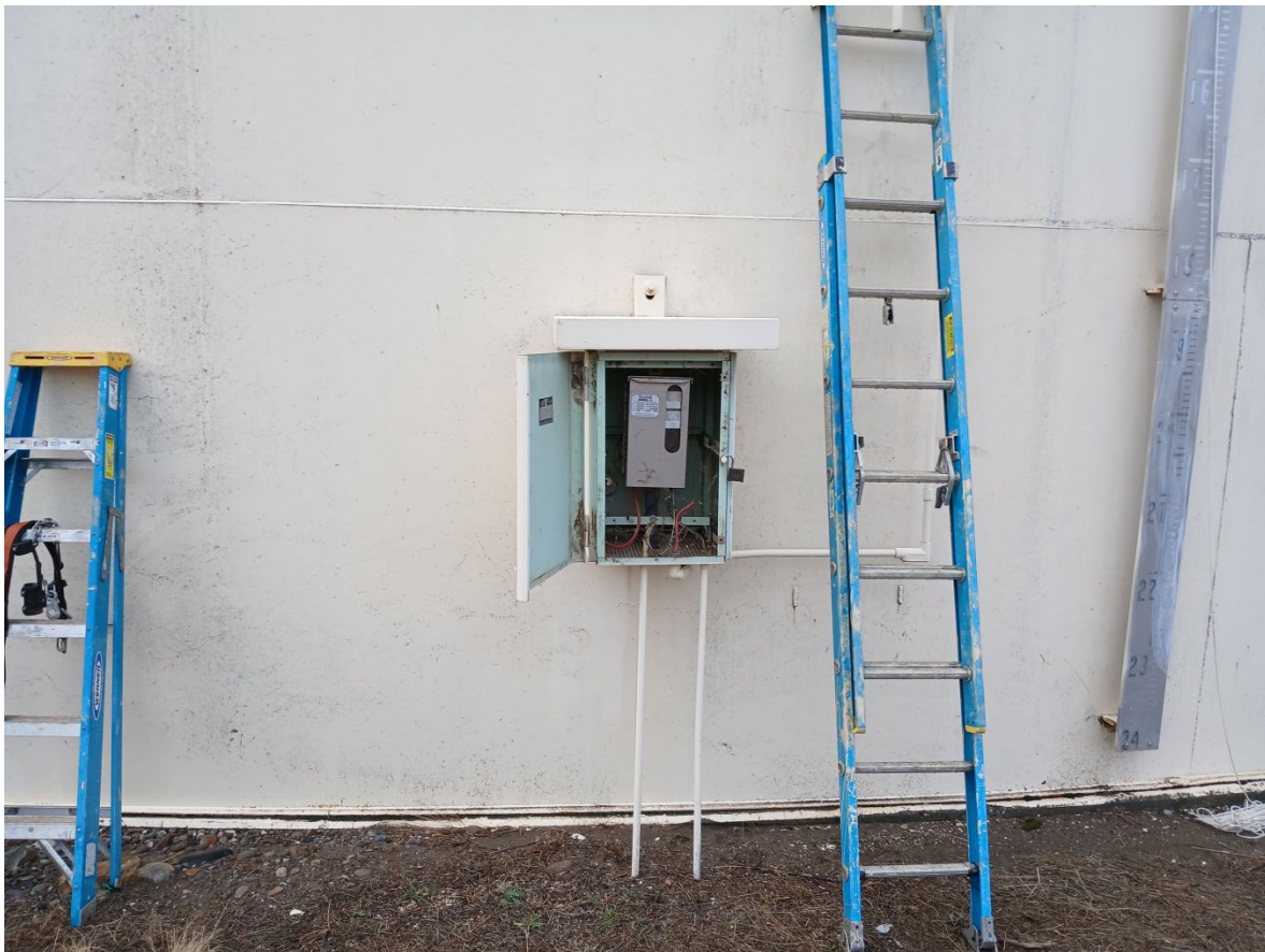
Photo 20. Cathodic protection rectifier for soil side of tank bottom
