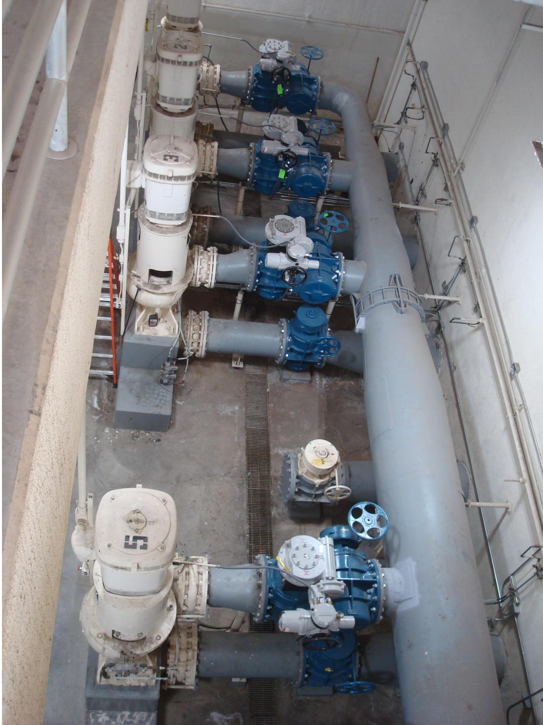
Photo #1: This photo shows the pump room with the intake and discharge pipe with gray paint on them. The pumps and pipes are in the basement of this building.
