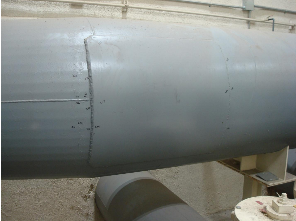
Photo #3: Another patch welded onto the steel pipe. The most recent patch made to the steel discharge pipe was completed in summer 2025.
