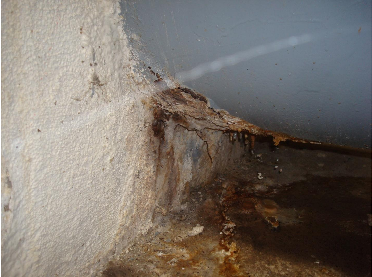
Photo #4: This photo shows the corrosion on the underside of one of the steel suction pipes at the concrete wall.
