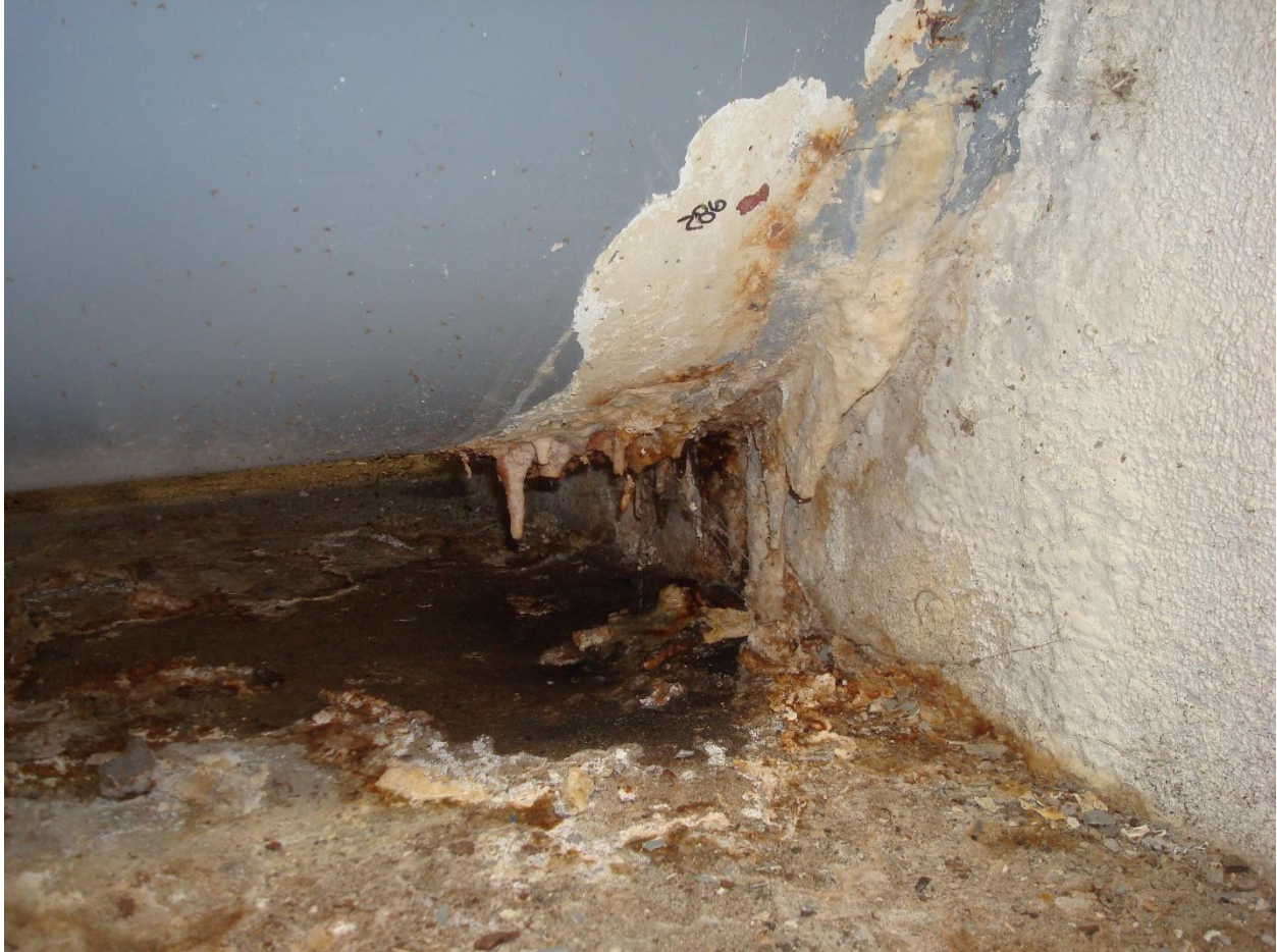
Photo #5: Another steel suction pipe showing signs of corrosion and seepage.
