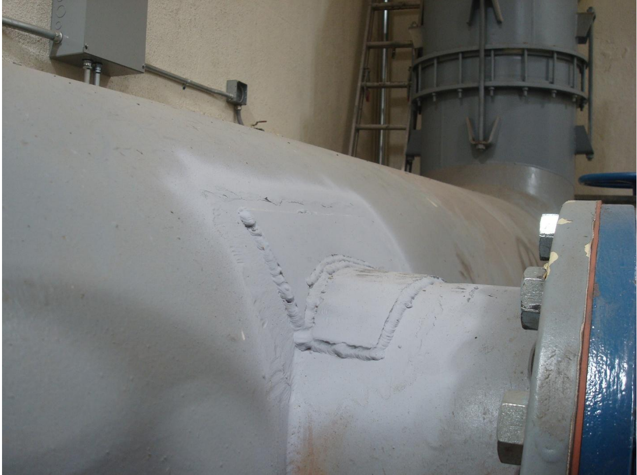
Photo #2: This picture shows a patch made to the steel discharge pipe.
