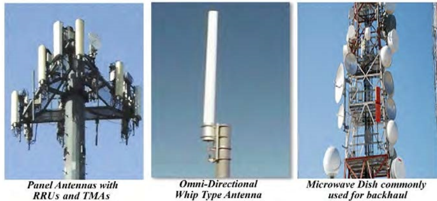
Figure 3: Examples of Panel, Directional and Microwave Antennas
