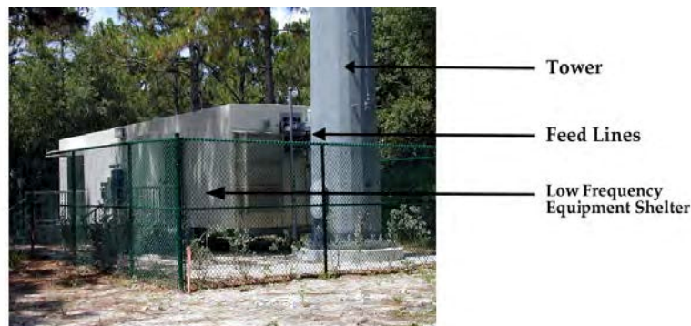
Figure 2: Example of Low Band Wireless Infrastructure Ground Equipment
