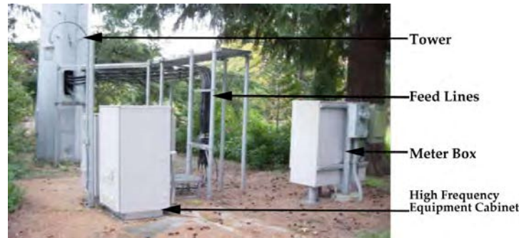
Figure 1: Example of High Band Wireless Infrastructure Ground Equipment
