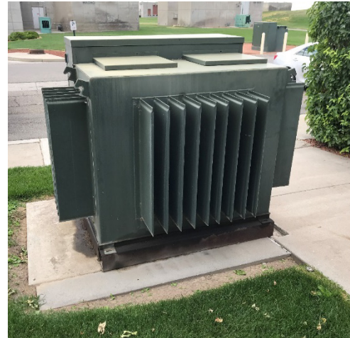
Figure 7.3 Administration Building Transformer
