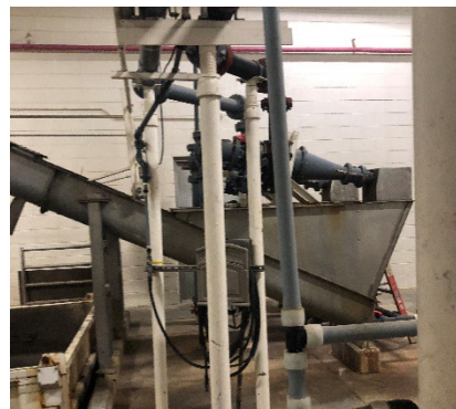
Grit washer compactor.
