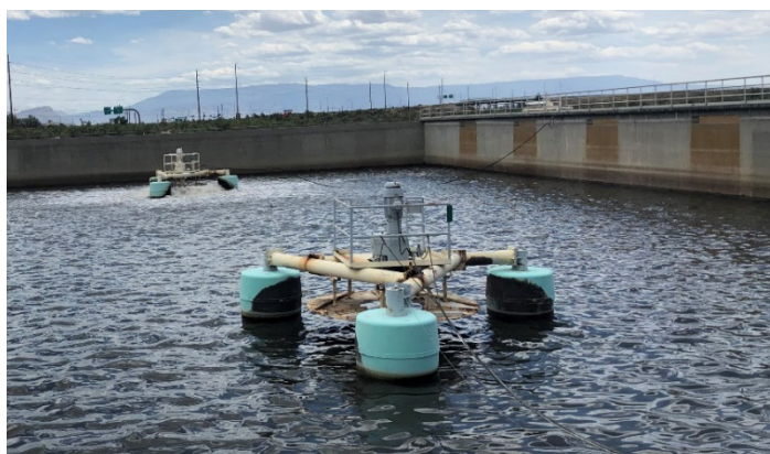
Figure 5.10 Floating Surface Aerators and FE Basin
