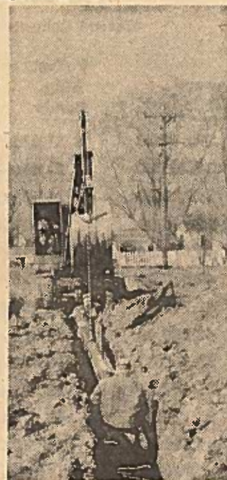
Annexations mean new water lines. A crew installs water mains in a part of the $60,000.00 Fruitvale project in 1960.
