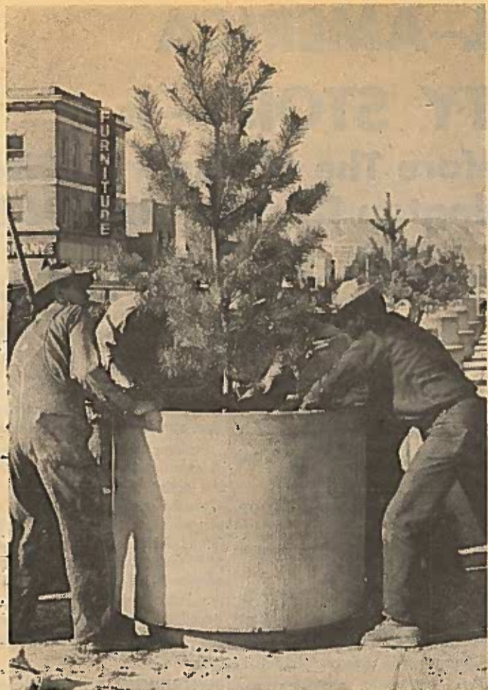
The first greenery in the new Shopping Park were the pines in the cement tubs. Each planter tub is equipped with its own sprinkling head and electrical outlet for decorative lighting. A special brilliant white masonry paint will finish the job.
