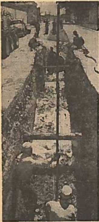
The new storm sewer is graduated up to a 3-foot diameter. The main trunk lies in Colorado Ave, and picks up drainage off Main via collector lines and gutters.
