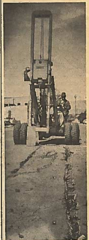
Opening the street surface in Colorado Ave. was the first step for the new storm sewer. Until 1962, the majority of the downtown area was not served by any storm sewer. The new sewer will allow regular flushing of the streets to keep the city center cleaner.
