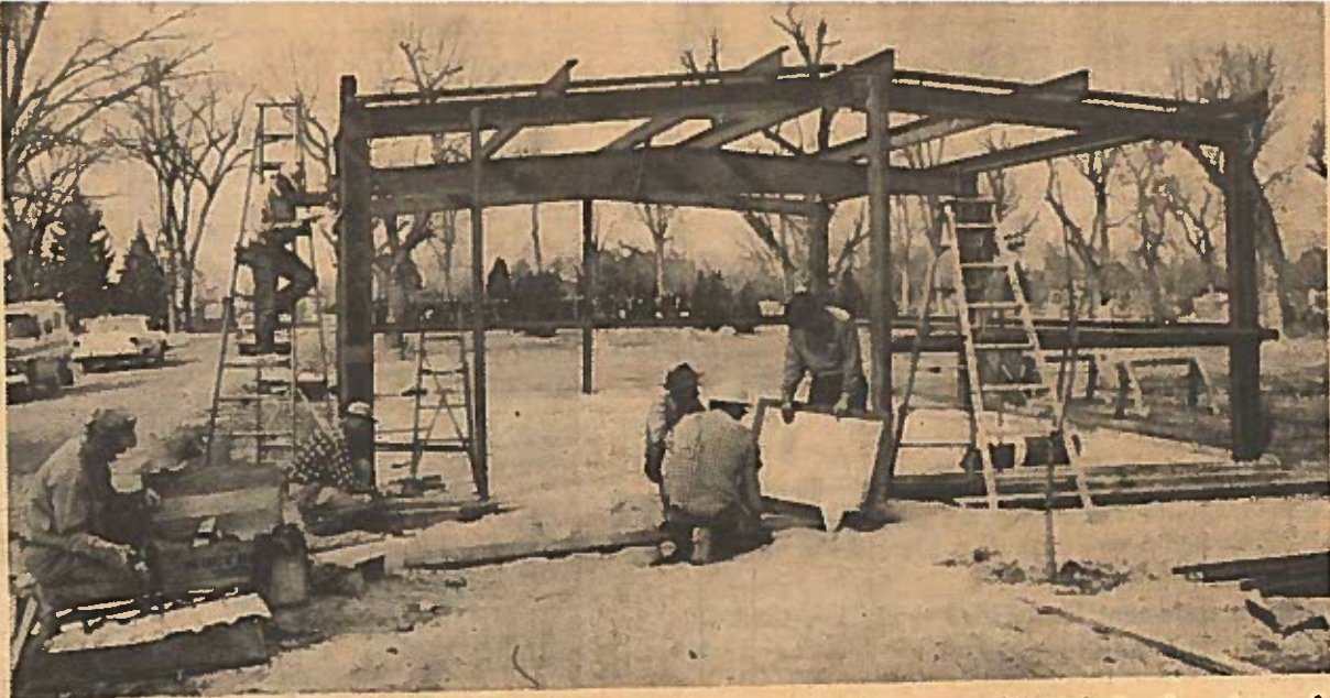
City Park and Cemetery crewmen assemble a new storage and work shop building for the extra work brought on by cemetery consolidation. More paved driveways and new entry arches the planned for 1966.
