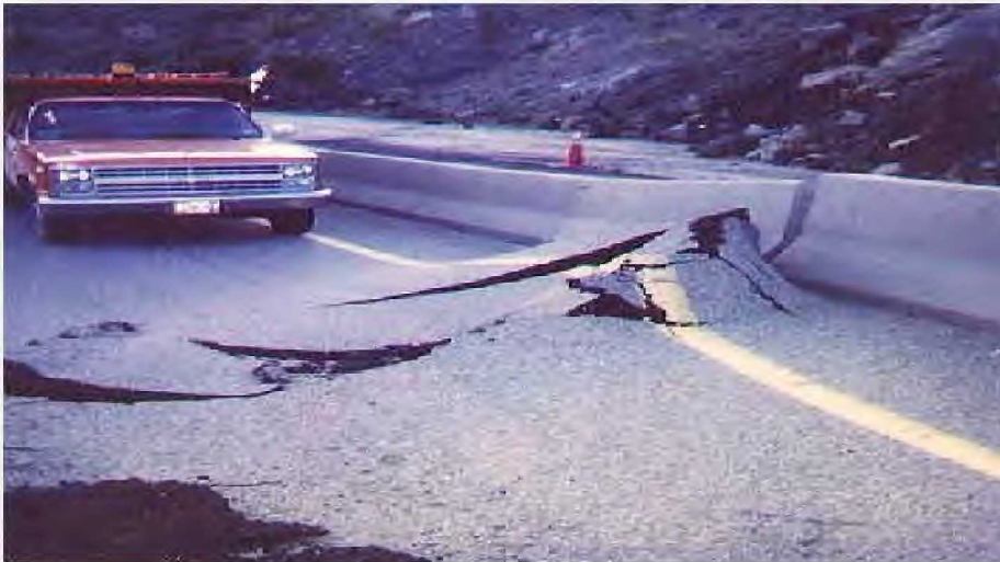
FIGURE 12 PHOTO OF DeBEQUE CANYON SLIDE AREA- INTERSTATE 70
