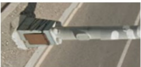
Electrical tape holding parts on to pole base
