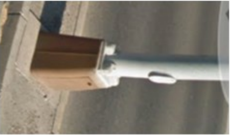
Inconsistent pole bases
