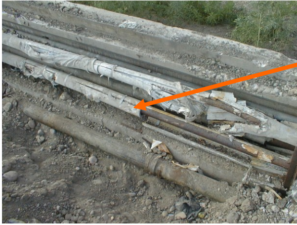
Asbestos wrapped steam line
