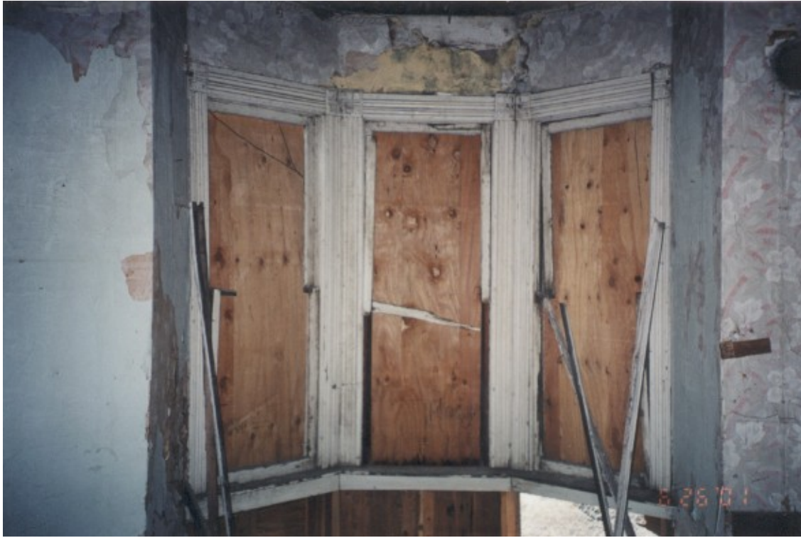
27. Interior side of boarded up bay window located on the east wall.
