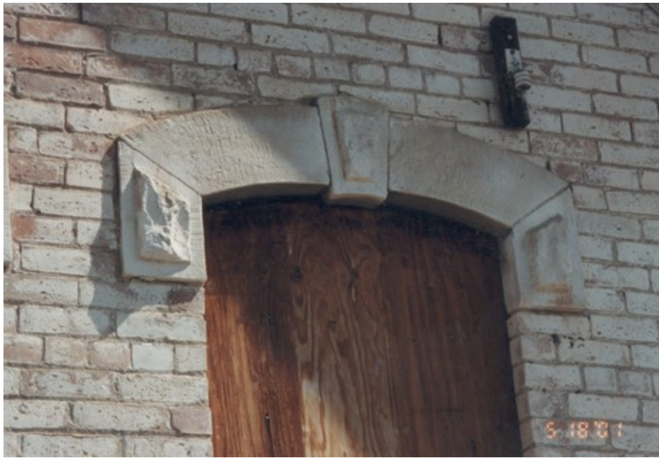
10. Close up of window hood on south face and porcelain electrical insulator.
