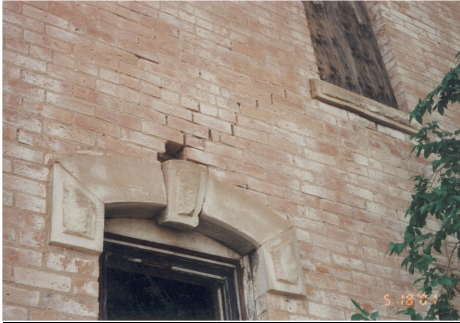
11. Close up of loose hood keystone and brick damage on west face of two story portion.
