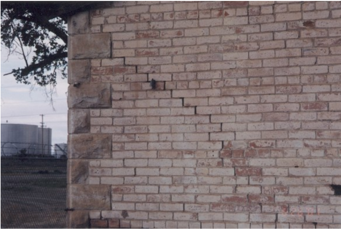
16. Southwest corner - Crack is result of possible foundation movement. This is just around the corner from the brick damage on the west side of the one story portion.
