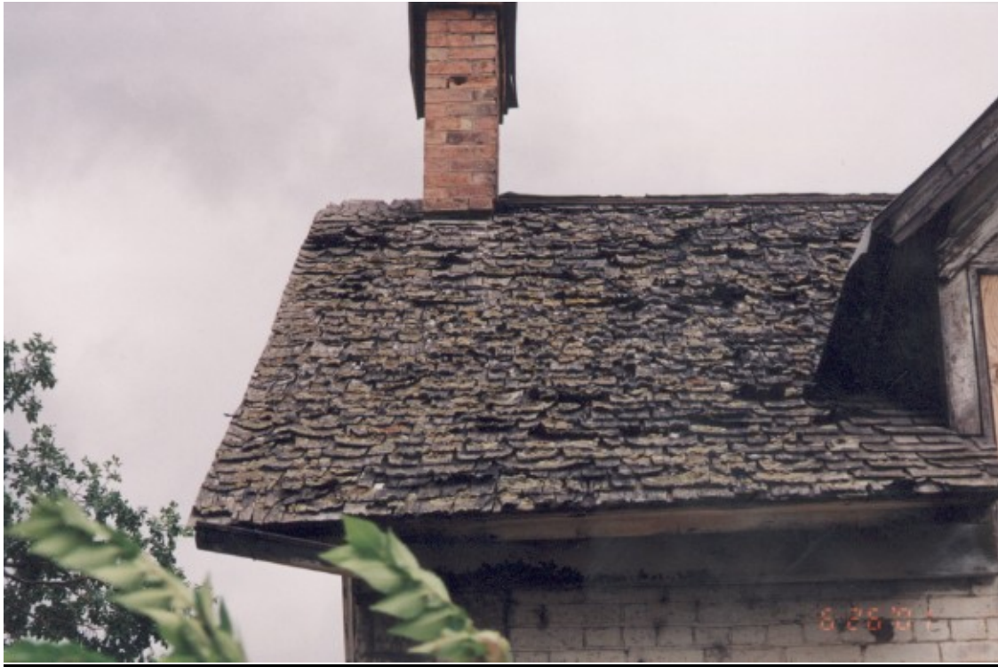
21. Northeast corner of two story portion with cupped and curled wood shingles still in place and chimney with a wood cap to temporarily protect the top curb.
