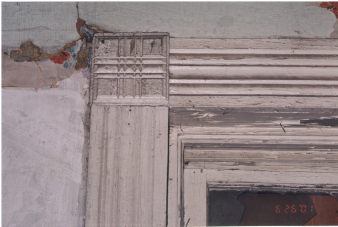
26. Close up of the typical interior door and window trim. This is a window on the south wall of the one story portion.
