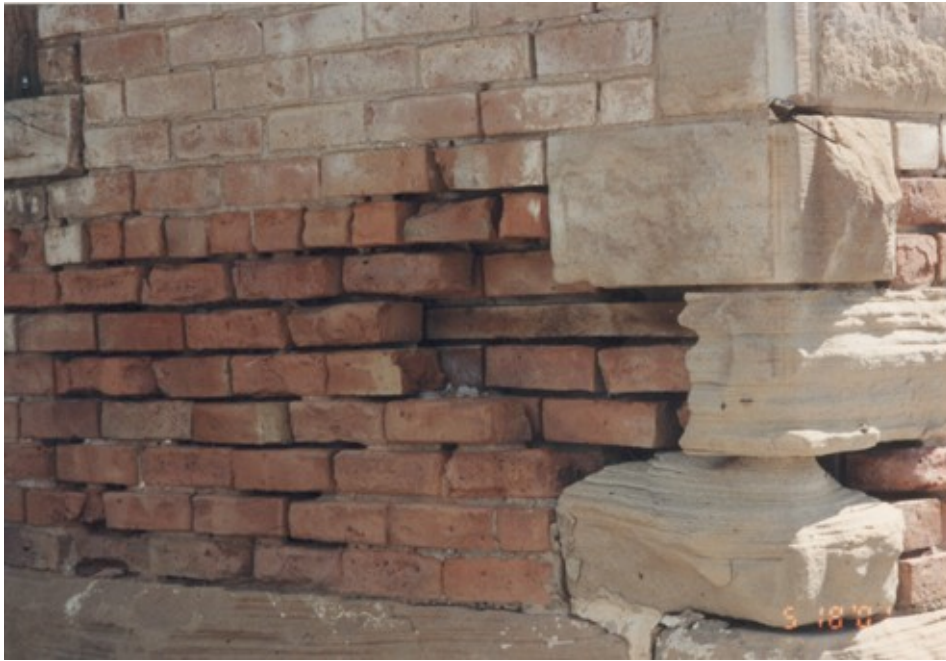
8. Close up of damage to brick and sandstone quoins at southwest corner of the one story portion.
