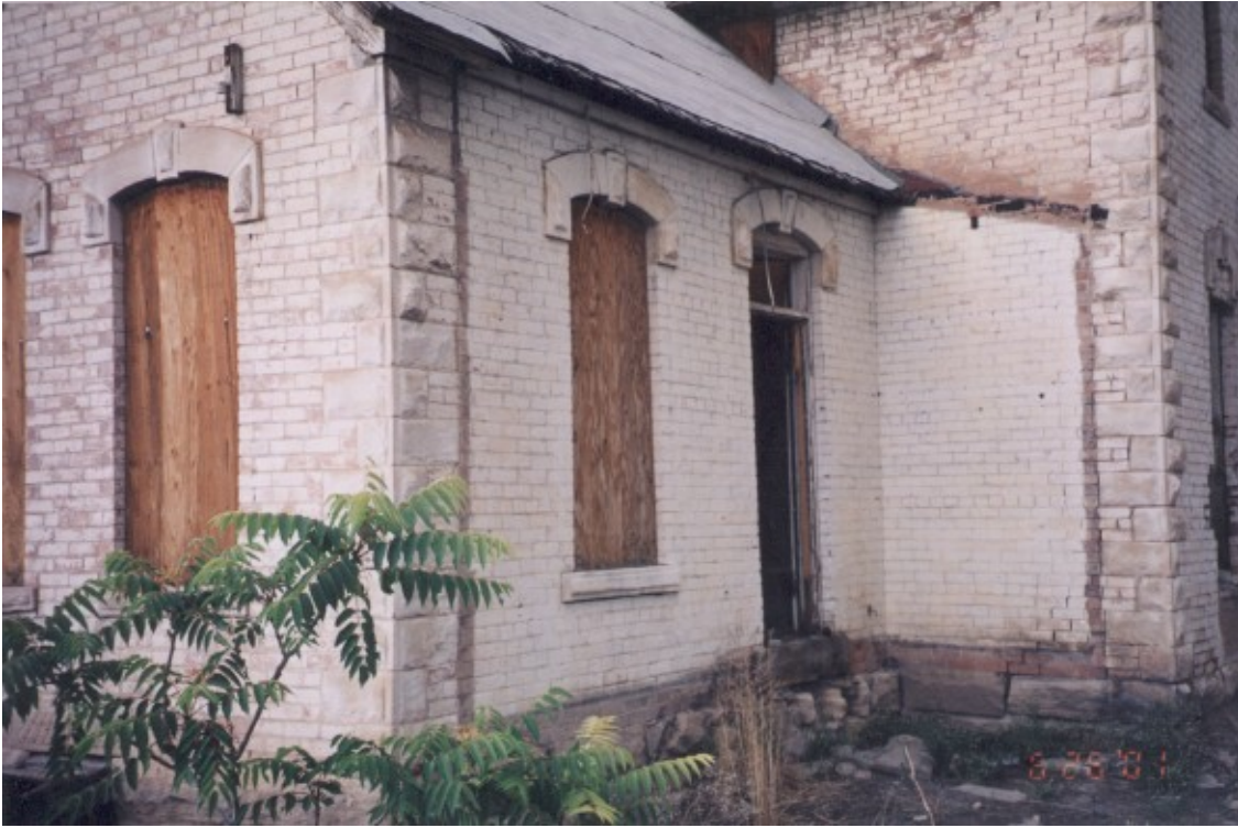
15. East entrance to the one story portion. The outline of a once present covered porch is visible in the painted brick.
