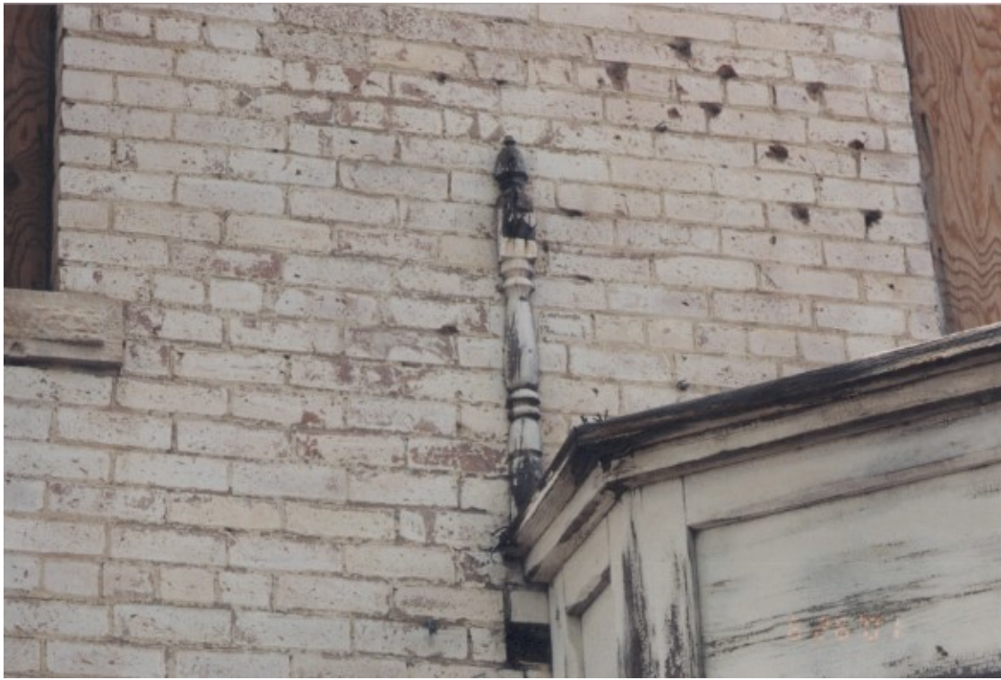
18. Guardrail post at deck on top of east side bay window. A few of the guardrail pieces have been salvaged and are stored within the house on the second level.
