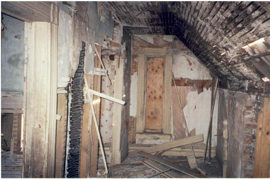
30. Upstairs hallway looking west to east shows some of the recent damage done by vandals.
