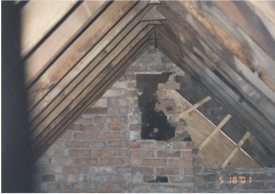
23. Roof rafters over the one story portion with bricks missing from the gable end and the chimney
