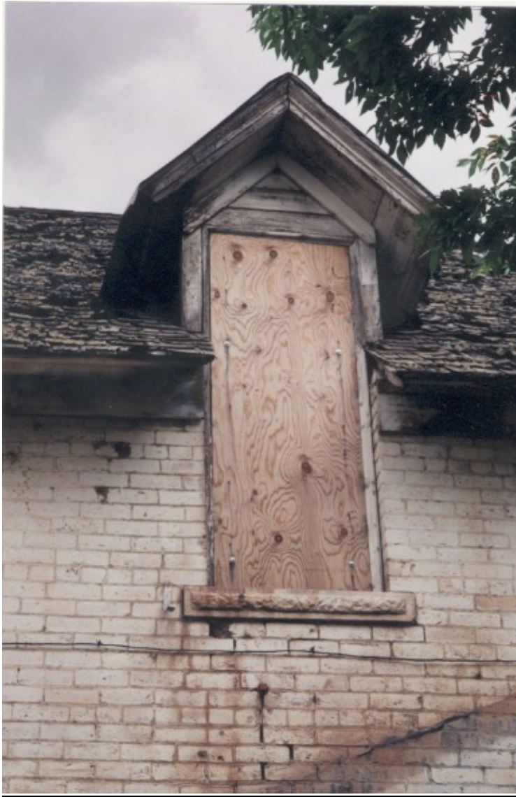
20. Boarded up bedroom gabled dormer at north side of two story with view of wood shingles.
