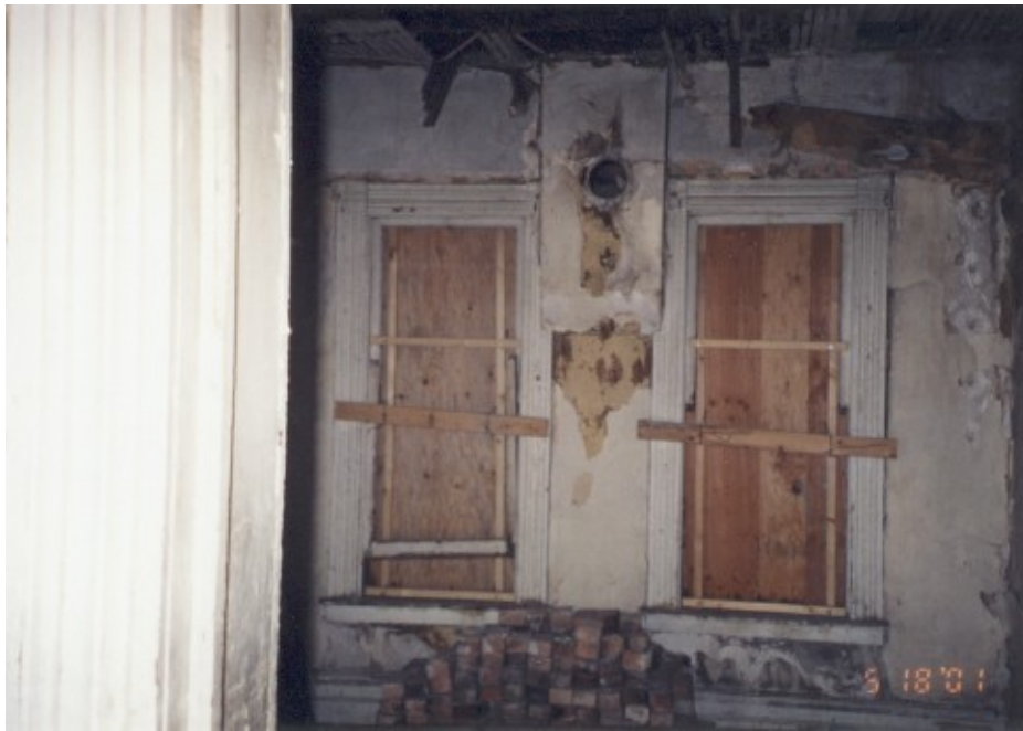
28. Interior side of windows at the south wall of the one story portion with wood stove chimney and a pile of bricks that came from gable end above windows.
