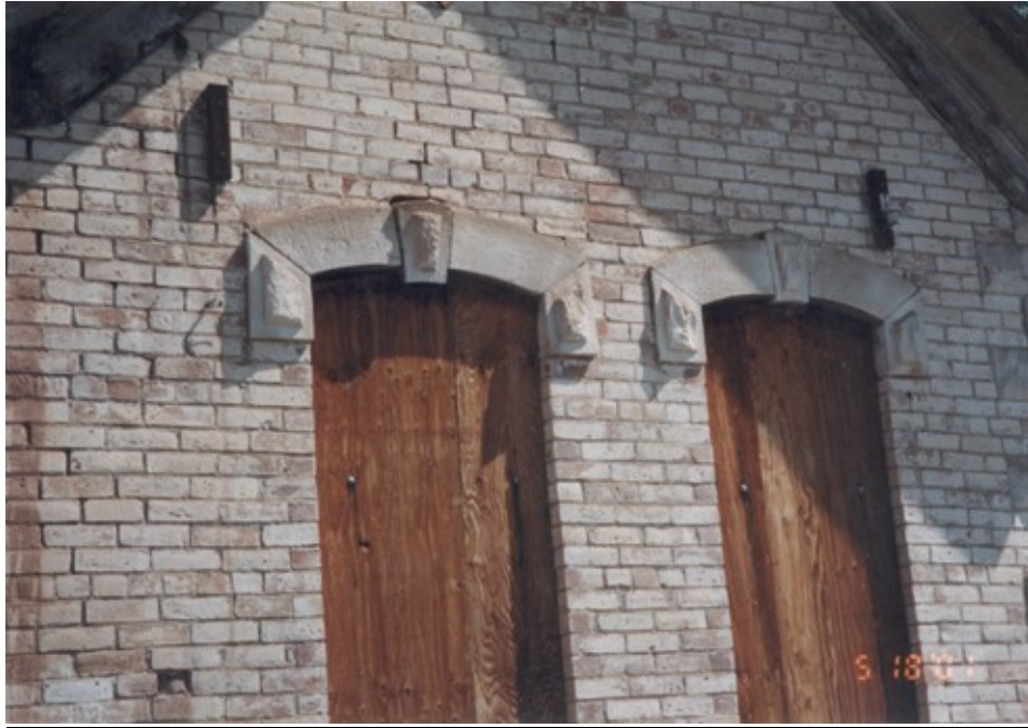
9. Typical window hoods at the south face of the single story portion. Also visible are two wooden mounts and one porcelain insulator from electrical wiring to south west room of the one story portion.
