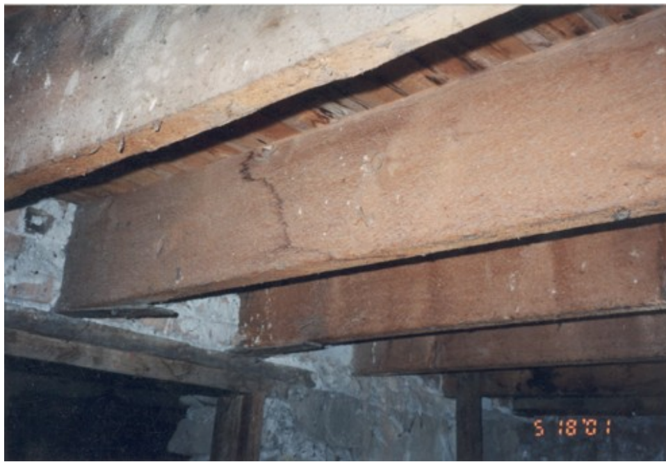
22. Bottom side of floor joist inside the basement under the southeast corner of the one story portion
