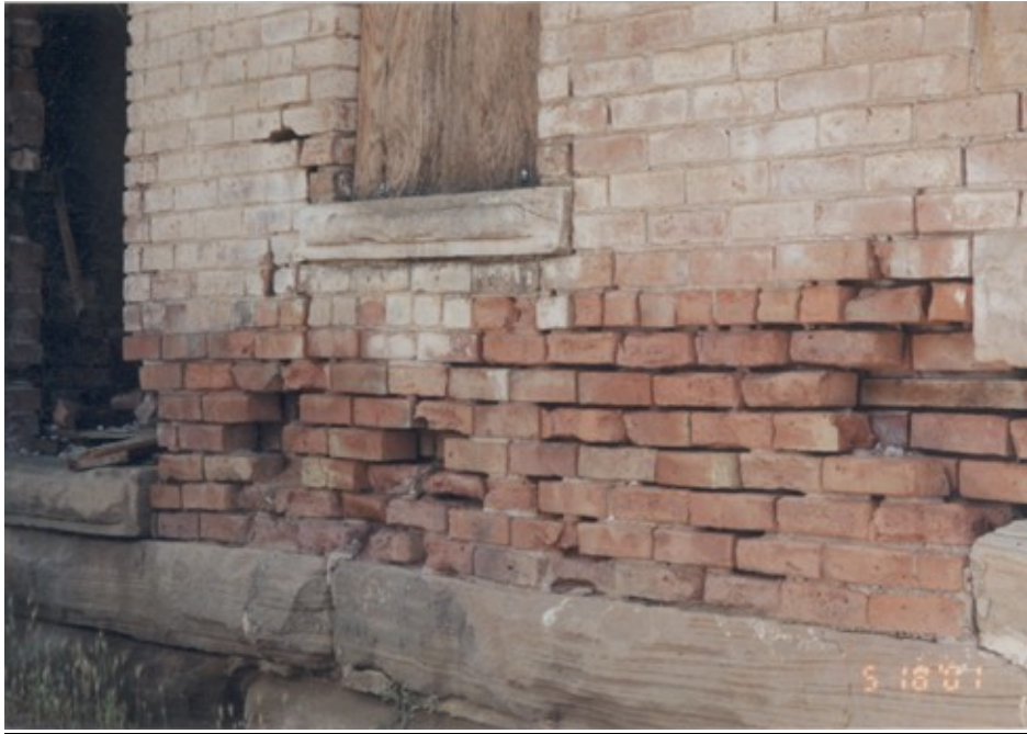
7. Deterioration due to water saturation at west side of the one story portion. Damage probable cause due to roof over this room gone prior to stabilization work by the City
