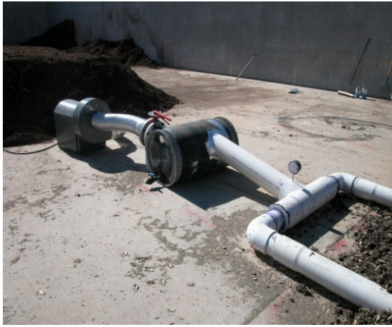
Aeration Blower/Drip Trap
