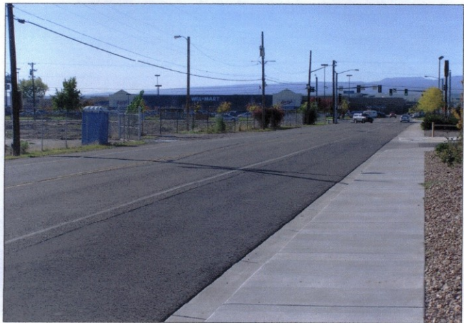
28 3/4 Road Project: Construct sidewalk, curb and gutter and widening along the east side of the street adjacent to The Plaza on North Avenue.
