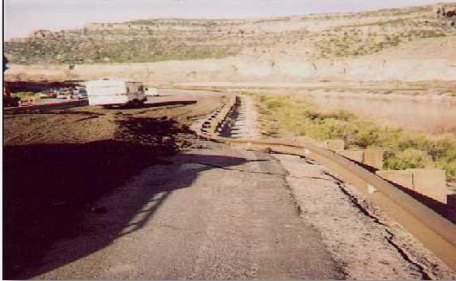
FIGURE 11 PHOTO OF DeBEQUE CANYON SLIDE AREA- INTERSTATE 70
