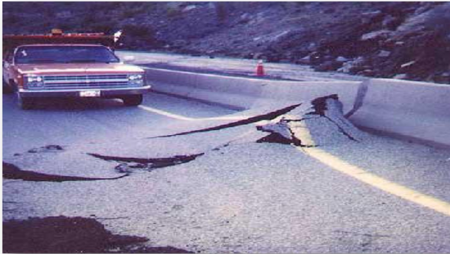
FIGURE 12 PHOTO OF DeBEQUE CANYON SLIDE AREA- INTERSTATE 70
